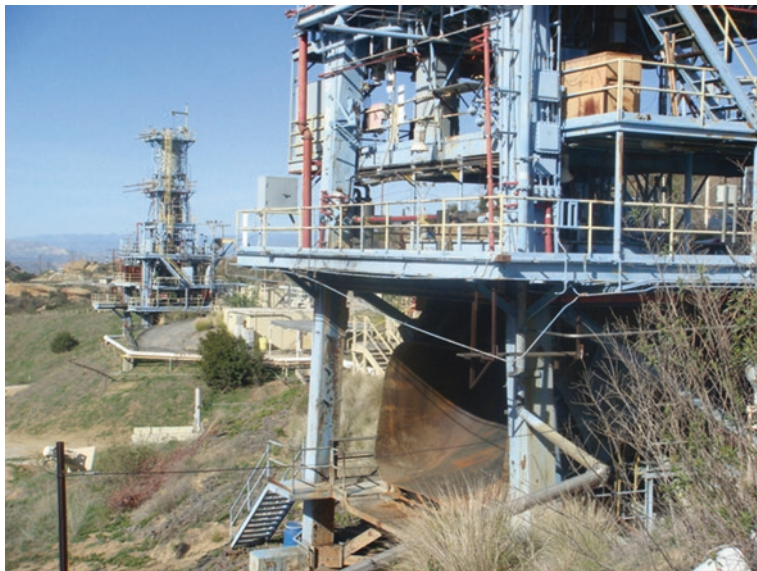
Fig. 7.6 Vertical Test Stand One, Santa Susana Field Laboratory, California. The Santa Susana Field Laboratory is a complex of industrial research and development facilities located on a 2,668 acre portion of the Southern California Simi Hills in Simi Valley, California, used mainly for the testing and development of liquid-propellant rocket engines for the United States space program from 1949 to 2006 (photo by the author)
