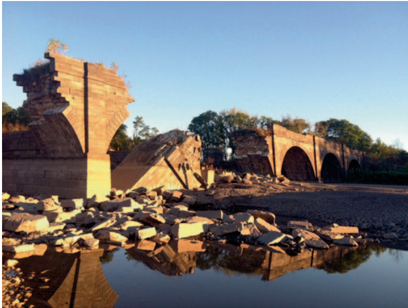
Fig. 3.3 The Schoharie Creek Aqueduct, Fort Hunter, NY, a portion of the historic Erie Canal, is a National Historic Landmark. Constructed from 1838 to 1841, the Army Corps of Engineers demolished six arches in the
