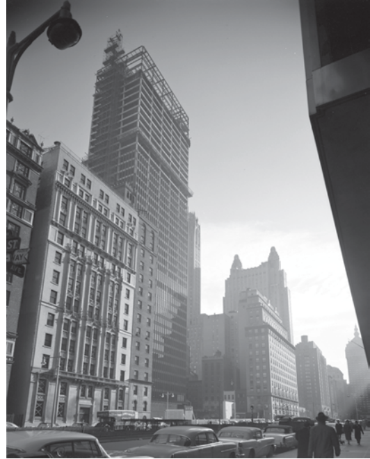
Fig. 6.9 The Seagram Building on Park Avenue, here seen under construction in January, 1957, was one of the first International Style skyscraper commercial structures to feature glass walls, in marked contrast to the properties around it. (Gottsocho Shleisner, Inc. photograph, Library of Congress)
