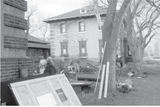
Fig. 6.10 The stabilization of the hospital buildings on Ellis Island involved securing the buildings and allowing sufficient light and ventilation in a very humid location. The documentation of the volunteer labor of Cornell students and alumni and other groups allowed the National Park Service to argue more effectively for financial support to continue to the work. (Author's photograph)
