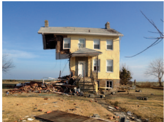
Fig. 6.25 Hurricane Sandy struck New Jersey and New York coastlines with an enormous amount of wind and water. Here, the typical result, in Union Beach Borough, Monmouth County NJ. (Courtesy of the New Jersey State Historic Preservation Office, 2012)
