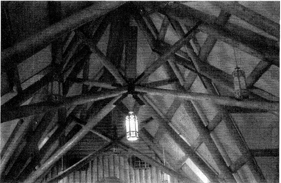
Fig. 10-2. Interior of church building with scissors trusses formed from peeled logs. (Photograph by authors.)
