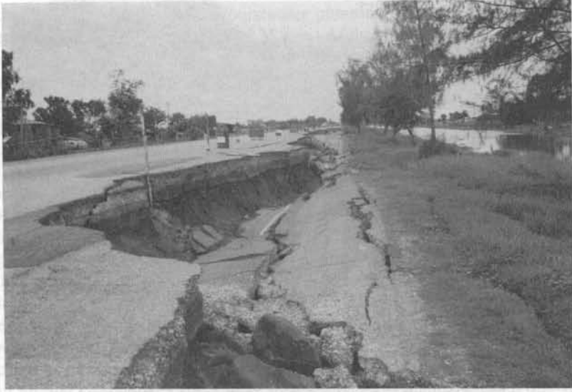
Fig. 1.1 Embankment Failures along an Irrigation Canal
