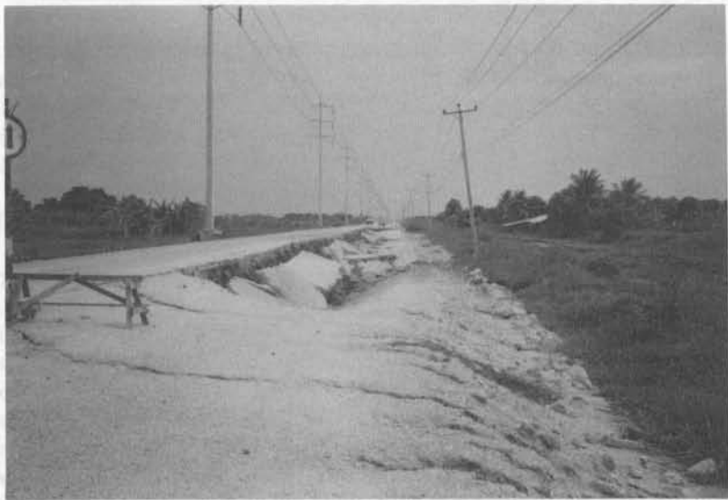
Fig. 1.2 Typical Failure of Road Embankment on Soft Ground
