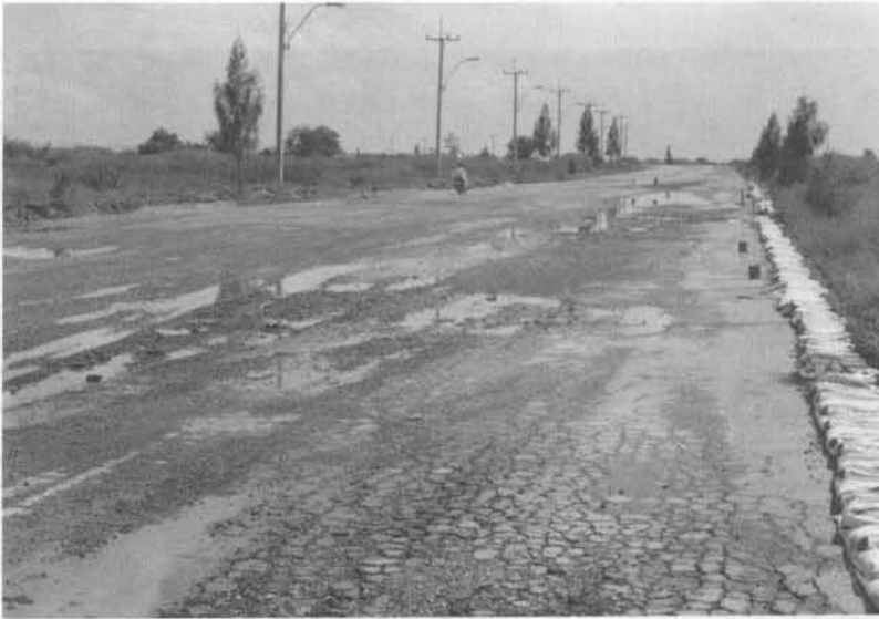
Fig. 1.4 Pavement Failures due to the Sinking of Road Embankment
