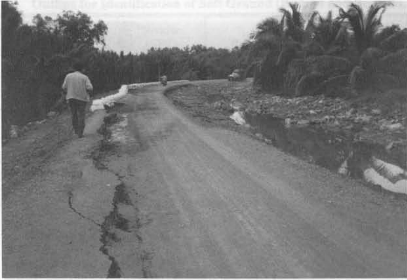
Fig. 1.3 Road Embankment Failure on Soft Ground
