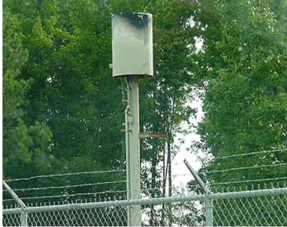
A methane "flare" is used for burning landfill gas.
