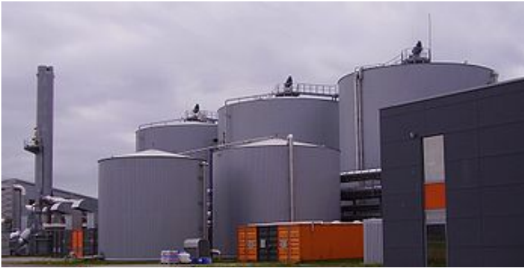
Fig. 6.14 Anaerobic digestion and air processing components of Lübeck mechanical biological treatment plant in Germany (From Wikipedia, Free encyclopedia)
