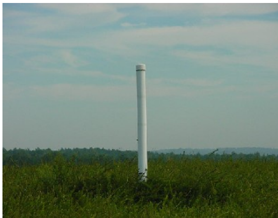
A methane collection pipe helps capture the hazardous gas.
