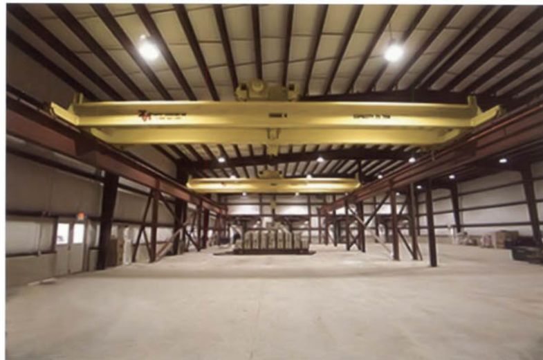
Crane not self-supporting for vertical and lateral loads
