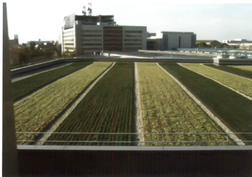
Weight of landscaping and other materials at roof garden is to be included in effective seismic weight.
