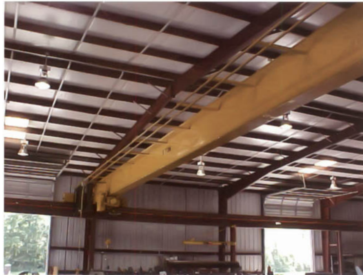
Crane self-supporting for vertical loads but not self-supporting for lateral loads
