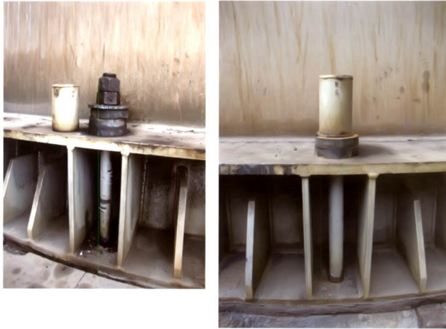
Anchors in concrete used for nonbuilding structure anchorage in Chile Courtesy of J. Silva, ASCE/SEI 2010 Chile Earthquake Reconnaissance Team
