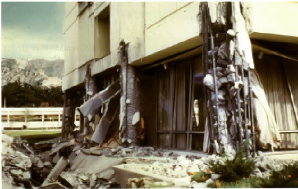
Olive View Memorial Hospital following the San Fernando earthquake of 1971. The columns supporting the discontinued shear walls are required by ASCE 7-10 to be designed for seismic load effects including overstrength factor.
