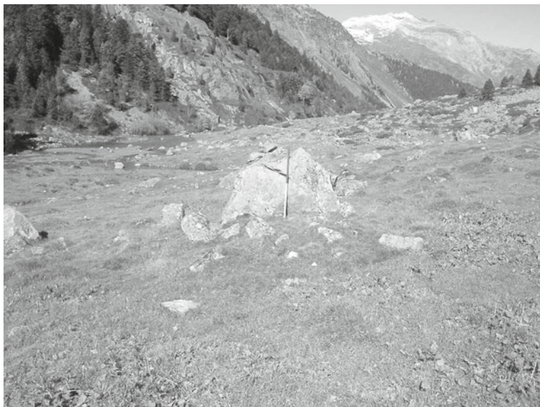
Fig. 5.17 Foundations of damaged hut resemble structure type 1b
