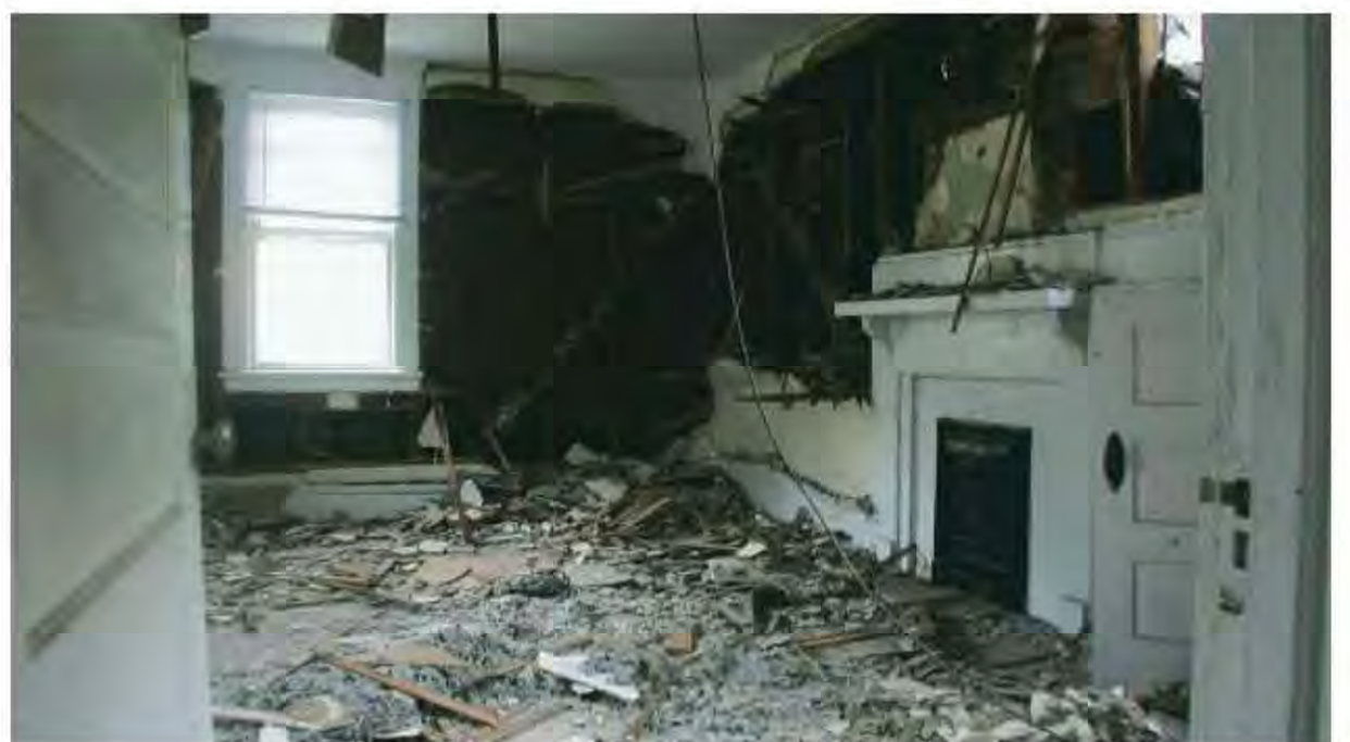
Fig. 6.32: A house in the process of a gut job — a messy, hazardous and major waste- producing procedure.
