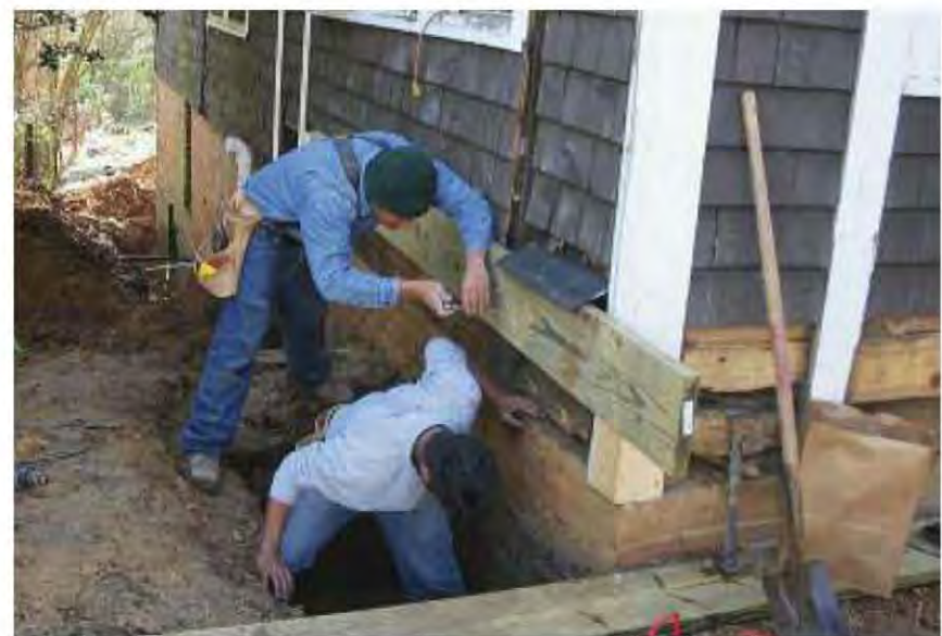
Fig. 9.25-26: Sill repair starts with jacking the home, done here by simultaneously lifting the joists from under the home and lifting the studs from the outside. The rotted sill was removed and replaced by a built-up 2x girder.
