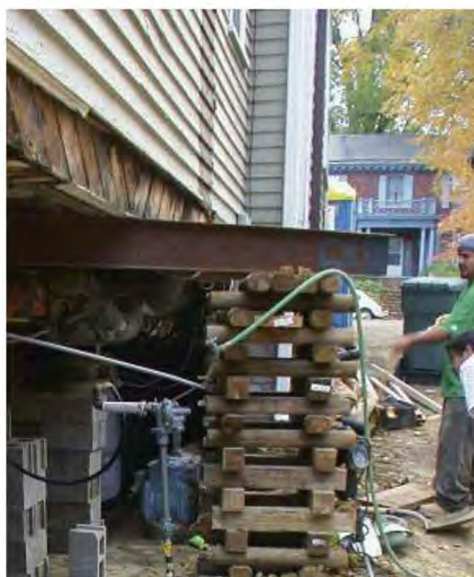
Fig. 9.14-15: Left, the house is held by steel beams while the foundation is reconstructed; a pier and curtain wall foundation is replaced by a more stable 12-inch-thick CMU block and brick veneer wall. Right, house jacks, typically 20-ton, do the heavy lifting.
