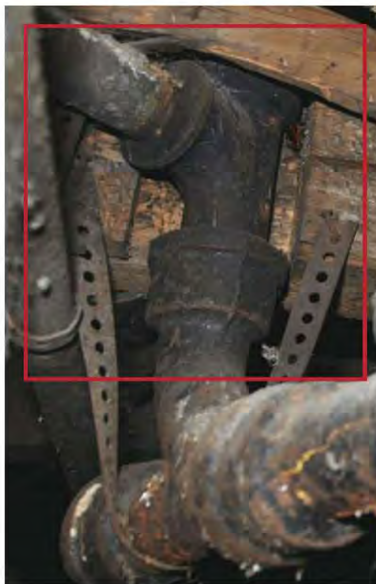
Fig. 12.7: A plumber installed a waste line directly through a primary structural girder, compromising the structural integrity of half the house. A heavy clawfoot tub, weighing nearly a ton when filled, lay directly above. Inadequate support for such weight can lead to serious structural failure.
