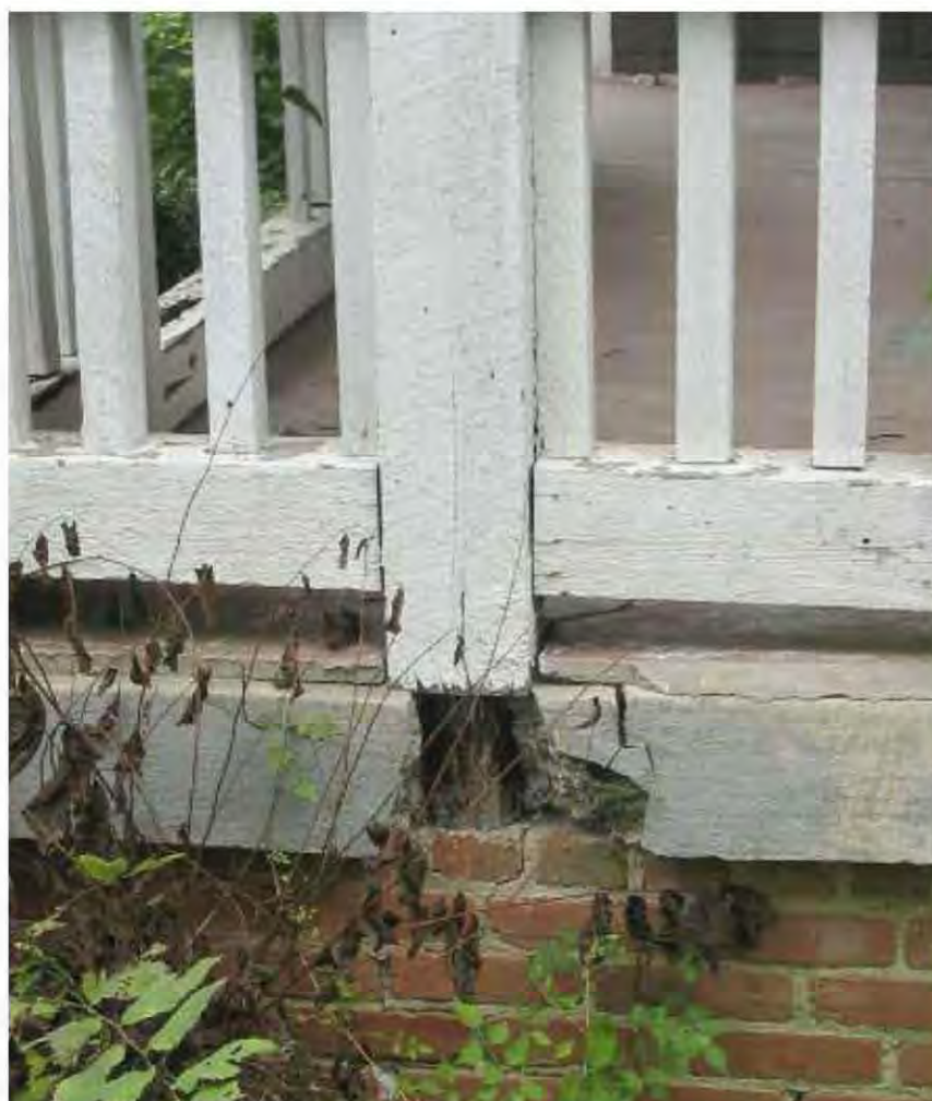
Fig. 8.29-30: Left, the porch structure on this transitional Craftsman had failed because the supporting 6x6 posts were wicking water and causing decay. Right, the 6x6 members were reconstructed and set on a small metal base that allows water to drain away underneath.
