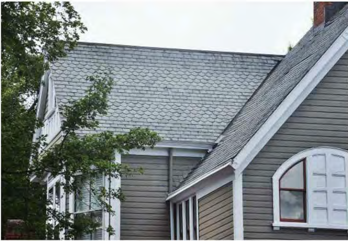
Fig. 8.18: A 130-year-old home, where the locals swear the slate roof is original. High pitches shed water and snow better, making materials last longer.
