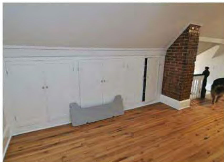
Fig. 7.5-6: An attic is converted to work space. Structural beams are painted to give a more finished look. Knee walls are great for built-in storage.
