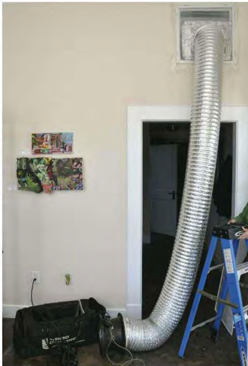
Fig. 13.13-15: A duct blaster being performed: a high-powered fan is hooked to the return, and all supply ducts sealed. The engineer will measure and identify leakage.
