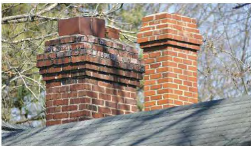
Fig. 8.25-26: Chimney caps vary from non-existent to simple to ornate. Chimney detailing, such as brick corbelling, is commonly overlooked in a large project. Masonry caps are particularly nice and worthy of rehabilitation. Metal caps are the modern norm, fabricated with common materials. Some feature bird screening.
