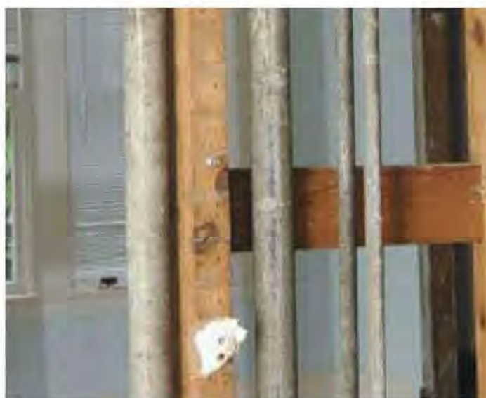
Fig. 12.6: Lead piping — a rare but serious concern.
