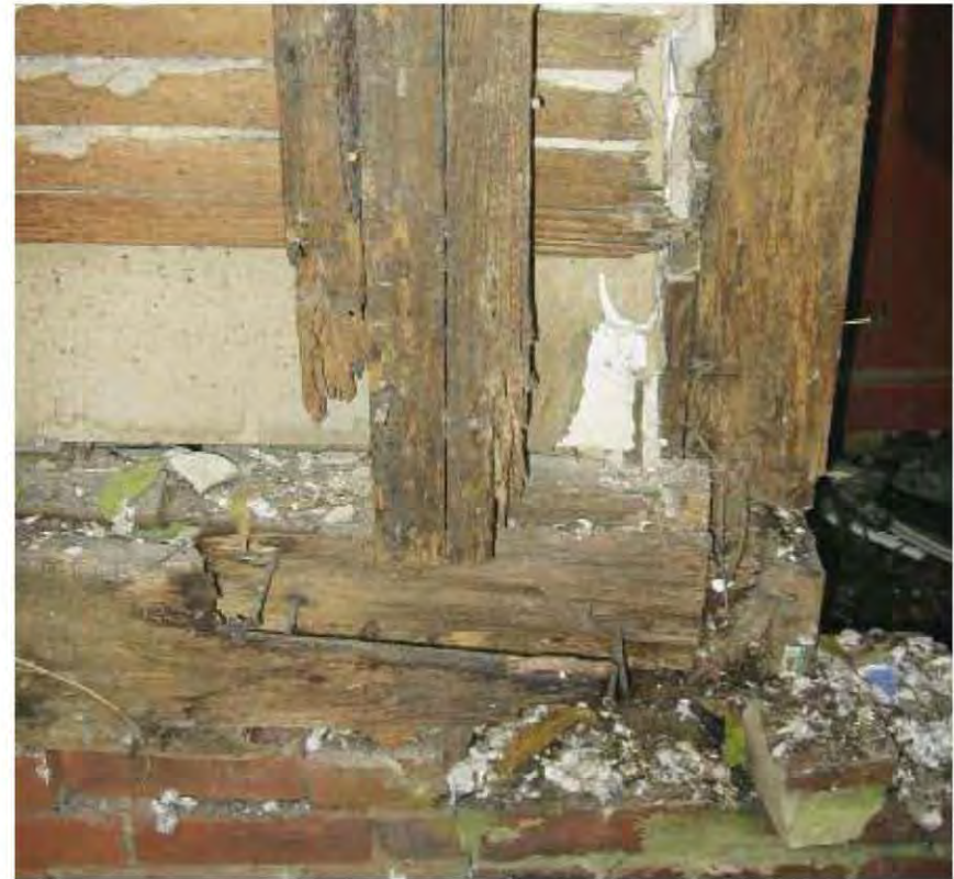
Fig. 9-20: A deteriorated stud. Sometimes partial sistering (called fish plating) can correct this problem. Other times an entirely new stud is warranted.
