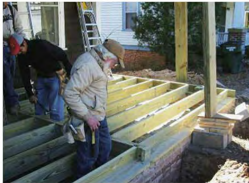
Fig. 8.31: Since porch flooring must allow for drainage the length of the board, and framing must run perpendicular to the flooring, porch framing requires installation of a mid-span girder.
