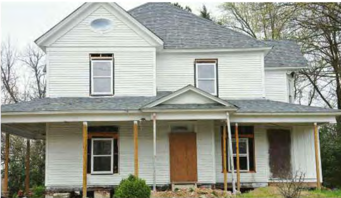
Fig. 11.9-11: Vinyl replacement would have been bad enough, but these replacements also don't match the size of the windows they're replacing. Left and center, new windows are half the size of the originals. Right, a vainly fake-muntin arched transom window, typical of modern McMansions, is installed on the second floor. Often in these cases, the cheapest available window is bought prior to sizing, then the opening is framed to the smaller unit. It often ends up costing more than rehabbing or buying a window of the proper size.
