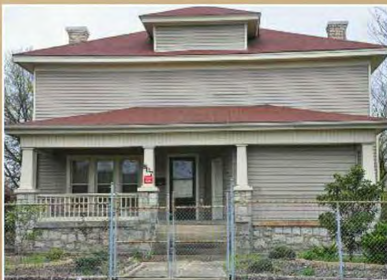
Fig. 8.2-3: A botched vinyl siding installation covers up all but one of the home's windows.
