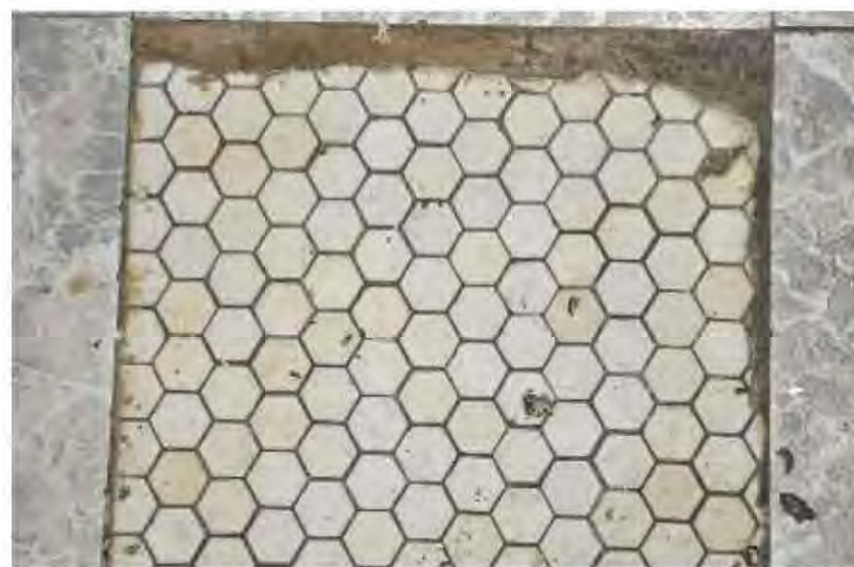
Fig 4.26: Original hexagonal tile covered by vinyl squares, a prime opportunity for restoration.
