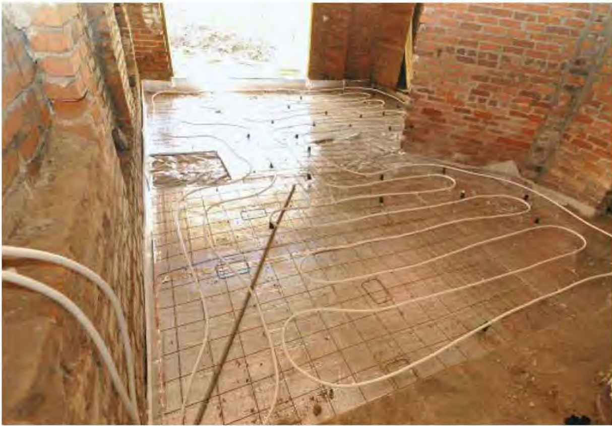
Fig. 13.11: A myriad of other systems offer options for any situation. Like all systems, careful attention must be paid to preservation principles. A radiant floor may be the most efficient option but is inappropriate if one has to tear up original wood floors to install such a system. Additionally, the average HVAC company will know about only some of these options, so pursuing them may require consulting a green building expert.
