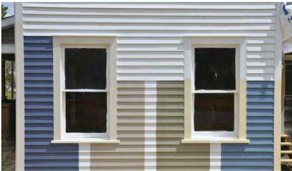
Fig. 8.34: A paint mock-up shows the client or designer different colors. Paint looks different in interior and exterior light, on wood as opposed to paper and in morning and afternoon light. All these are good reasons to do a test swatch on the building wall prior to choosing final colors.
