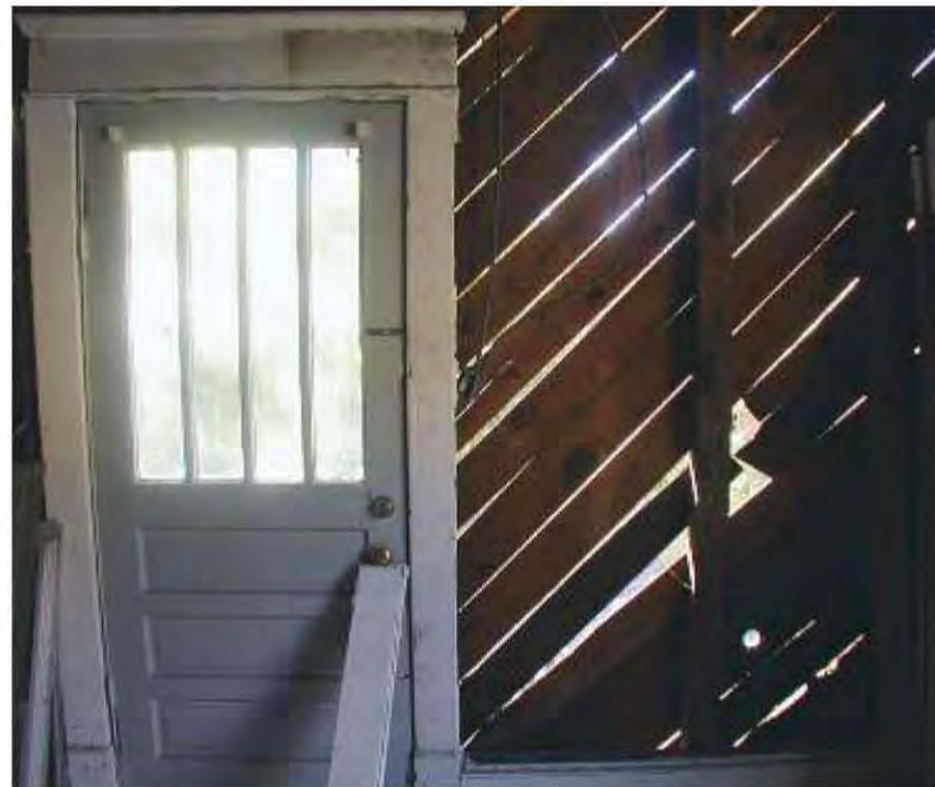
Fig. 9.18-19: Top, diagonal sheathing gave balloon frames greater sheer strength. Bottom, a Victorian has no sheathing, making it less structurally stable.
