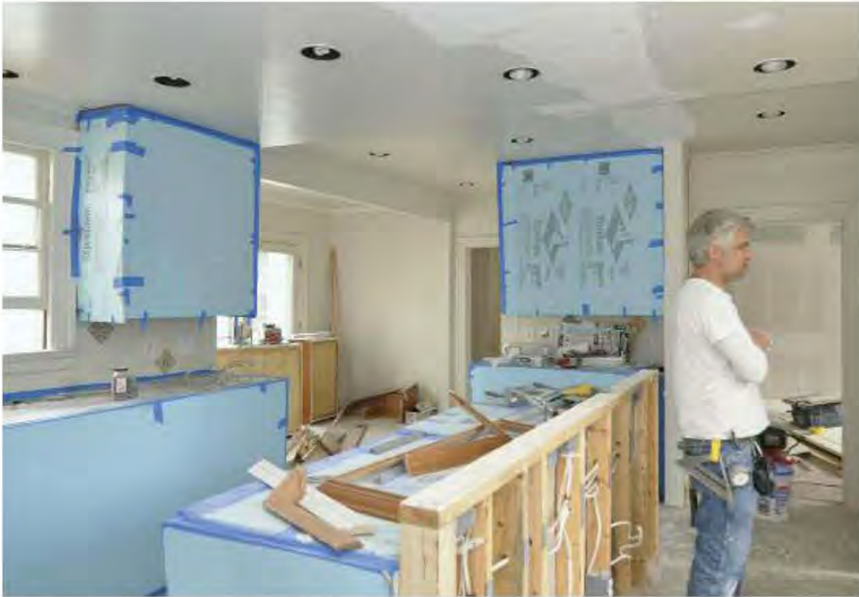
Fig. 5.32: Cabinets are temporarily protected from construction with foamboard (which can then be reused as insulation).
