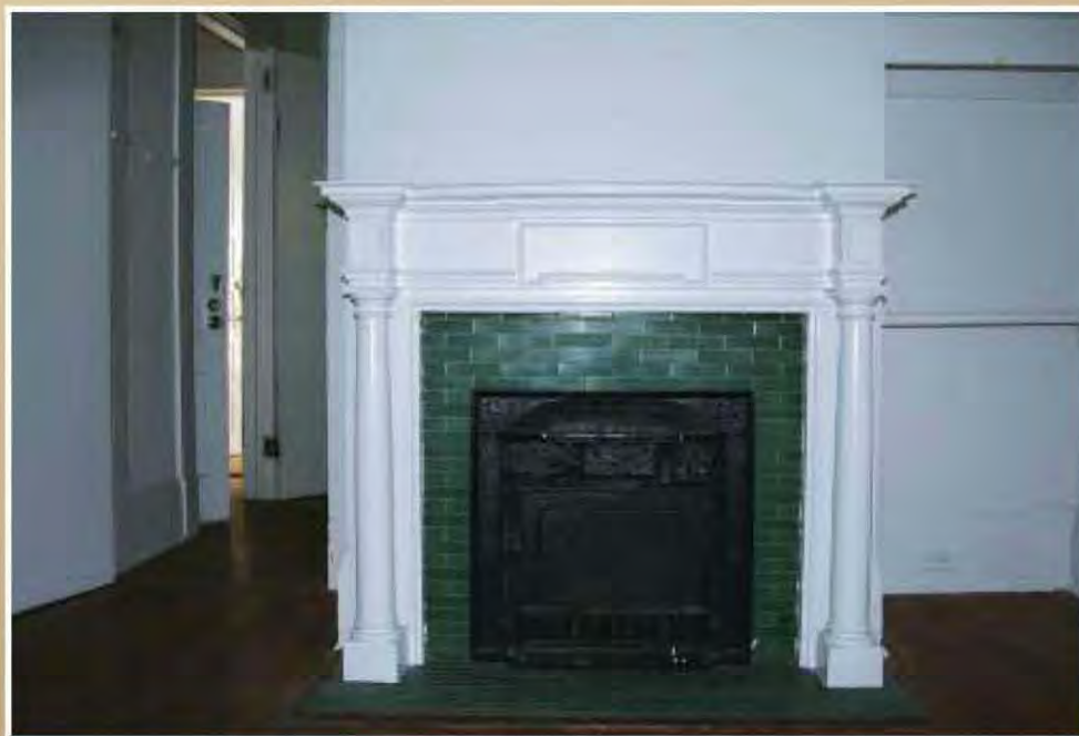
Fig. 6.8: A landlord sealed the fireplace so fraternity members would not burn the house down.
