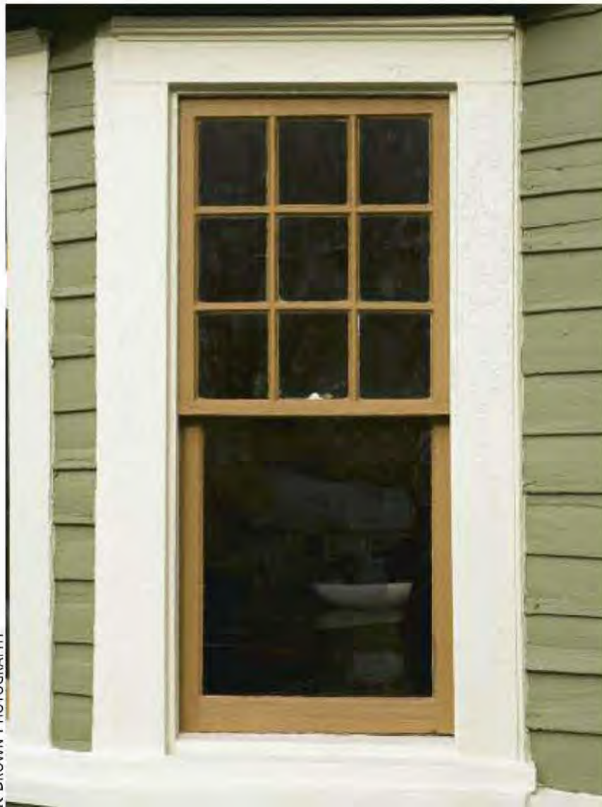
Fig 2.2-3: Detailing unique to historic homes. Preservation incentives and restrictions aim to protect such architectural character.
