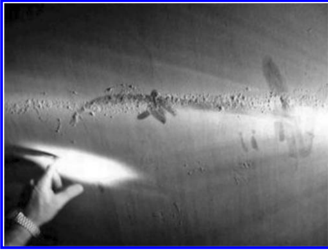
Blistering where a stiffener was welded on the other side of the plate.
