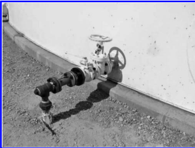
Water draw off piping.
