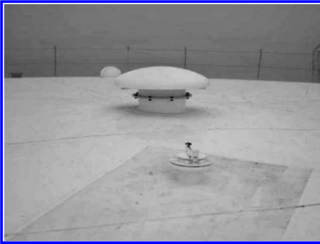
Fixed roof mushroom circulation vent.
