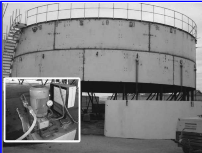
Tank in lifted position (inset hydraulic pump).
