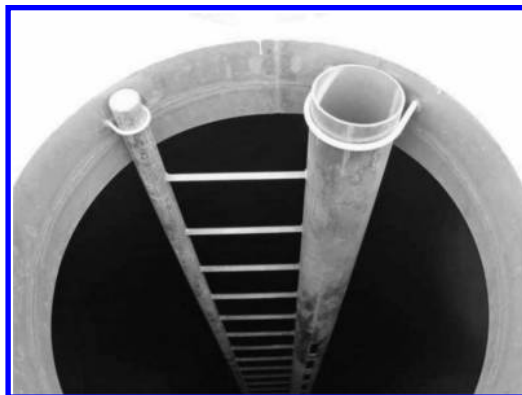
Internal ladder with slotted gauge pole.
