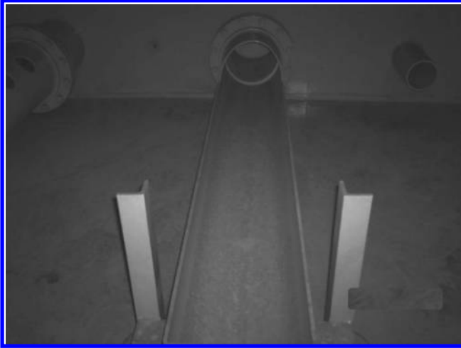
Suction Line Trough
