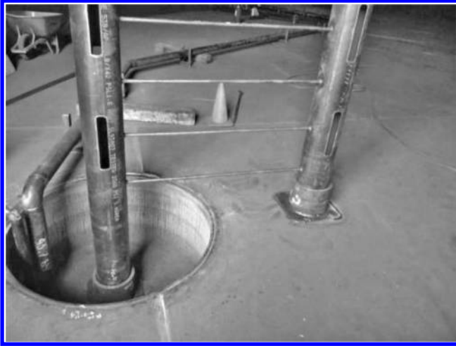
Ladder, slotted gauge pole, and sump.
