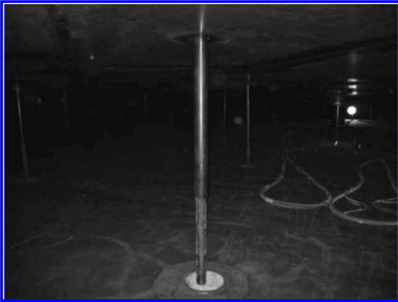
Floating roof support leg and sleeve (high leg position).
