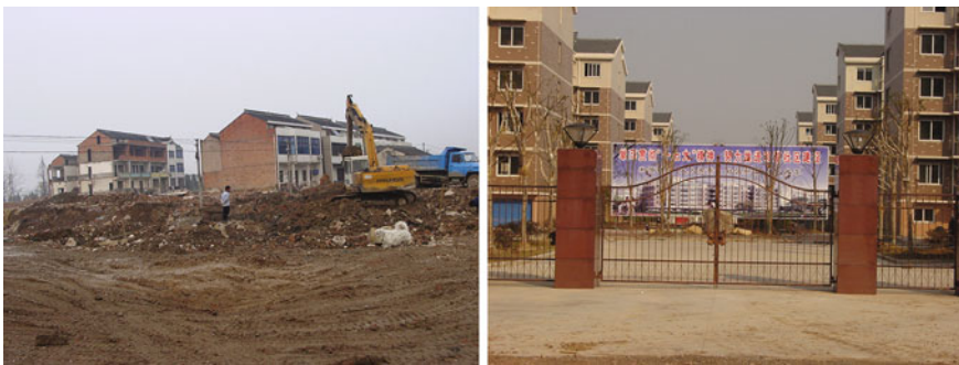
Photo 12.1 Villagers’ traditional homes ( left ) in Jiangsu Province are being demolished to be replaced with “villager apartments” ( right ) (Photo by the author)
