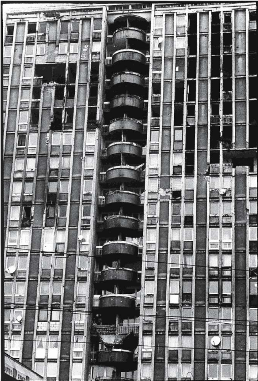
Fig. 5.5 War-torn residential block (Photo: R. Schmid)
