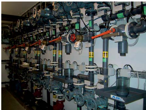
Fig. 22.2. Waste disposal area at the Department of Nuclear Medicine and Endocrinology, PET/CT Center Klagenfurt
