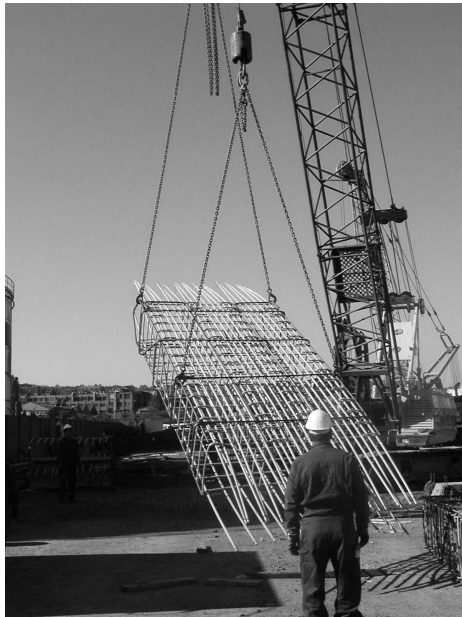
Figure 1.3 Reinforcing cage being readied for placement in forms for a tunneling application. (Courtesy of Hughes Brothers.)
