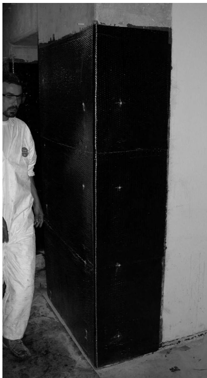
Figure 10.2 FRP shear strengthening of a wall with openings. (Courtesy of Racquel Hagan.)
