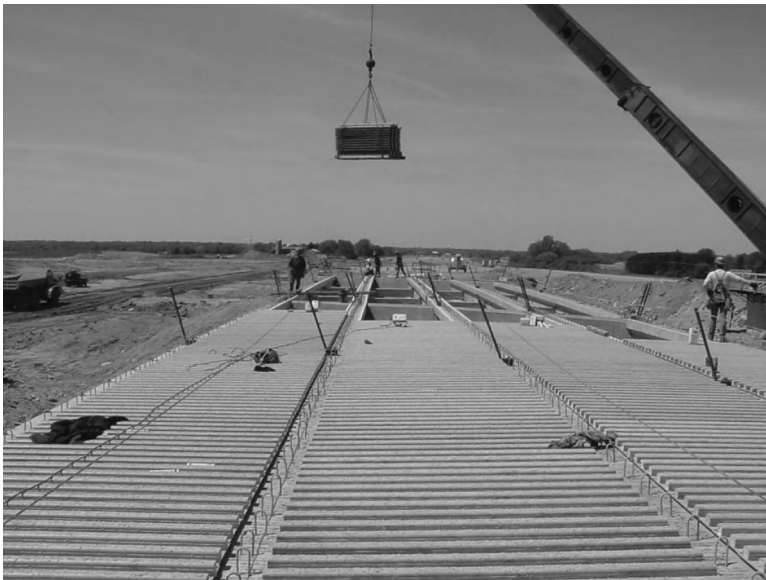
Figure 1.6 Placement of FRP stay-in-place forms for a bridge deck. (Courtesy of Adam Berg.)
