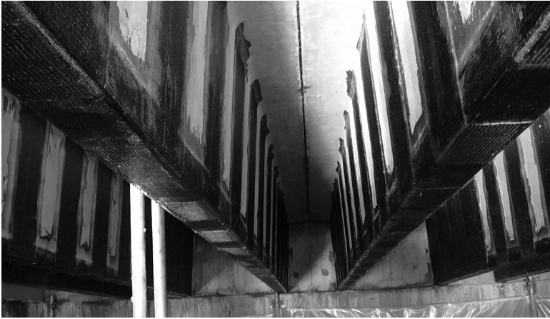
Figure 9.1 Flexural (and shear) strengthening of a reinforced concrete beam. (Courtesy of Fyfe Company.)
