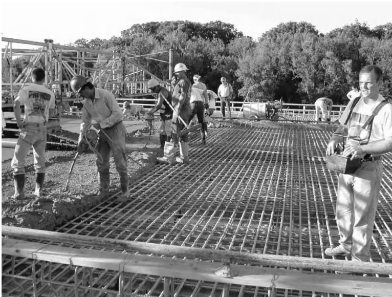
Figure 1.4 Bridge deck slab with a glass FRP top mat being poured. (Courtesy of Hughes Brothers.)
