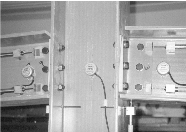
Figure 15.13 Out-of-plane forces in clip angle simple shear beam-to-column connections. (Courtesy of J. T. Mottram.)
