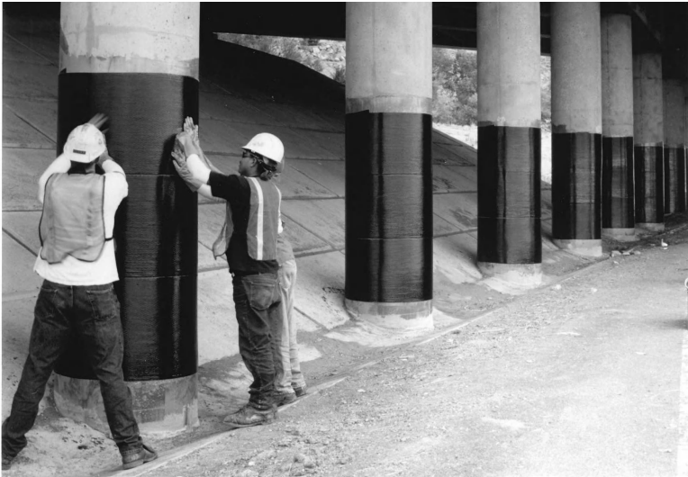
Figure 1.12 FRP wrap being installed on a highway column. (Courtesy of Sika Corporation.)
