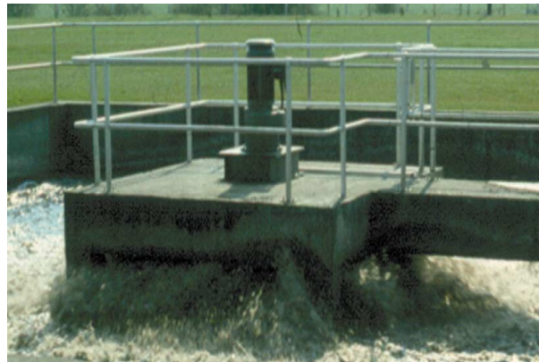
Fig. 5.19. Platform mounted Simcar ® aerator in action.
