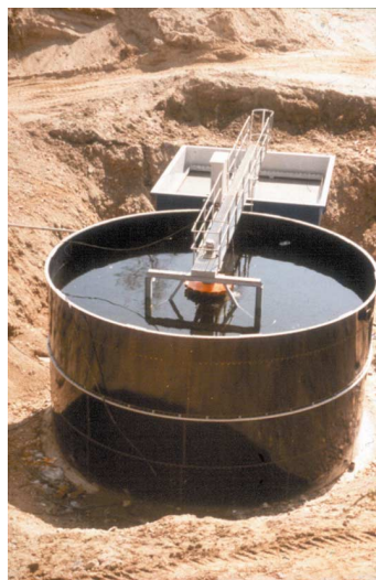
Fig. 5.57. Newly sited aeration tank for 1000 people, with a Euromatic aerator. Sludge separation is by an upflow clarifier with a wedgewire filtration system. Sludge is returned from the centre of the clarifier to the aeration tank by an airlift pump.
