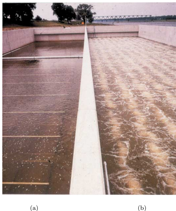
Fig. 5.27. (a) Fine bubble tube aerators mounted on a framework of air supply pipes. (b) Aeration in operation (with permission of Rosewater Engineering Ltd.).
