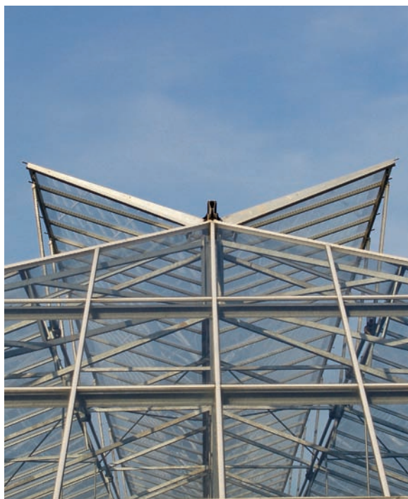
Roof vents that are triggered to open automatically by sensor alerts are far and away the most important component of a greenhouse cooling system. But additional cooling devices may be necessary.
