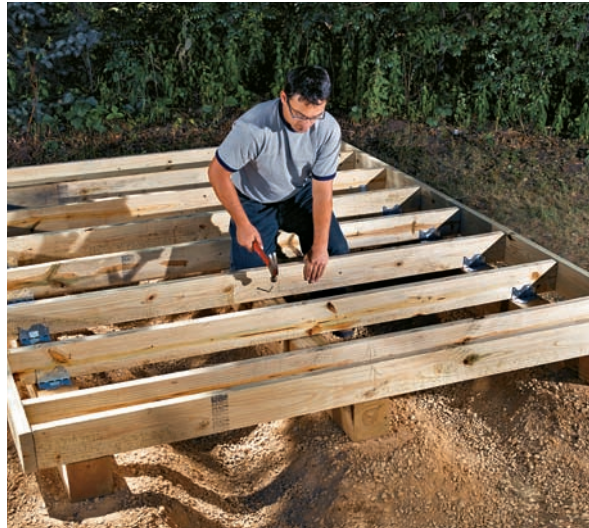
Timbers can be leveled on a well-drained base to create a shed foundation. Drive rebar stakes through the timbers and into the ground to hold them in place.
