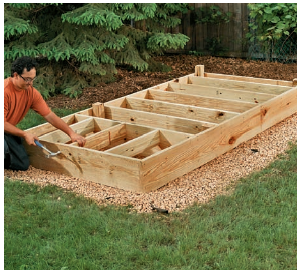
Wood posts set in concrete offer many possibilities for creating a foundation. Here, the floor joists are mounted directly to the sides of the posts with lag screws.
