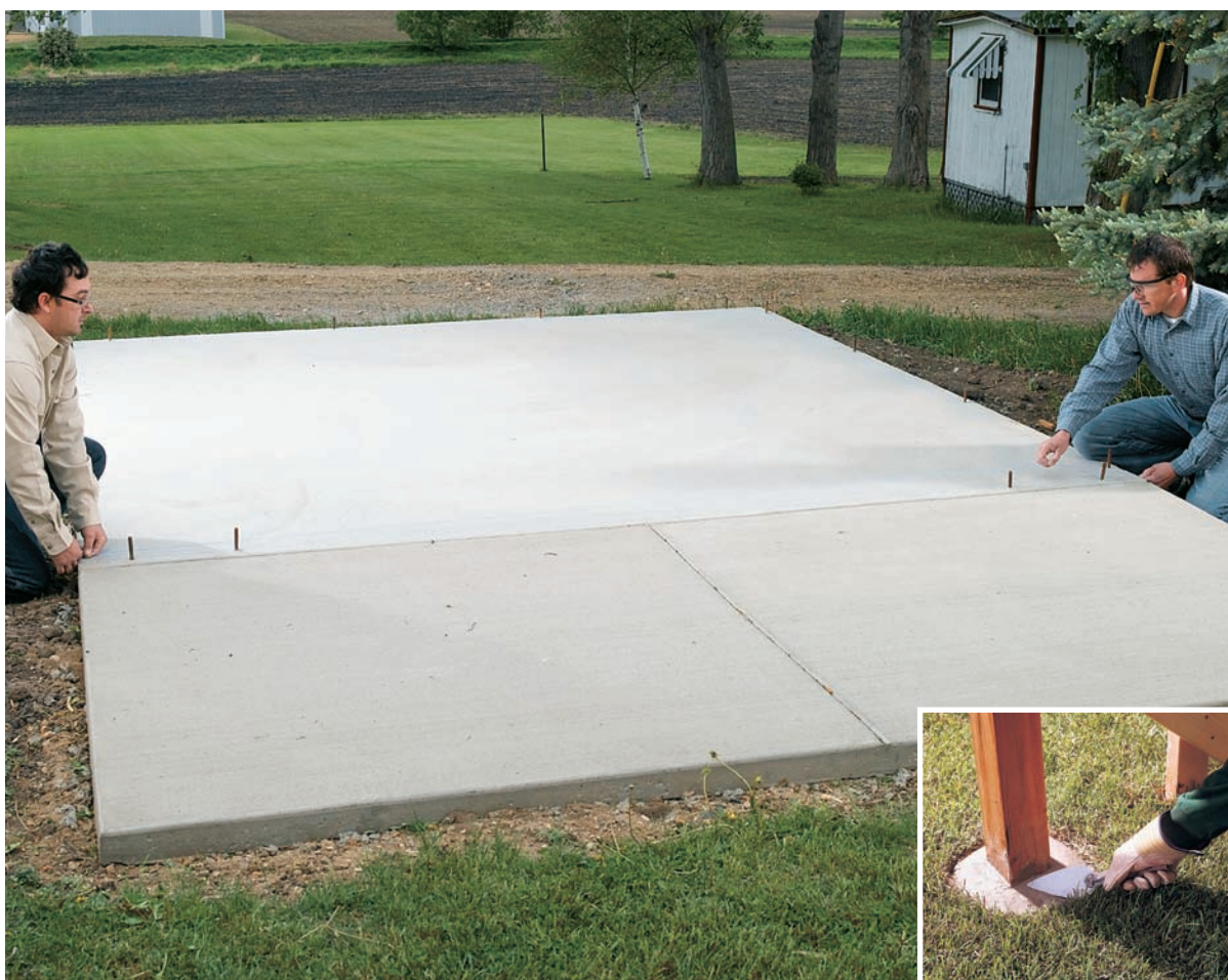
Other foundation options include suspending a floor undercarriage frame from wood posts that are set into concrete (inset), or pouring a concrete slab (above). A concrete slab is an excellent choice if you'll be parking lawn tractors or other vehicles in the shed—especially if a skirt is included to function as a driveway.
