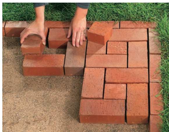
Brick pavers can be set onto a sand bed to create a semipermanent greenhouse floor that offers drainage and looks beautiful.
