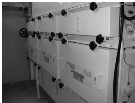
Figure D-3 PVCRI HEPA filter bank. SOURCE: Barbara Johnson, committee member.
