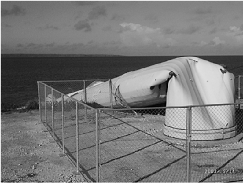
Figure 11.6 A failed wind turbine tower following a typhoon (picture by Dr M.Matsui, Tokyo Polytechnic University).
