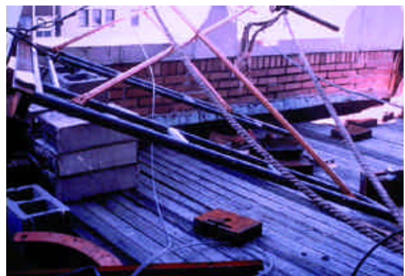
FIGURE 4.9 On top of the building above the decedent, a pulley device with counterweights had been knocked over by high winds. See next photo.
