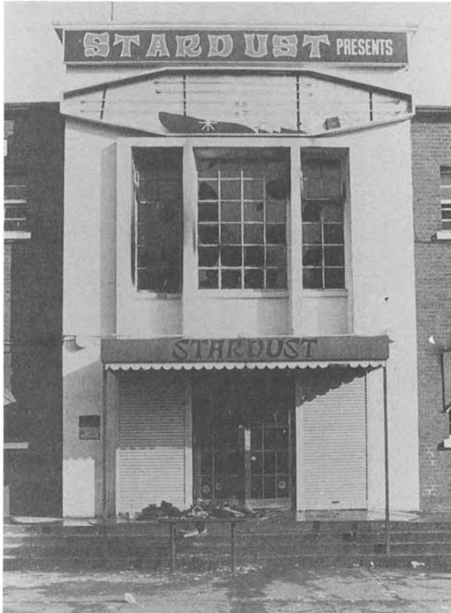
Figure 2. The entrance/main exit showing shutters closed on each side, which opened upwards and without any mechanism to hold them open
