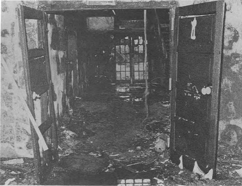
Figure 4. The main exits from the inside after the fire
