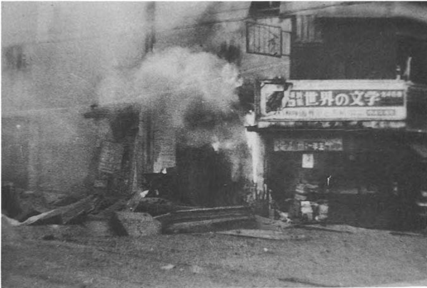
Figure 1. Blown out concrete blocks and burning houses at the construction site gas explosion accident
