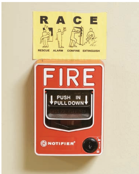
FIGURE 3-9 Fire extinguisher. Fire pull and RACE card.
