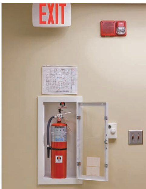
FIGURE 3-10 Fire extinguisher with evacuation plan and fire alarm.
