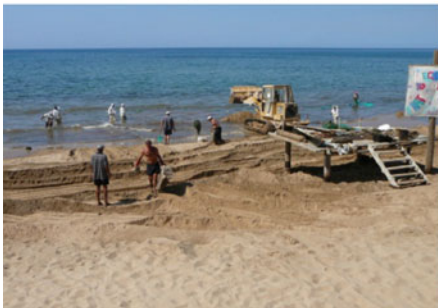
Sand washing operation to remove oil spilled from the Jiyah power plant spill, Lebanon.
