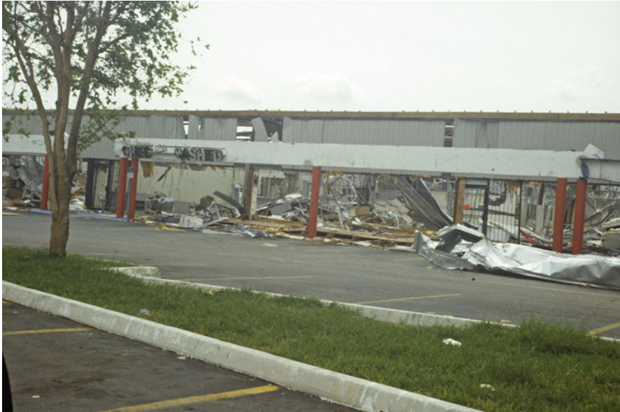
Fig. 1.4 Shopping center in Homestead, Florida, situated just south of the Miami metro area, showing complete destruction shops in this mall by Hurricane Andrew. Tornadoic winds associated with H. Andrew devastated many built-up areas, attesting to the hazards posed by hurricane-related wind fields (Photograph by C.W. Finkl)
