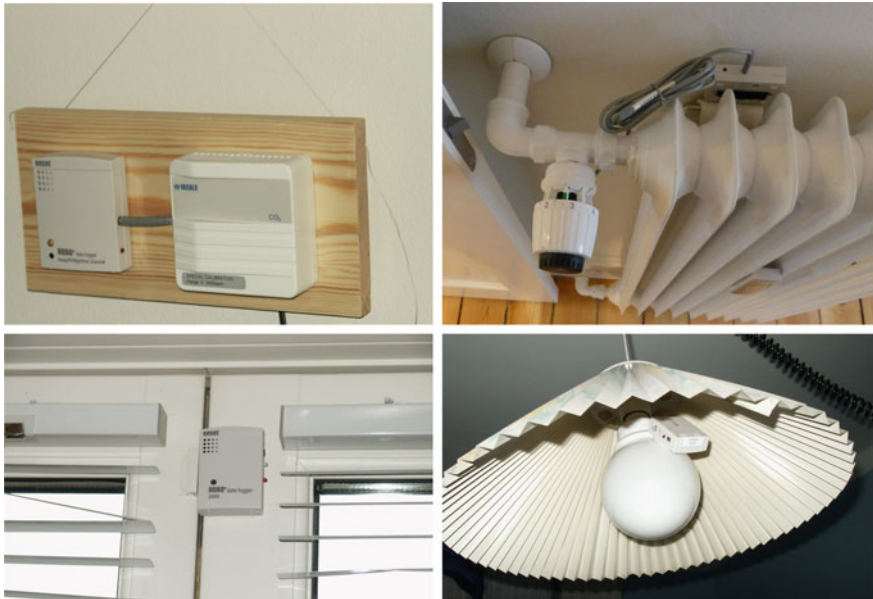
Fig. 6.8 Example stand-alone sensor systems. Clockwise from top-left CO 2 concentration sensor connected to data logger; custom-built thermostatic radiator valve position sensor connected to a data logger; light state logger; and operable window state logger (photos from Rune Andersen)
