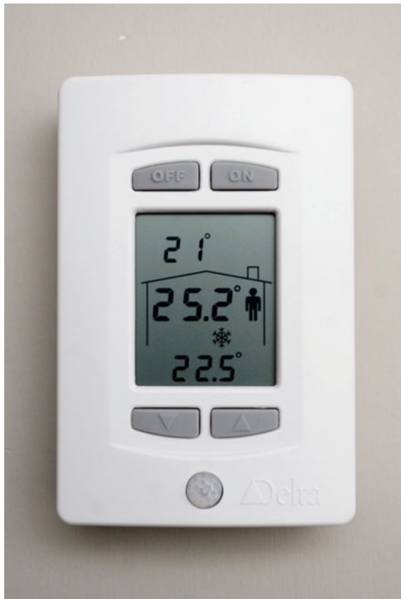
Fig. 6.3 Example thermostat with buttons for light switching and temperature setpoints adjustment, which also measures occupancy, CO 2 concentration, temperature, and relative humidity
