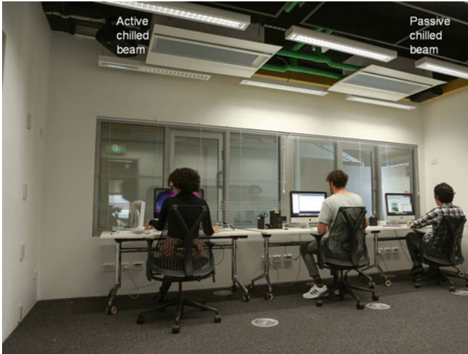
Fig. 7.12 Passive and active chilled beam systems in chamber 2 of the IEQ Lab (photo by Richard de Dear, University of Sydney)
