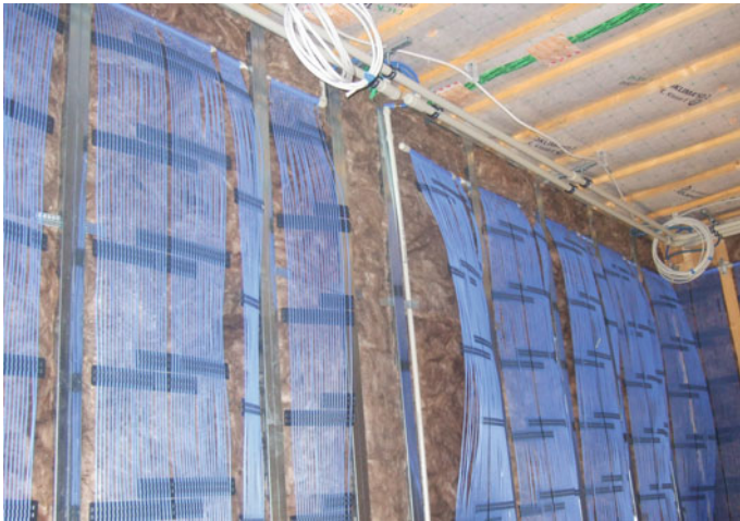
Fig. 7.15 Capillary tube systems for radiant heating and cooling with low thermal inertia; installed in the LOBSTER (photo by Marcel Schweiker, KIT)
