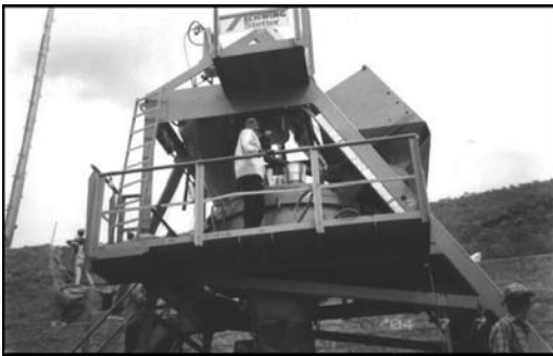
Figure 6. Concrete Batching plant erected on site.
