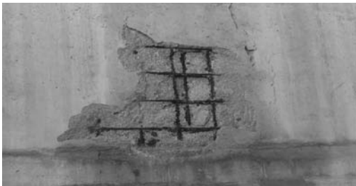
Figure 1. The bulk of durability problems concern the corrosion of reinforcing steel.
