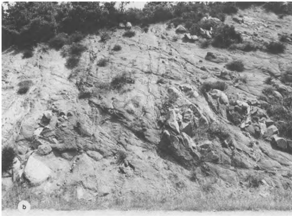
Fig. 4.4 (b). Corestones and grus with veins in situ exposed in road cutting in northeastern Sardinia (R.F. Peel).
