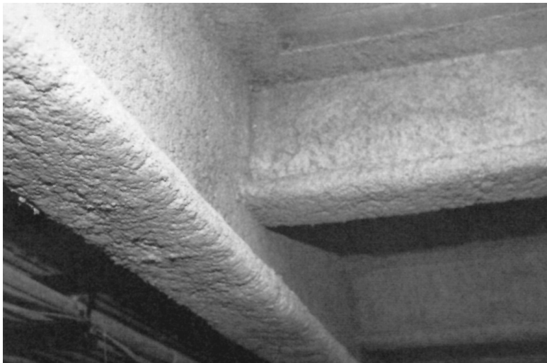
Figure 11.6 Sprayed-on friable asbestos fireproofing.
