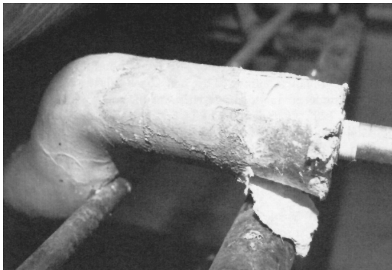
Figure 11.7 Partially damaged asbestos thermal system insulation.
