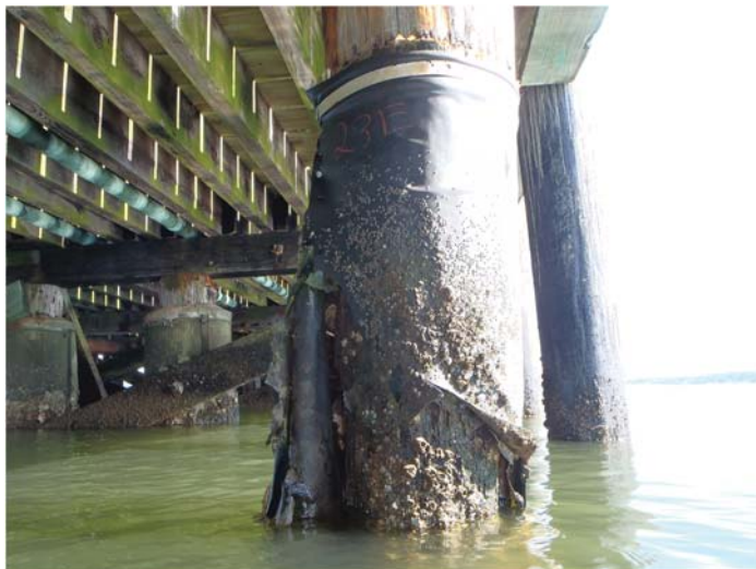
Fig. B-33. Torn PVC wrap exposing a timber fender pile
