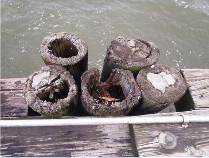
Fig. B-21. Rot at the top of timber fender piles
