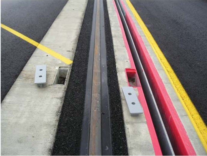
Fig. A-62. Cable trench (to the right of the crane rail)
