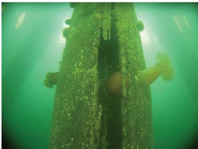
Fig. B-20. Underwater photograph showing hollowing of the interior of a timber pile from Teredo
