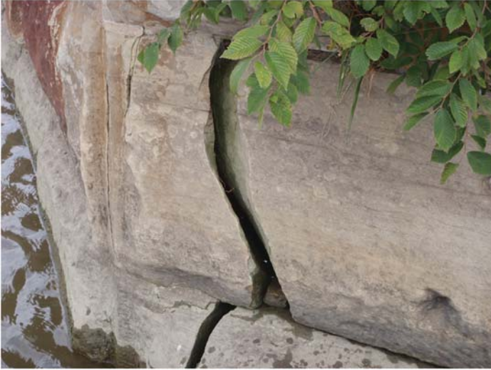
Fig. A-23. Cracking through masonry blocks
