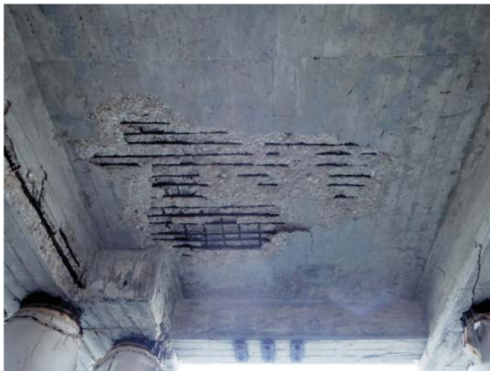
Fig. B-6. Open corrosion spall on the underside of a reinforced concrete deck Source: Courtesy of Marine Solutions, Inc., reproduced with permission.
