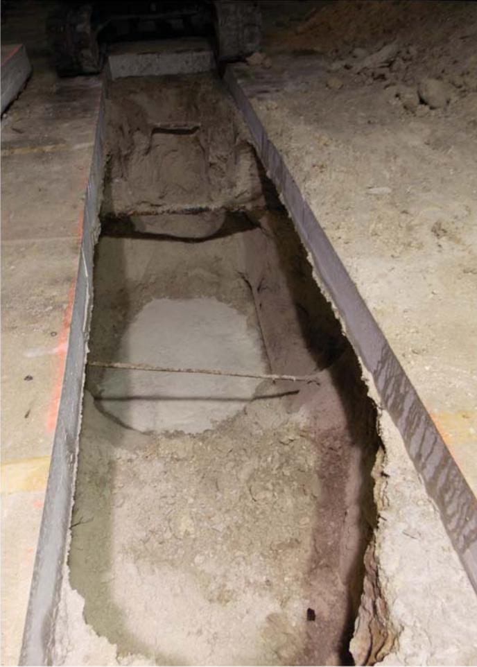
Fig. C-24. Excavation of tie rod to measure remaining tie rod area Source: Courtesy of Collins Engineers, Inc., reproduced with permission.
