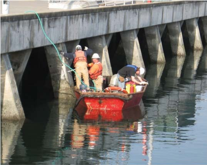
Fig. 4-2. Coring operations over water to extract samples from prestressed piles Source: Courtesy of Appledore Marine Engineering, Inc., reproduced with permission.
