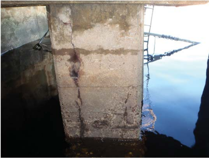
Fig. B-3. Typical corrosion crack on a reinforced concrete pile Source: Courtesy of Marine Solutions, Inc., reproduced with permission.
