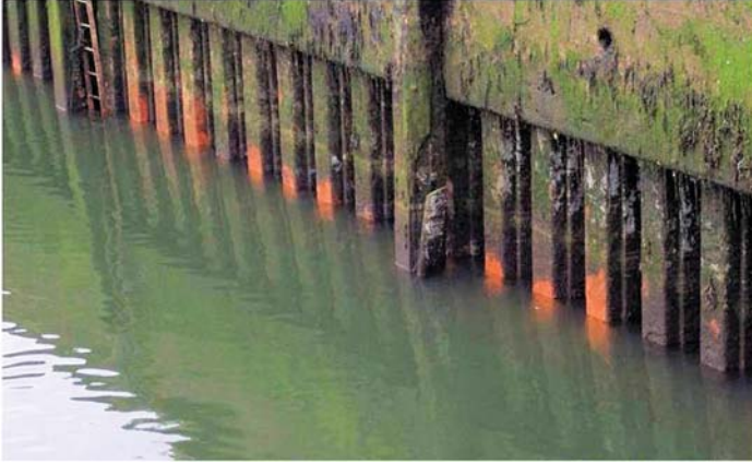
Fig. C-36. Steel sheeting bulkhead with living MIC colonies near low water level Source: Courtesy of Collins Engineers, Inc., reproduced with permission.
