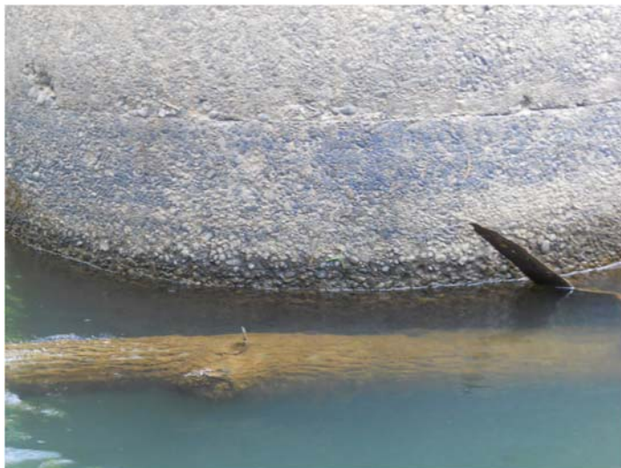
Fig. B-11. Concrete scaling at the water surface
