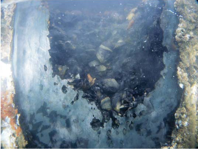
Fig. A-29. Underwater photograph showing a hole in a cellular structure due to corrosion
