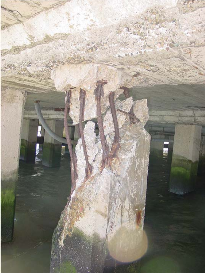
Fig. A-8. Severely damaged concrete pile from vessel impact Source: Courtesy of Simpson Gumpertz & Heger, Inc., reproduced with permission.
