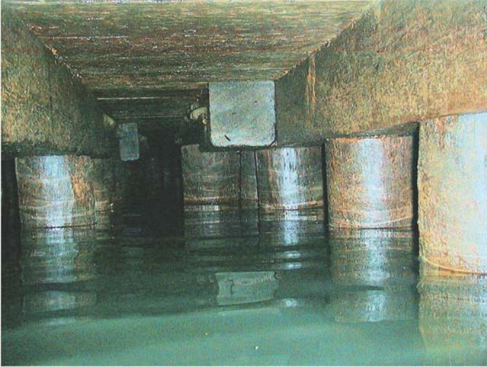
Fig. A-15. Underside of relieving platform at extreme low tide; access and inspection of deck components can be difficult and often requires penetration diving techniques
