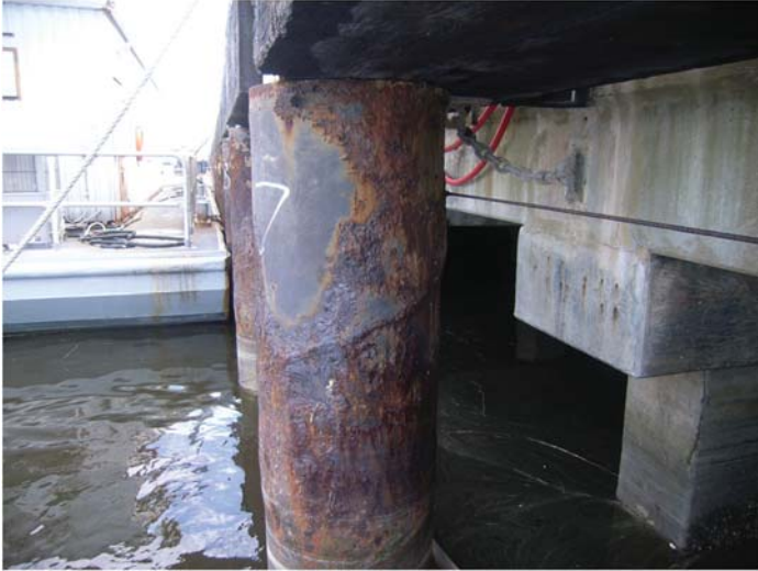
Fig. B-32. Deteriorated coal-tar epoxy polyamide coating resulting in corrosion of a steel fender pile
