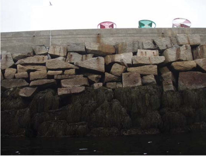
Fig. B-25. Erosion and movement of a masonry block structure
