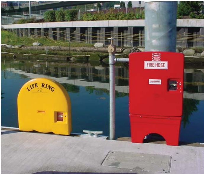
Fig. A-53. Typical float-mounted appurtenances: throw ring, fire hose, and fire pull box
