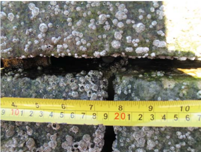
Fig. B-28. Close up view of loss of mortar between masonry blocks
