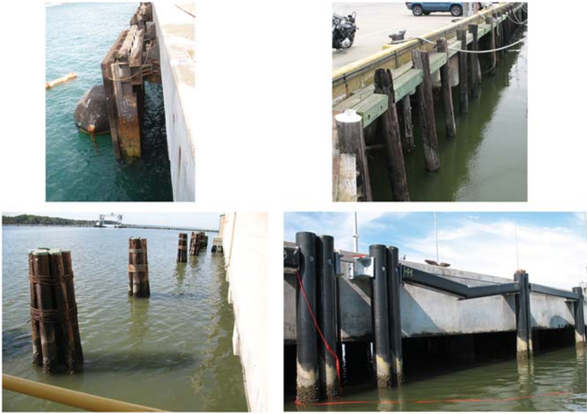
Fig. A-44. Steel H-piles supporting a timber fender framing and rub strip (top left), timber fender pile system (top right), clusters of timber fender piles banded together with wire rope (bottom left), composite fender pile system with a broken wale (bottom right)
