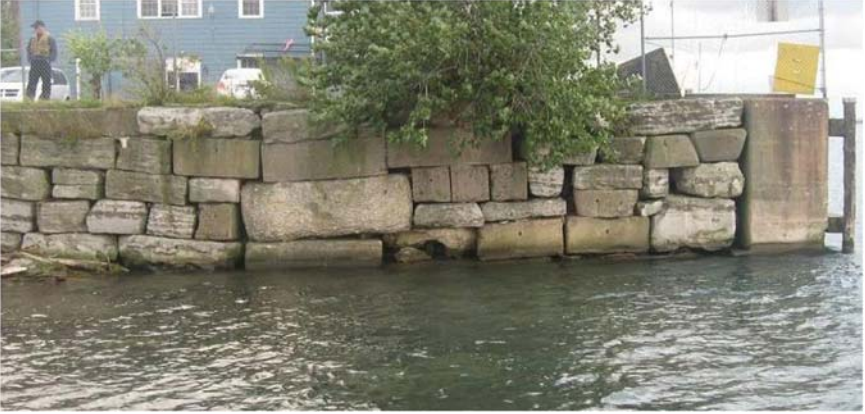
Fig. A-20. Settlement and bowing of masonry block seawall Source: Courtesy of Marine Solutions, Inc., reproduced with permission.
