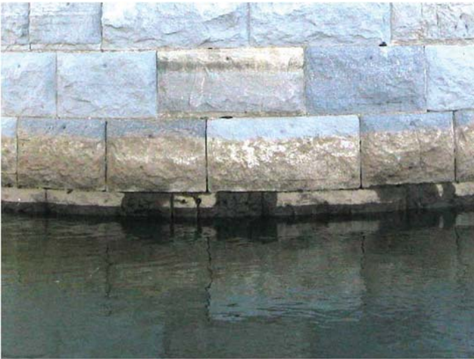
Fig. A-21. Erosion of masonry blocks at the water surface Source: Courtesy of Marine Solutions, Inc., reproduced with permission.
