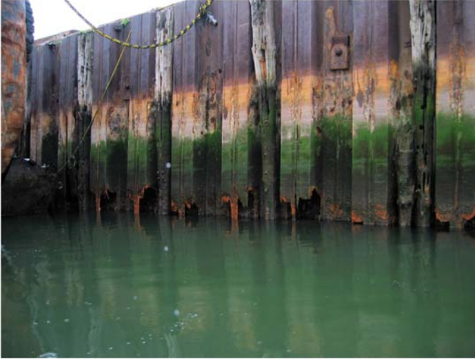
Fig. A-17. Severely deteriorated steel sheet pile bulkhead
