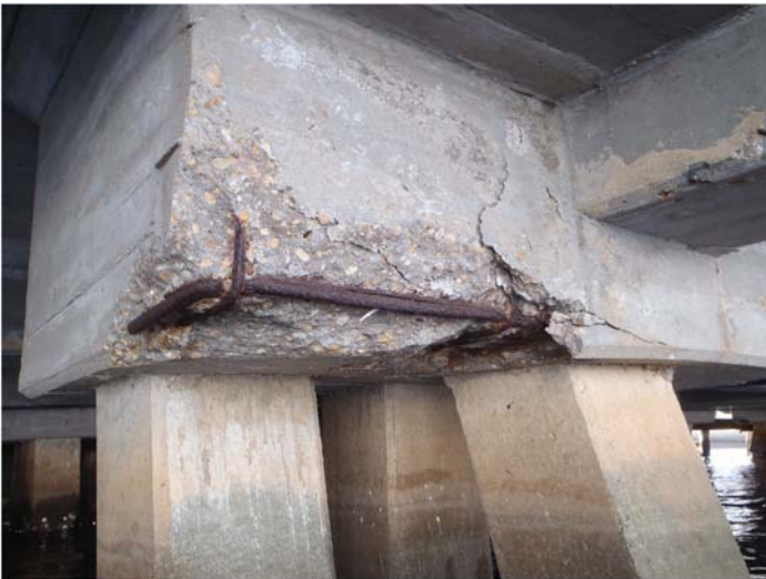
Fig. B-5. Open corrosion spall on the corner of a reinforced concrete pile cap Source: Courtesy of Marine Solutions, Inc., reproduced with permission.
