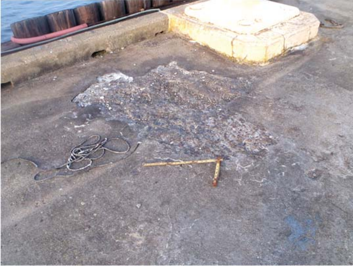
Fig. B-7. Delaminated area on a reinforced concrete pier deck Source: Courtesy of Marine Solutions, Inc., reproduced with permission.
