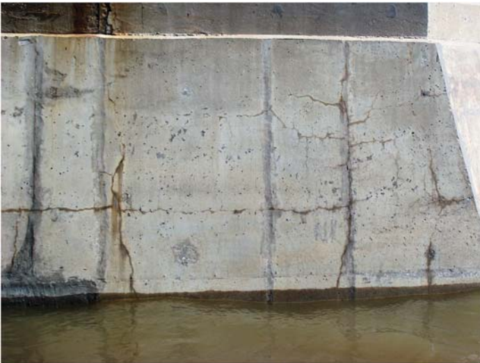
Fig. B-2. Nonstructural cracking on the face of a concrete bulkhead Source: Courtesy of Marine Solutions, Inc., reproduced with permission.
