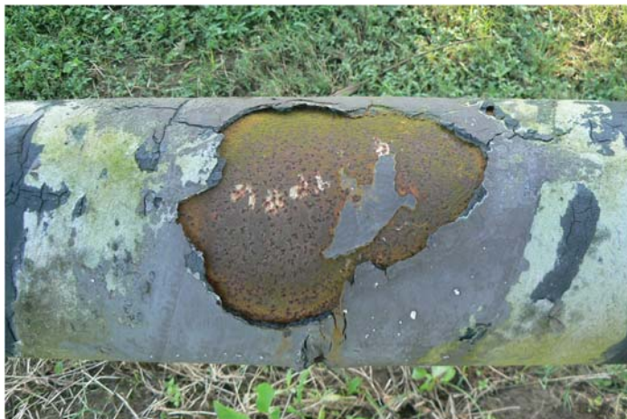
Fig. B-31. Coating failure on steel bracing Source: Courtesy of Marine Solutions, Inc., reproduced with permission.
