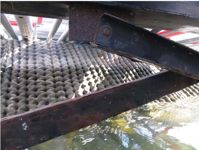
Fig. A-13. Corrosion of steel bracing
