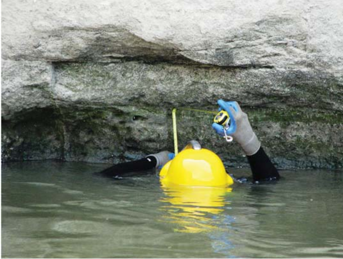
Fig. B-15. Diver measuring severe erosion damage
