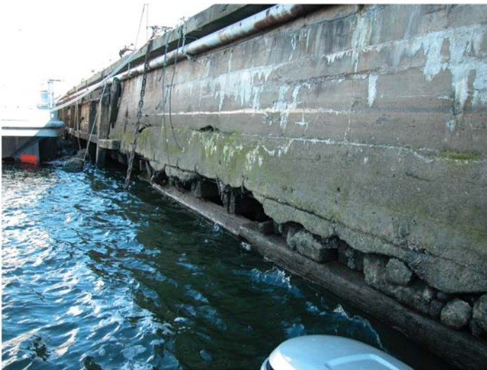
Fig. A-14. Deteriorated relieving platform
