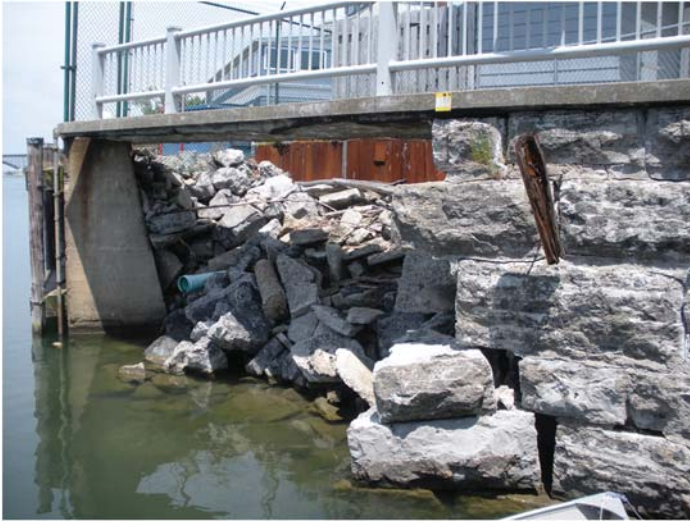
Fig. A-24. View of a collapsed section of masonry block wall due to insufficient foundation support
