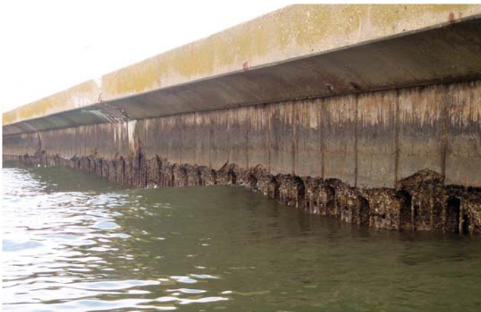
Fig. B-14. Severe erosion of a concrete sheet pile breakwater Source: Courtesy of Marine Solutions, Inc., reproduced with permission.
