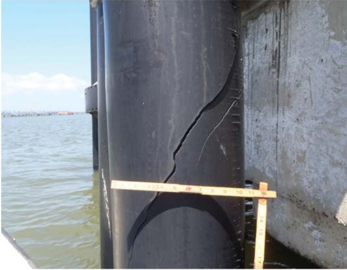
Fig. B-30. Cracked FRP pile from vessel impact Source: Courtesy of Marine Solutions, Inc., reproduced with permission.
