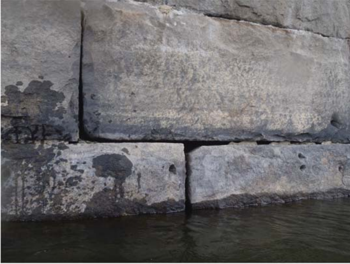
Fig. A-22. Loss of mortar between masonry block units Source: Courtesy of Marine Solutions, Inc., reproduced with permission.
