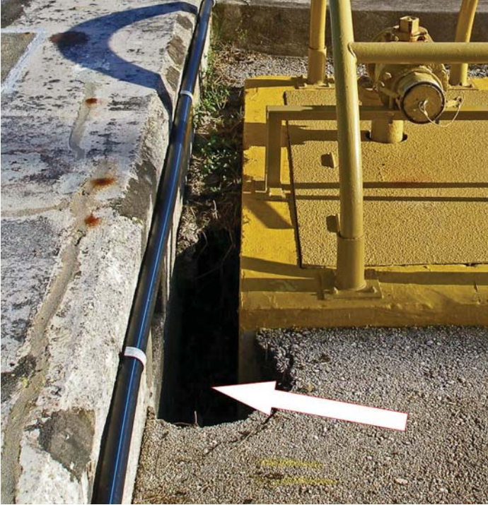
Fig. A-30. Hole in pavement (arrow) due to erosion behind sheet pile bulkhead Source: Courtesy of Moffatt & Nichol, Inc., reproduced with permission.
