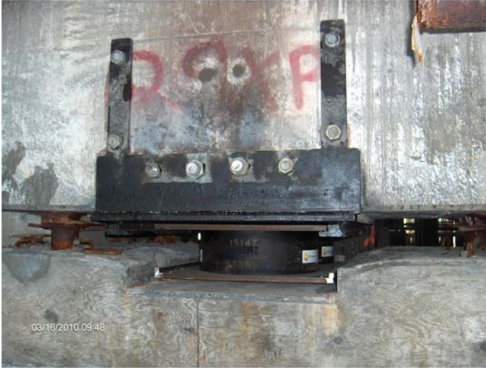
Fig. B-34. View of a lead-rubber base isolation unit installed below pier deck Source: Courtesy of Moffatt & Nichol, Inc., reproduced with permission.
