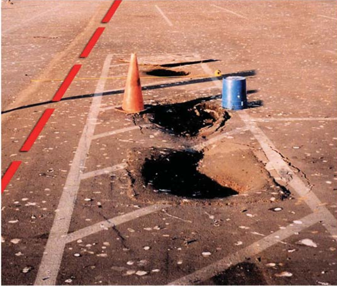
Fig. A-37. The pavement has failed entirely as a result of soil migrating from beneath the pendant wall below (indicated by the dashed line)
