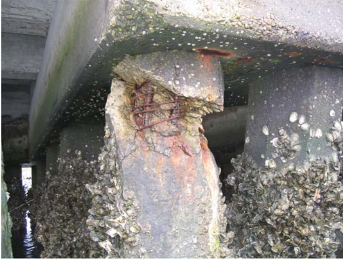
Fig. B-10. Reinforced concrete pile with impact damage
