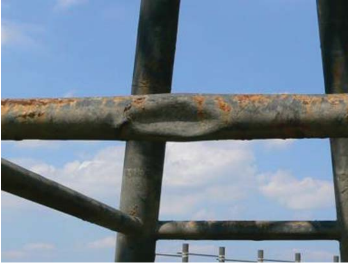
Fig. B-18. Impact damage on a steel brace
