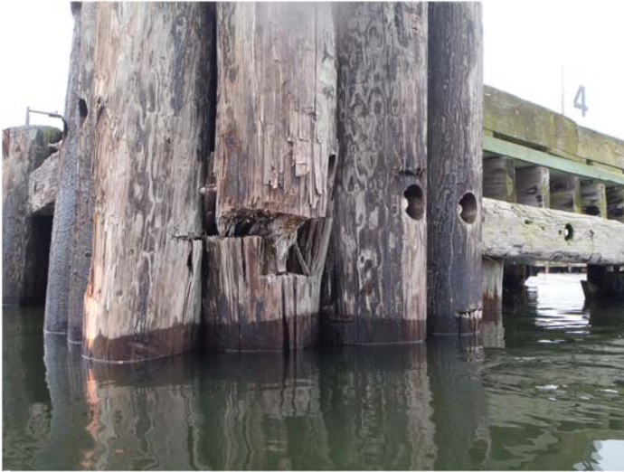
Fig. B-23. Impact damage on a timber fender pile
