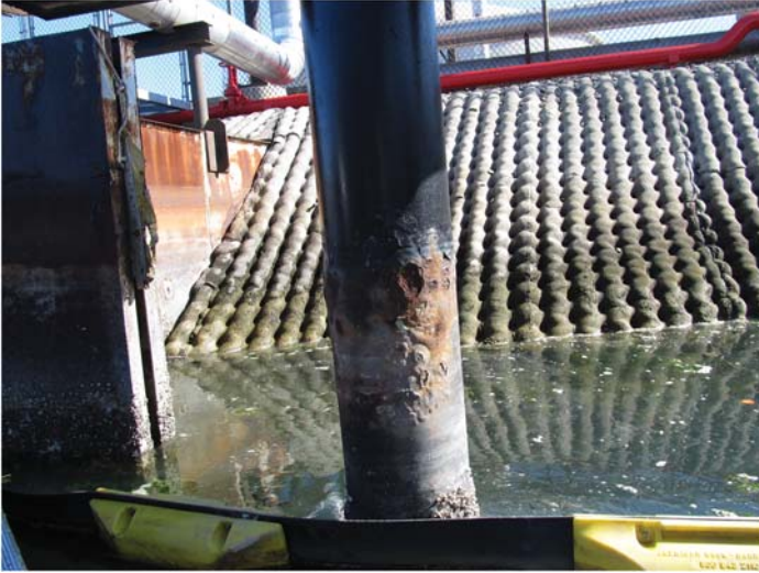
Fig. A-12. Pitting and splash zone corrosion of steel pile
