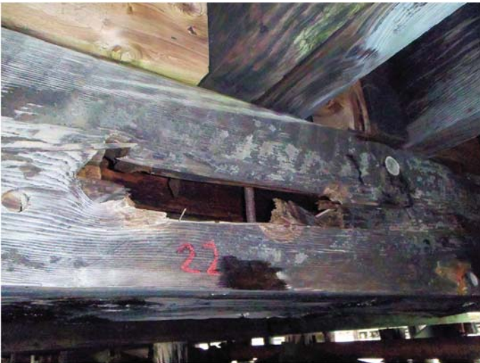
Fig. B-22. Severe rot due to moisture located on a timber beam
