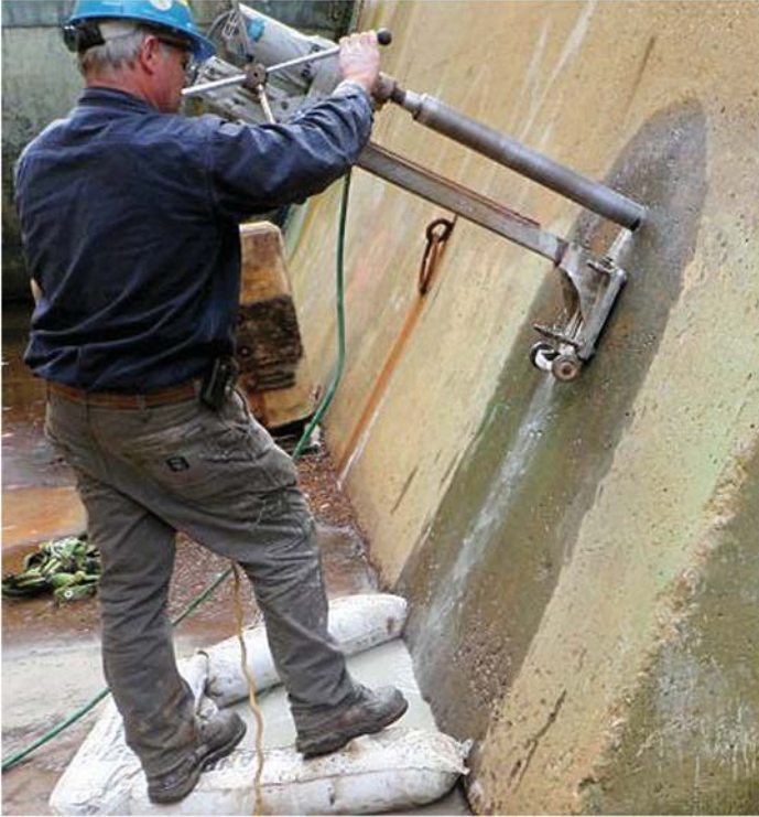
Fig. 4-3. Coring operation of dry dock wall; note wastewater containment Source: Courtesy of Appledore Marine Engineering, Inc., reproduced with permission.
