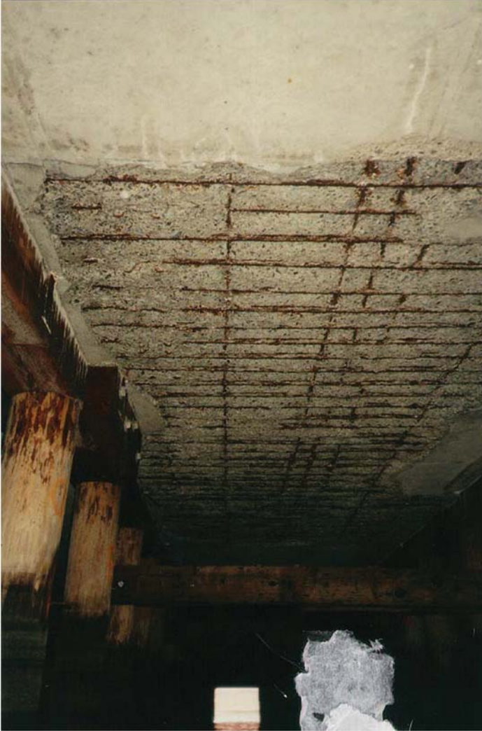
Fig. A-10. Corroded underside of concrete deck Source: Courtesy of CH2M HILL, Inc., reproduced with permission.
