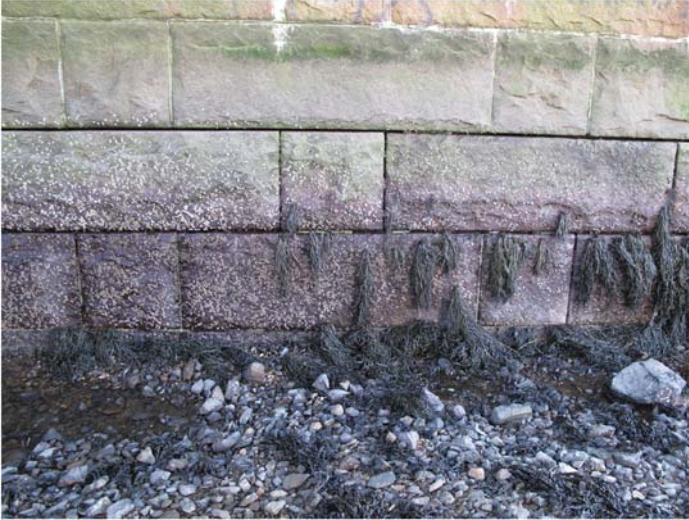
Fig. B-27. Mortar degradation in the tidal zone
