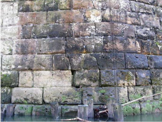
Fig. B-26. Splitting of masonry blocks
