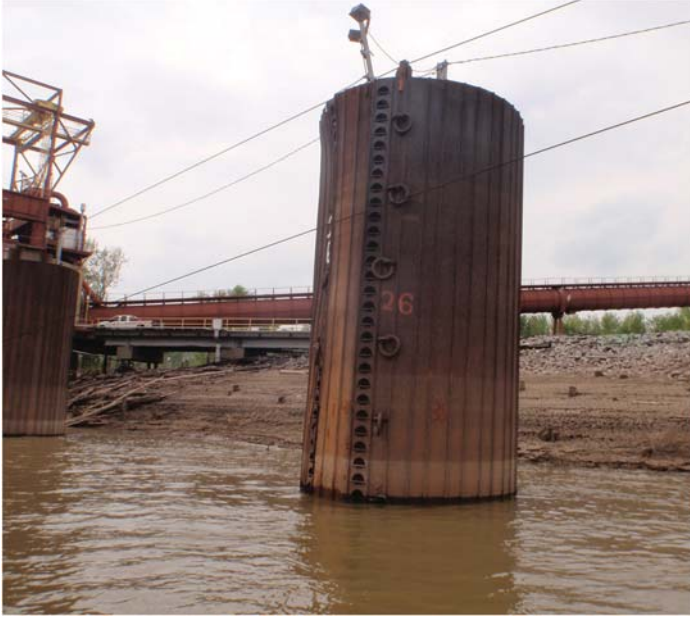
Fig. A-27. Leaning of a cellular structure due to scour and slope instability Source: Courtesy of Marine Solutions, Inc., reproduced with permission.
