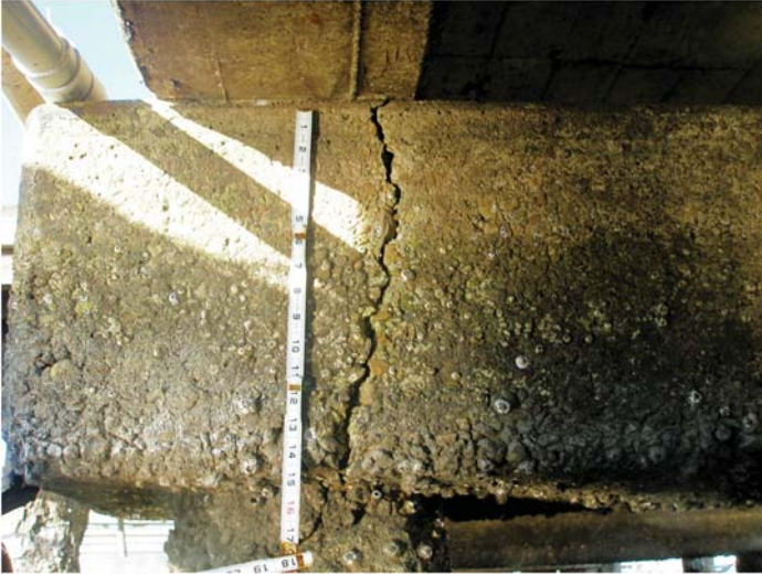
Fig. B-1. Structural crack on a reinforced concrete pile cap Source: Courtesy of Marine Solutions, Inc., reproduced with permission.
