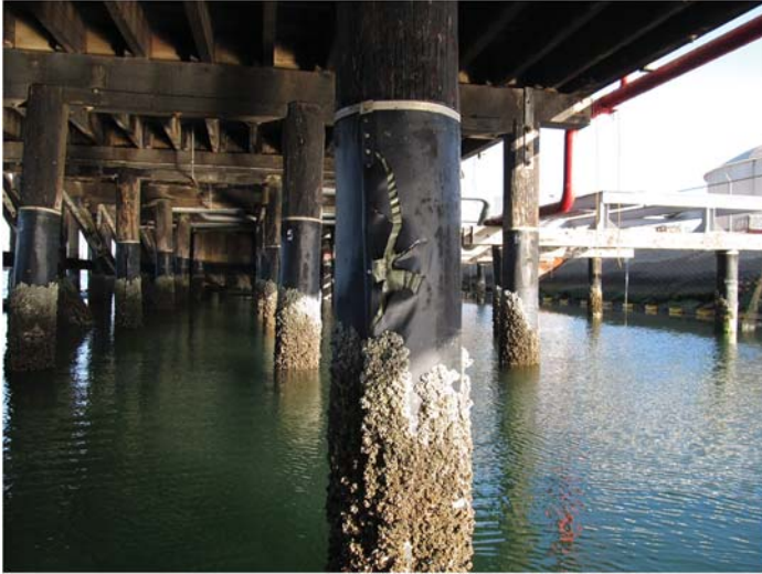
Fig. A-5. Typical timber pile with wrap damage; note wrap tear that originates from the nailed seam
