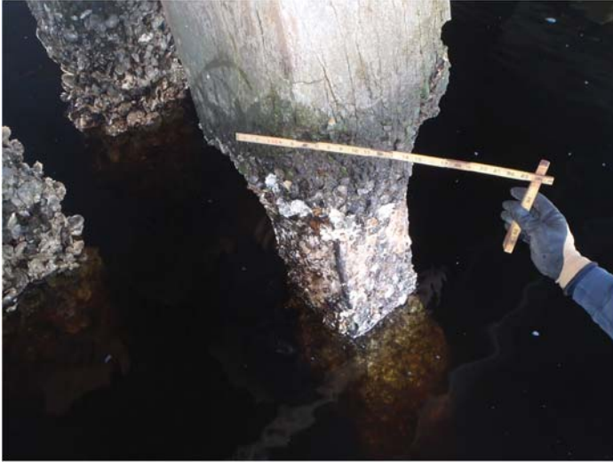
Fig. B-9. Reinforced concrete pile with loss of section below the high tide level Source: Courtesy of Marine Solutions, Inc., reproduced with permission.
