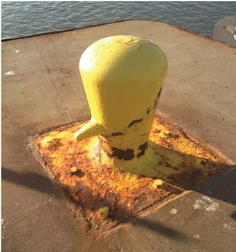
Fig. A-40. Severe anchorage corrosion of a cleat (top) and a bollard (bottom) Source: Courtesy of Simpson Gumpertz & Heger, Inc., reproduced with permission.
