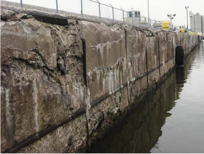
Fig. B-12. Freeze-thaw damage along the face of a reinforced concrete bulkhead Source: Courtesy of Marine Solutions, Inc., reproduced with permission.
