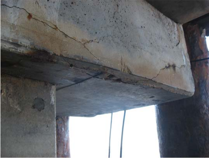
Fig. B-4. Cracking indicating a closed corrosion spall on the corners of a pile cap Source: Courtesy of Marine Solutions, Inc., reproduced with permission.
