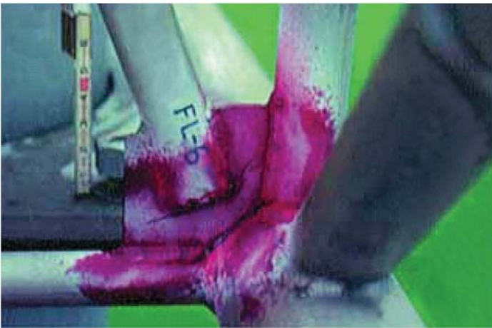
Fig. C-17. Gusset plate with applied dye penetrant Source: Courtesy of Collins Engineers, Inc., reproduced with permission.
