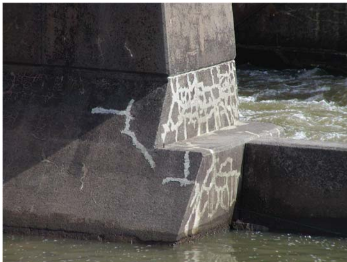
Fig. B-8. Epoxy-covered cracks formed from ASR
