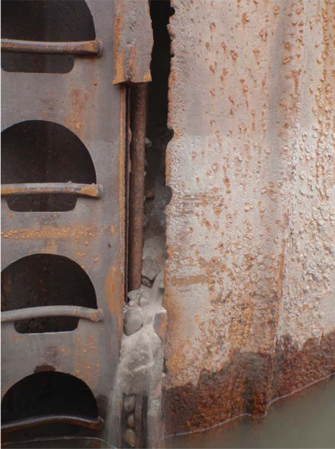
Fig. A-28. Broken and separated sheet pile interlock resulting in the loss of infill material
