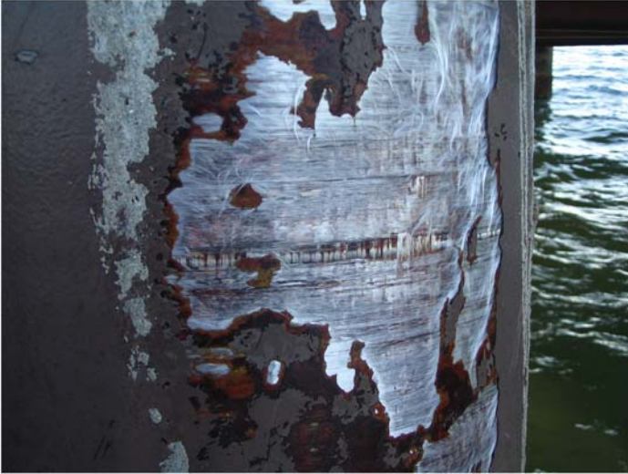
Fig. B-29. Degraded fiberglass-reinforced pile casing showing abraded fibers Source: Courtesy of Marine Solutions, Inc., reproduced with permission.
