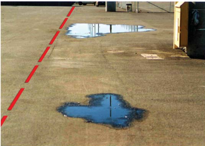
Fig. A-36. The ponding seen in this photo indicates subsidence, probably through the pendant wall below (delineated by the dashed line) Source: Courtesy of Moffatt & Nichol, Inc., reproduced with permission.
