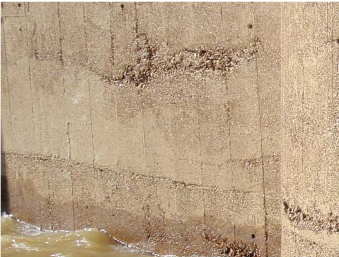
Fig. B-13. Honeycombing on the side of a reinforced concrete bulkhead Source: Courtesy of Marine Solutions, Inc., reproduced with permission.
