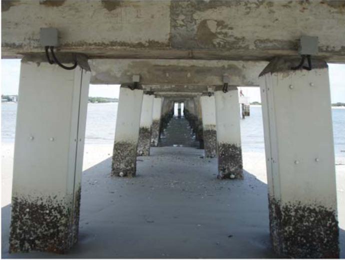
Fig. 4-1. Concrete pier with pile jackets incorporating cathodic protection to increase service life
