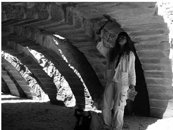
Figure 14.23. Cistern at Humayma with an arched roof (scale provided by Dr Claire Rambeau) (© R. Foote).
