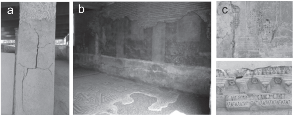
Figure 2. a. Restored column; b. Damages caused by cement pavement in Basilica House; c. Metallic elements.
