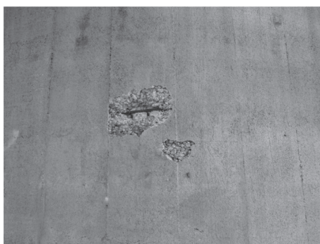
Figure 2. Spalling due to corrosion of reinforcement in the upper zone.
