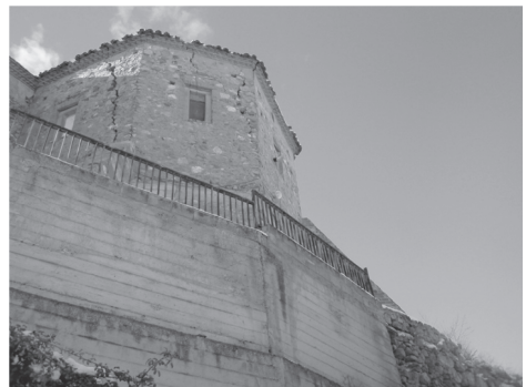
Figure 2. Actual church situation, over a retain-ing wall and very cracked, specially the apse.
