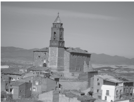
Figure 1. Church actual state. It is sited on vil-lage top. The roof is broken. Some of the neigh-bouring houses are collapsing.
