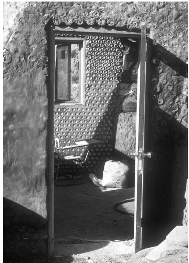
Figure 29-7 Students at the University of Cincinnati built an experimental passive solar greenhouse using all recycled materials, inspired by the work of Mike Reynolds. The materials included tires rammed with earth, bottles, and aluminum cans.
