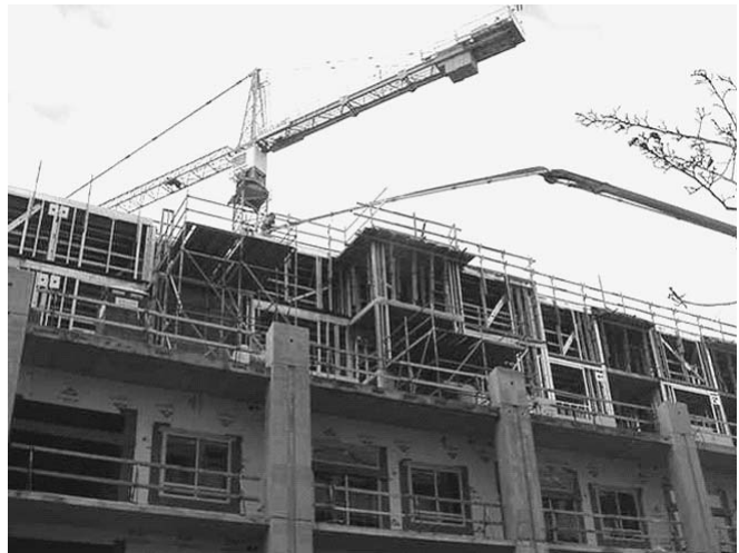
Figure 17-4 Commercial high-rise building under construction, showing a tower crane and the arm of a concrete pump truck.
