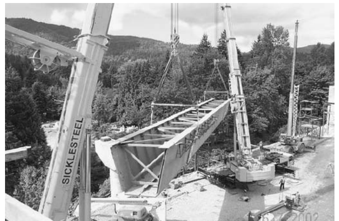
Figure 17-6 Bridge construction with two cranes lifting and then setting a large steel girder.
