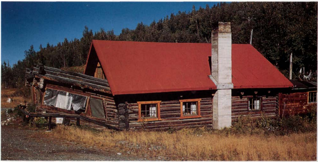
Figure 10.23 This cabin in central Alaska settled more than a meter in 8 years as permafrost beneath its foundation thawed.
