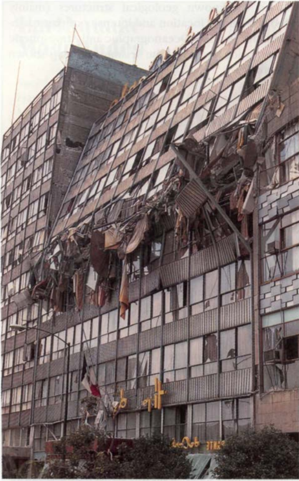
Figure 3.10 A building that was not constructed to withstand expected earthquakes, the Hotel DeCarlo, was one of the buildings that collapsed during the earthquake that struck Mexico City in 1985. Proper building design can minimize damage. Nearby buildings of sturdier construction withstood the shaking.
