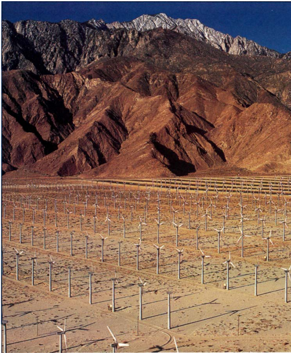
A wind farm at Corgonia Pass, near Palm Springs, California. Each windmill drives a generator.
