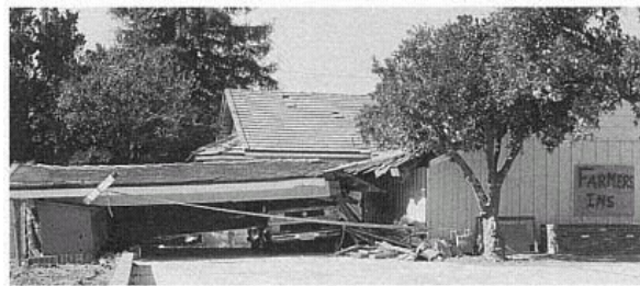
Figure 39 Typical Carport Collapse, San Fernando Valley. Nearly one-third of the insured losses were of appurtenant structures such as carports and garden walls. (Mary C. Comerio)
