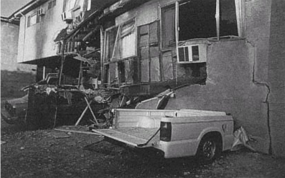
Figure 42 Stucco Failure in Collapsed Multifamily Building. After soft first stories, the second major cause of damage was insufficient shear strength in stucco walls. (© J. Scott Smith)
