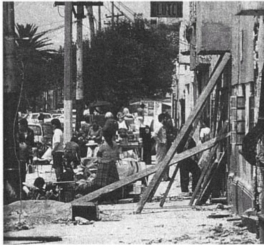
Figure 51 Wooden Bracing for Damaged Buildings. Most viviendas would have been considered uninhabitable before the earthquake, even though most had been occupied by the same families for twenty to thirty years. (Christopher Arnold)
