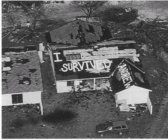
Figure 32 Wind-Damaged Home with "I SURVIVED ANDREW" on Roof. A home owner broadcast a message from the remains of his house. (Raul De Molina, Sygma)
