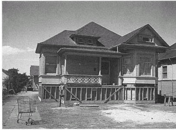
Figure 25 Home Repair, Watsonville. Damaged homes in Watsonville were rebuilt with new foundations and cripple walls. (Mary C. Comerio)
