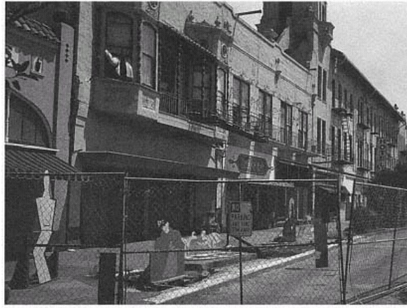
Figure 22 St. George Hotel, Fenced before Demolition. Four hundred residential hotel rooms in four buildings were destroyed in Santa Cruz. Most of the tenants were elderly. (Mary C. Comerio)
