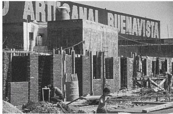
Figure 54 New Low-Rise Housing under Construction. Nearly forty-eight thousand new units were built in two years. (Christopher Arnold)
