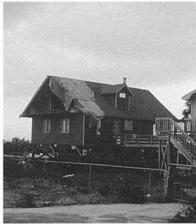
Figure 17 Typical Minor Roof Damage. Costly damage results from improperly secured roofs, because water soaks the interior finishes and contents. (Peter R. Sparks)
