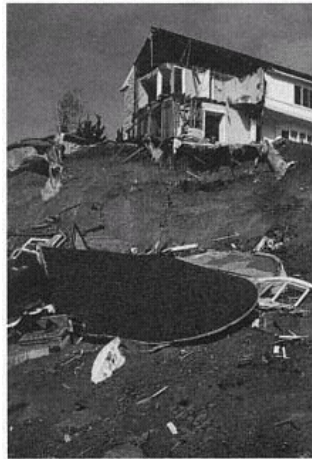
Figure 37 House Pulled Apart by Landslide. Landslides caused a few dramatic losses of single-family homes, but the majority of houses damaged suffered only minor cracking and broken glass. (© J. Scott Smith)
