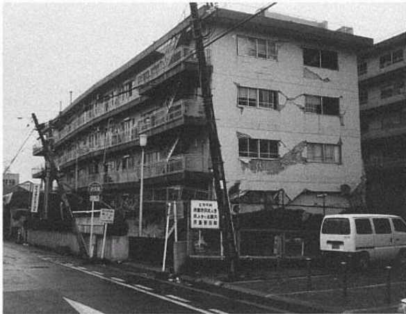
Figure 61 Damage to Multifamily Four-Story Structure. More modern apartments were damaged alongside older wooden structures, which constitute the majority of Kobe's housing stock. (Catherine Bauman)
