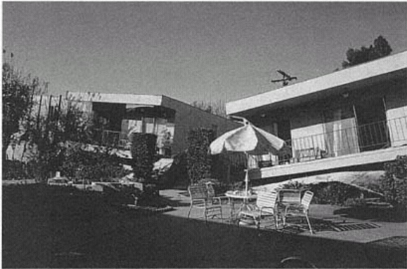
Figure 41 Damaged Garden Apartments. Modern building codes did not prevent significant damage to wood-frame apartments, a result of poor design and construction practices and code deficiencies. (© J. Scott Smith)
