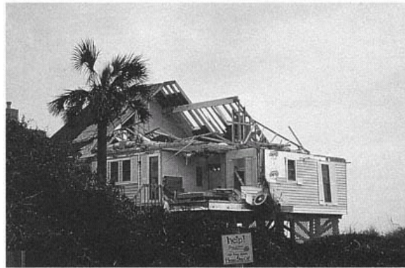
Figure 13 Beach House, Folly Beach. Roofs constructed without hurricane clips were stripped by the high winds. (Peter R. Sparks)
