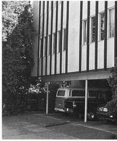
Figure 69 Typical Modern Multifamily Housing, Berkeley. Many apartments were built in the 1960s and 1970s on infill sites throughout the East Bay Area. In order to accommodate parking, there are few structural supports at the lower level. (Mary C. Comerio)
