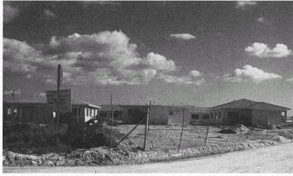
Figure 33 Reconstruction in Homestead. Streets and homes were rebuilt on existing subdivision lots. (Catherine J. Firpo)
