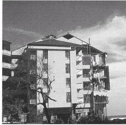
Figure 12 Ocean Club Condominiums, Isle of Palms. Inadequate codes and poor-quality construction contributed to the extensive damage to vacation developments. (Peter R. Sparks)
