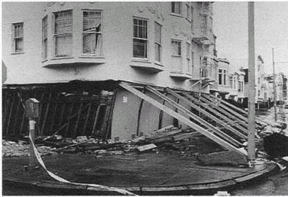
Figure 2 Residential Earthquake Damage, Loma Prieta. Earthquake damage to multifamily structures is often caused by the collapse of a "soft" first story. (California Governor's Office of Emergency Services, Earthquake Program)
