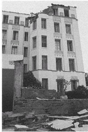
Figure 38 Damaged Historic Unreinforced Masonry Building, Santa Monica. Unreinforced masonry buildings in Santa Monica were heavily damaged. The city had not begun implementation of a retrofit program at the time of the earthquake. (© J. Scott Smith)
