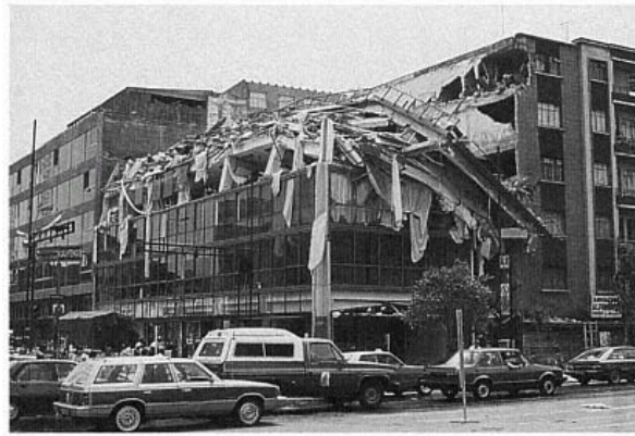
Figure 49 Typical Pancake Collapse of Concrete Building, Mexico City. The columns of mid-rise concrete buildings collapsed, and floors pancaked one upon the other. Soft soils amplified the ground shaking, causing massive failures in a variety of building types. (California Governor's Office of Emergency Services, Earthquake Program)
