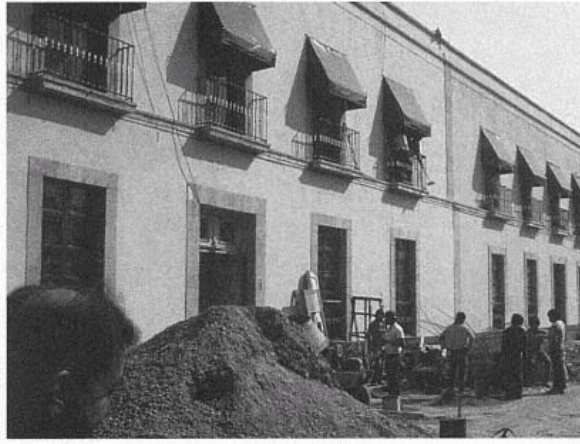
Figure 55 Repaired Masonry Housing Structure. Nearly thirty-eight thousand damaged buildings were repaired at the same time. (Christopher Arnold)
