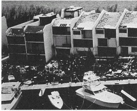
Figure 31 Waterfront Condominiums with Roof and Window Damage. Multifamily structures comprised more than 40 percent of the housing losses in Hurricane Andrew—some were beachfront condominiums, but the majority were apartments for moderate-income service personnel. (National Oceanic and Atmospheric Administration Photo Library)
