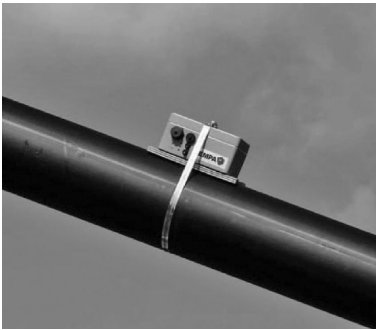
176 Sensor mounted to stay cable. (Source: Used with permission from Reference 14.)
