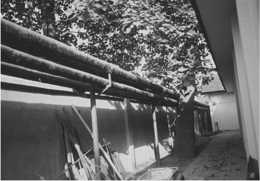
Plate 19 Central heating and hot water pipes leading from a boiler to a building (Beijing)
