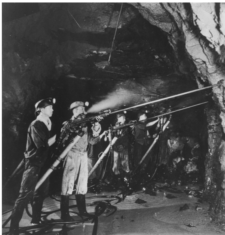
Plate 4 New tunnel construction at Yanzhou CMA (Shandong) (Photo: Courtesy of The Beijing Review )
