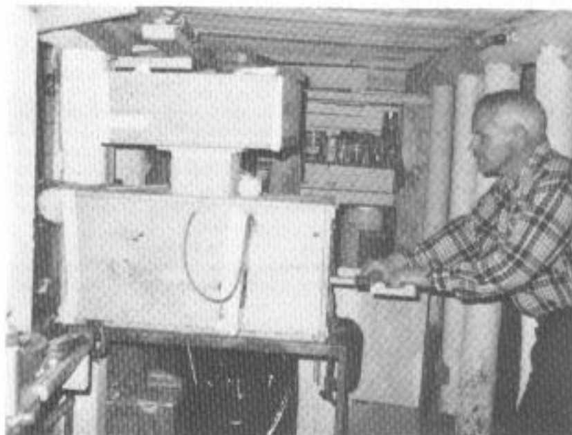
Fig. 3. Pump with Homemade Filter (20 x 20 x 8-inches inside dimensions) connected airtight on top of the pump's 6 x 6-inch air-intake duct.
