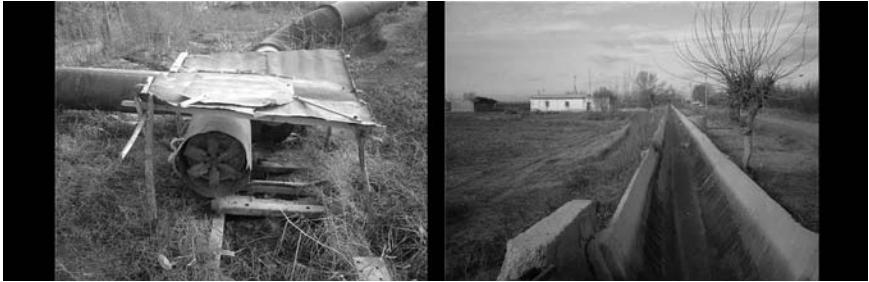
Figure 16.3 Condition of irrigation network in Khorezm, 2003 (Own presentation).
