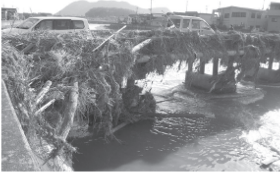
Photo 6. Driftwoods sticking to a bridge after flood in 2004 (Sugihara River, Japan).
