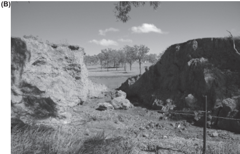
Fig. 11. Dam failures. (A) Malpasset dam, Fréjus, France in September 2004 (Courtesy of Sylvia Briechle); (B) Farm dam failure near Biggenden (QLD, Australia) on 5 March 2013.
