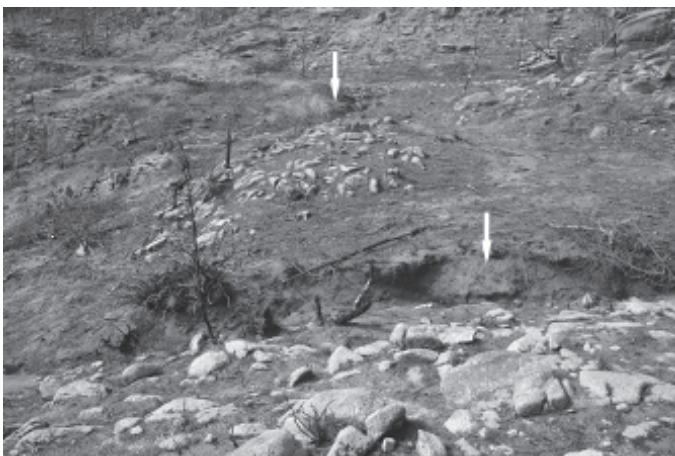
Photo 3. Selected area for the implementation of channel erosion mitigation measures (the arrows indicate the gullies that were intervened).
