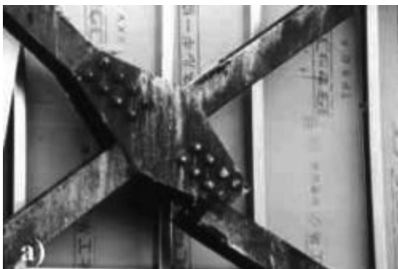
Figure 1.30 Collapse of bolted connections in bracings. (Gioncu, V., Mazzolani, F.M. 2002: Ductility of Seismic Resistant Steel Structures . Spon Press, London; after Fischinger, M. 1997: EASY, Earthquake Engineering Slide Information System. FGG-IKPIP Institute Slovenia.)
