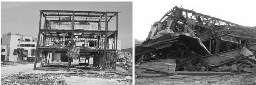
Figure 1.55 Structure damage and collapse due to tsunami. (After Midorikawa M. et al. 2012: Earthquake and tsunami damage on steel buildings caused by the 2011 Tohoku Japan earthquake. International Symposium on Engineering Lessons Learned from the 2011 Great East Japan Earthquake , Tokyo, March 1–4, 1061–1076.)
