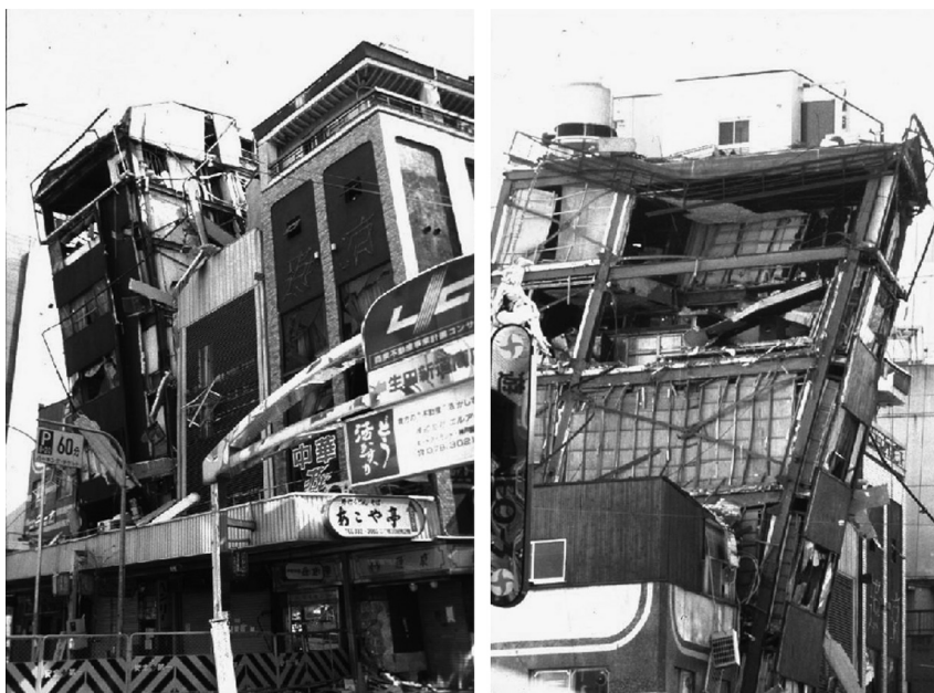
Figure 1.31 Damage of a steel structure. (Gioncu, V., Mazzolani, F.M. 2002: Ductility of Seismic Resistant Steel Structures . Spon Press, London; after Fischinger, M. 1997: EASY, Earthquake Engineering Slide Information System. FGG-IKPIP Institute Slovenia.)
