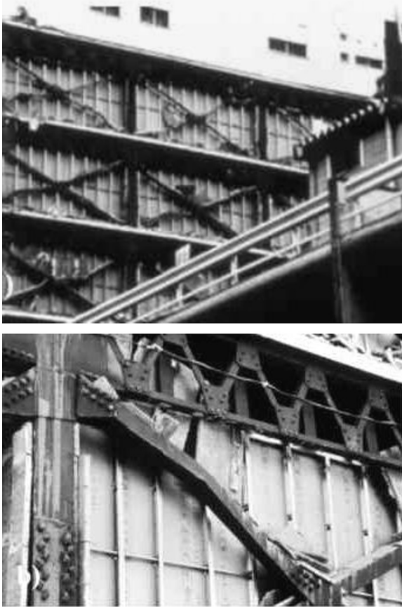
Figure 1.29 Buckling of bracings. (Gioncu, V., Mazzolani, F.M. 2002: Ductility of Seismic Resistant Steel Structures . Spon Press, London; after Fischinger, M. 1997: EASY, Earthquake Engineering Slide Information System. FGG-IKPIP Institute Slovenia.)
