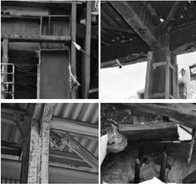
Figure 1.54 Damage or fractures of connections, braces, and anchor bolts due to ground motions. (After Midorikawa M. et al. 2012: Earthquake and tsunami damage on steel buildings caused by the 2011 Tohoku Japan earthquake. International Symposium on Engineering Lessons Learned from the 2011 Great East Japan Earthquake , Tokyo, March 1–4, 1061–1076.)
