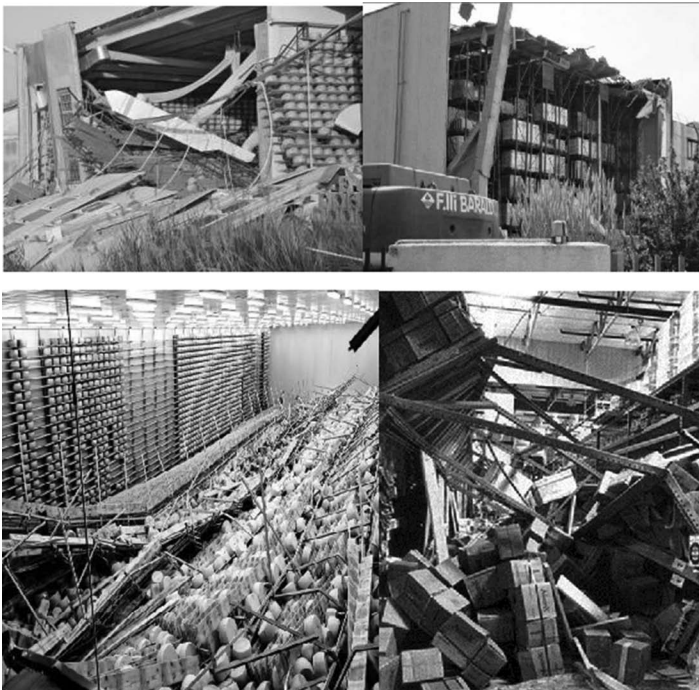
Figure 1.68 The collapse of industrial shelves during the Emilia earthquake. (Faggiano, B. et al. 2012: Steel buildings within the Emilia earthquake (in Italian). Progettazione Sismica , n.3, IUSS Press, ISSN 1973–7432.)
