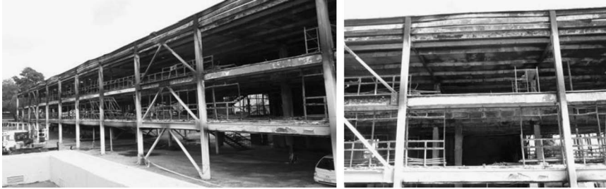
Figure 6.11 The steel building of the University of Chile damaged by fire after an earthquake. (Photo by Mazzolani.)
