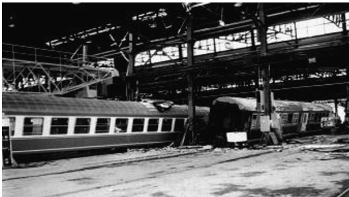
Figure 1.43 Damaged steel building of the railcar factory. (After Erdik, M. 2000: Report on 1999 Kocaeli (Turkey) Earthquake. Bogazici University Report 2000.)
