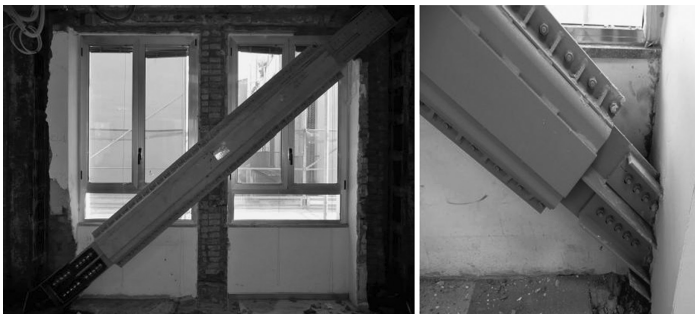
Figure 4.33 The BRB brace in the Deutsche Bank building in Naples and the connection details.
