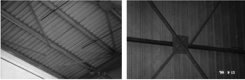
Figure 1.62 Bracing fractures during the 1999 Athens earthquake. (Altay, G. 2005: Post-earthquake damage assessment in the Mediterranean regions. Earthquake protection of historical buildings by reversible mixed technologies, PROHITECH, WP 2.)
