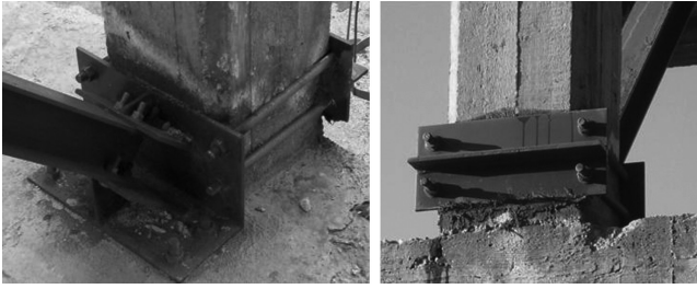
Figure 4.10 Diagonal brace-to-RC end connection. (Della Corte, G., Mazzolani, F.M. 2006: In Proceedings of the 2nd FIB Congress , Naples, Italy, 5–8 June.)
