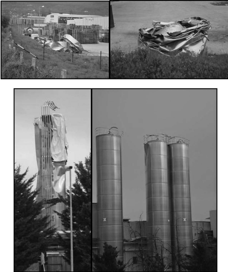
Figure 1.64 Local and global failure of silos.
