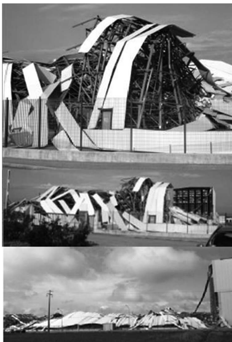
Figure 1.66 The collapse of an industrial building during the Emilia earthquake. (Faggiano, B. et al. 2012: Steel buildings within the Emilia earthquake. (in Italian). Progettazione Sismica , n.3, IUSS Press, ISSN 1973–7432.)
