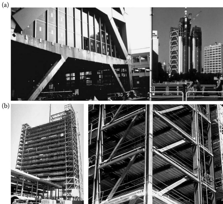
Figure 4.3 (a) Century Tower, Tokyo (1991); (b) multistoried building in San Diego (California, USA).
