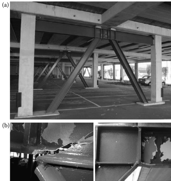
Figure 1.51 Parking garage: (a) eccentrically braced system; (b) damage of the link beam in the welding zone and yielding in the web. (Clifton Ch. et al. 2011: Bulletin of the New Zealand Society for Earthquake Engineering , 44(4):297–318.)
