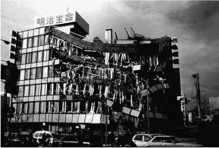
Figure 1.32 Partial collapse of a building corner. (Courtesy of Fischinger, M. 1997.)
