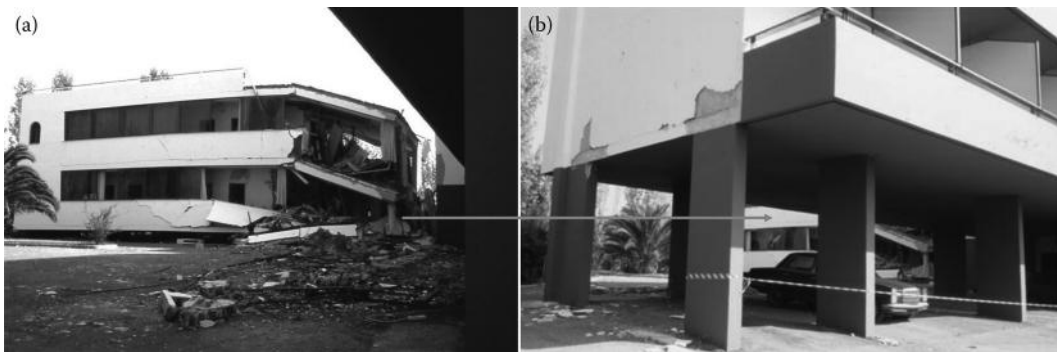
Figure 2.10 (a) Collapse of open ground storey building; (b) collapsed building shown at the background; similar building at the foreground is still standing with large ground storey drift.
