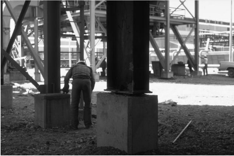
Figure 2.31 Earthquake-induced foundation settlement (Michoacán Guerrero earthquake, 1985).
