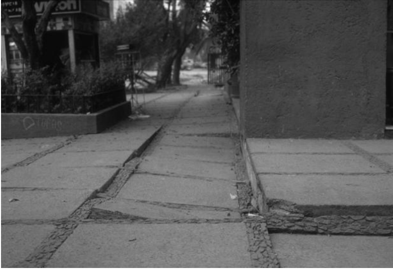
Figure 2.33 Settlement of a pipeline trench adjacent to a building (Mexico, 1985).
