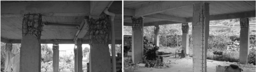
Figure 2.20 Despite complete failure of columns across the ground storey, their residual axial load capacity still supports gravity loads.
