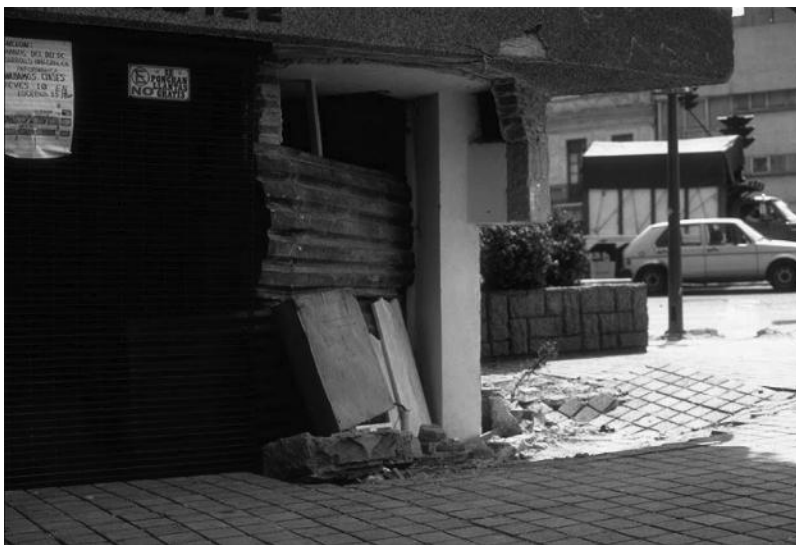
Figure 2.30 Bearing capacity failure in Mexico City (Michoacán Guerrero earthquake, 1985).
