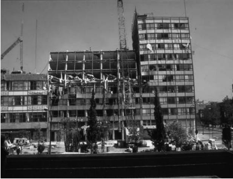
Figure 6.3 Pounding of adjacent buildings in Mexico City due to soil–structure interaction.
