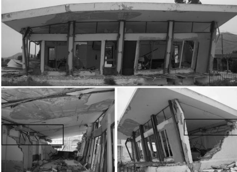
Figure 2.17 Shear failure of short columns on stiff side (inside rectangle) causes collapse of flexible side as well.
