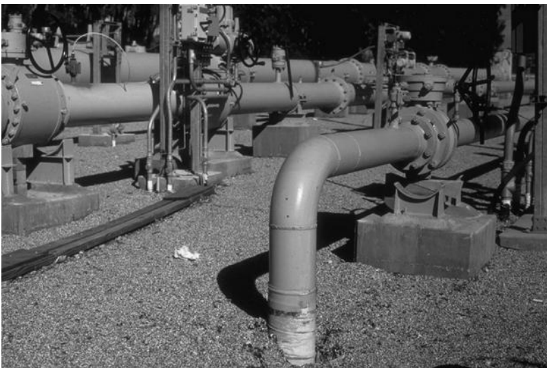
Figure 2.32 Settlement of a poorly compacted backfill (Moss Landing, Loma Prieta earthquake, 1989).
