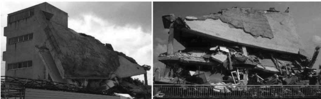
Figure 2.16 Collapse of flexible sides in torsionally imbalanced building with stiffness concentrated near one corner.
