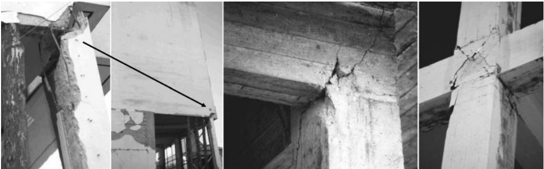
Figure 2.21 Shear failure of beam–column joints.
