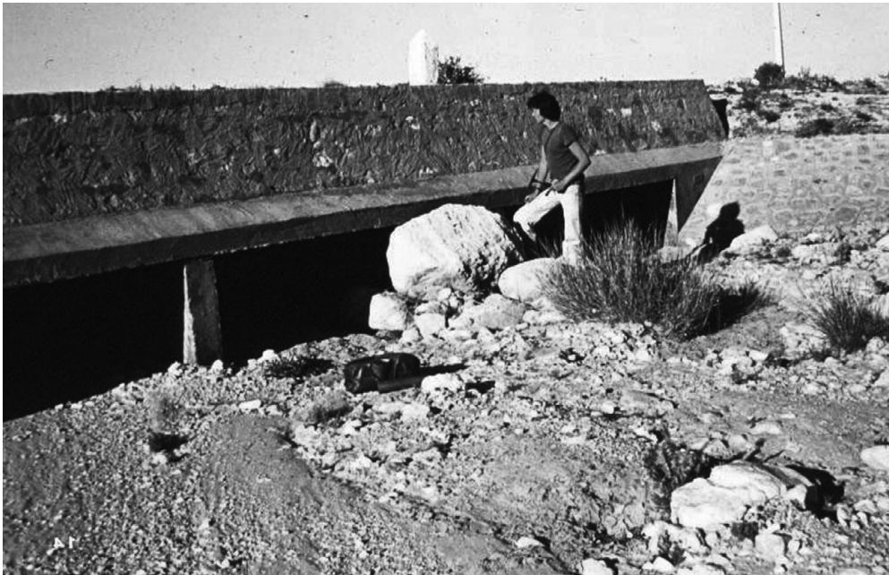
Figure 6.12 A road bridge in southern Tunisia that has been partially blocked by a large boulder brought down in a flood. (ASG)
