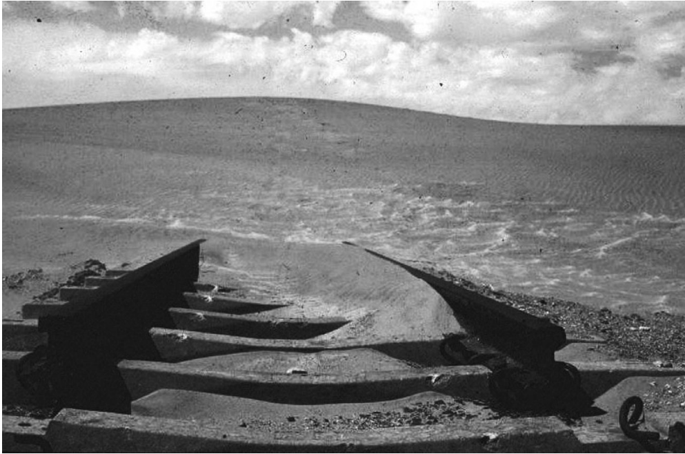
Figure 6.2 The main railway line between Walvis Bay and Swakopmund in Namibia had to be realigned because of sand encroachment. (ASG)
