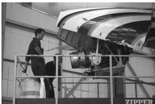
1.5 Maintenance staff working at height considering the alignment of the APU prior to fit
