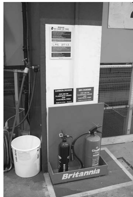
1.9 Typical aircraft hangar fire point
