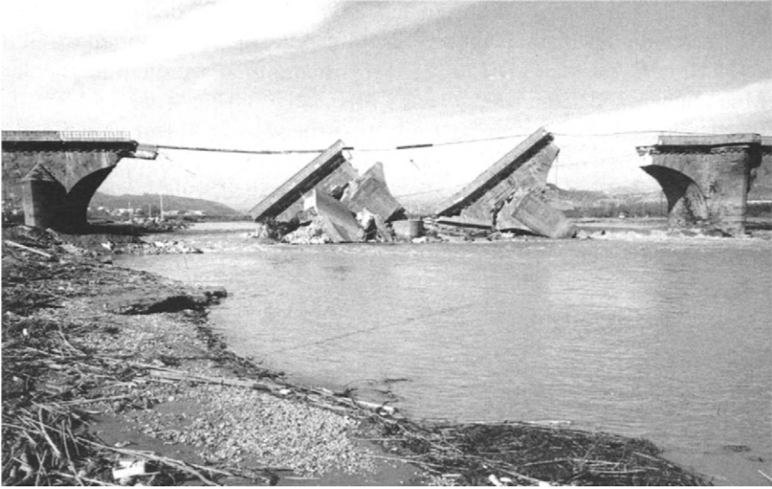
Figure 7. The Carlos III bridge (18th century) in the Llobregat River, Spain, after its collapse during a flood in 1971. Lack of sediment feeding from upstream reaches due to gravel mining was the main cause (source: [151]. The photo is reproduced with kind permission of the Spanish Society of Geomorphology and the Spanish Quaternary Association)
