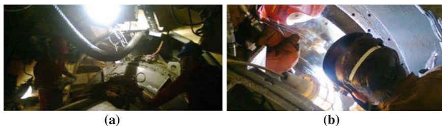
Fig. 9 Presentation of limited space for the shaft recovery. a Shaft prepared for recovery. b Position of the welding operator during recovery
