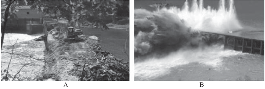
Figure 1-1. Dam removal. (A) Smelt Hill Dam removal in 2002, Presumpscot River, Maine (photo courtesy of Friends of the Presumpscot River); (B) Embrey Dam removal in 2006, the Rappahannock River, Virginia (photo courtesy of the U.S. Dept. of Defense, Integration and Application Network, Image Library, http://ian.umces.edu/imagelibrary ).
