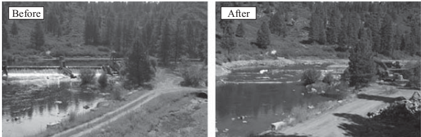
Figure 1-3. Restoration of the Sprague River, Oregon, after the Chiloquim Dam removal. These two photographs were taken by a time-lapse camera that Tim Randle and Mike Neuman of the U.S. Bureau of Reclamation set up during the summer of 2008.
