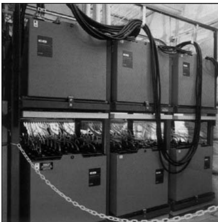
Figure 6 Large lead-acid battery bank
