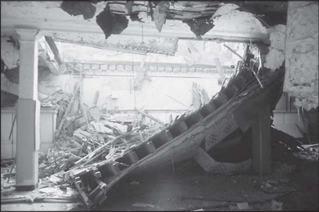
Fig. 6–3. An example of a floor beam collapse
