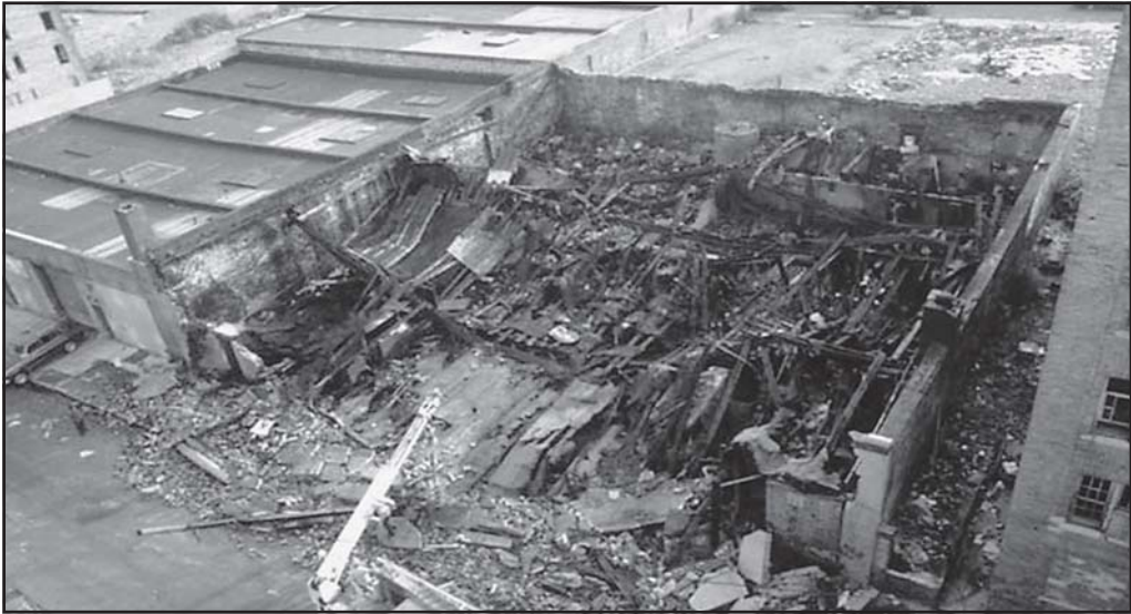
Fig. 8-7. The roof size-up is more accurate than the size-up report given by interior operating forces. When a chief officer receives conflicting reports the chief should rely on the roof report over the interior report.
