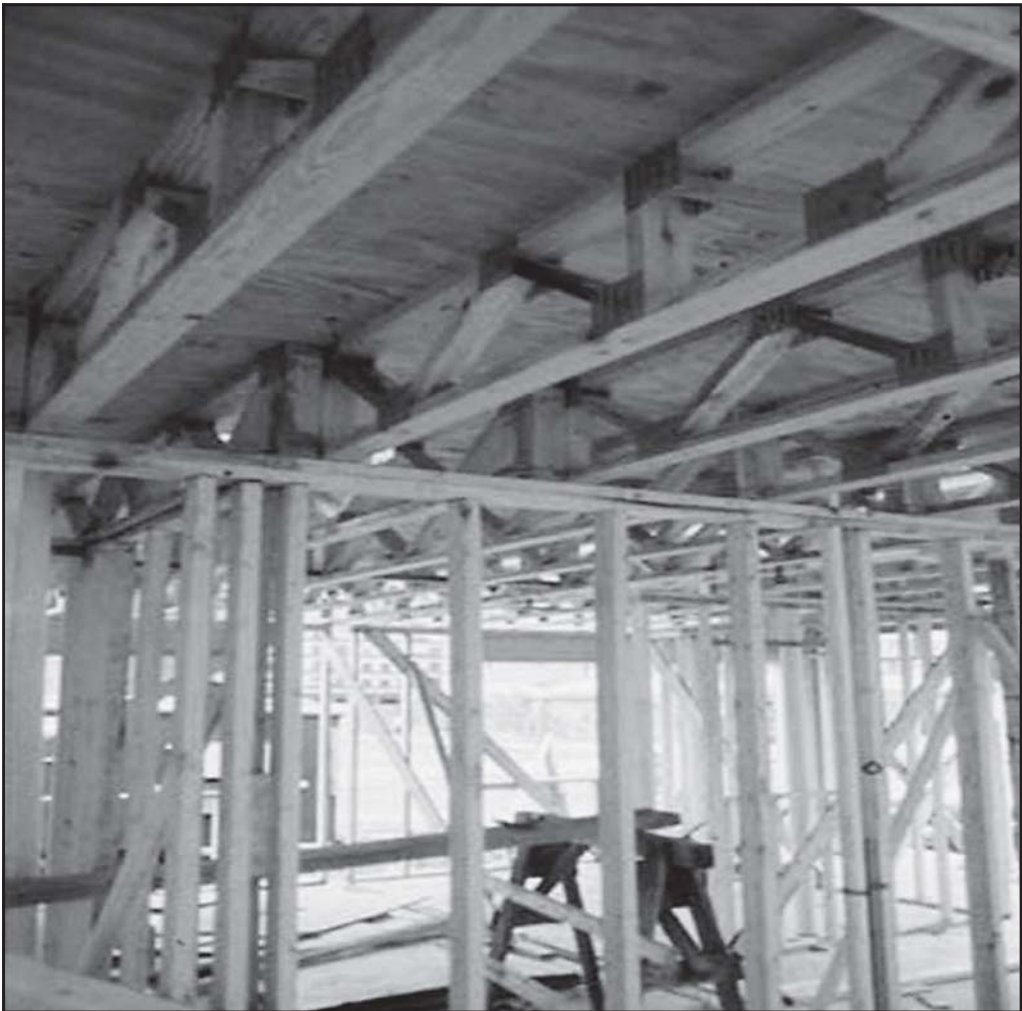
Fig. 11-3. When fire enters the concealed spaces there is a 100% faster fire spread. Flames spread through web members.
