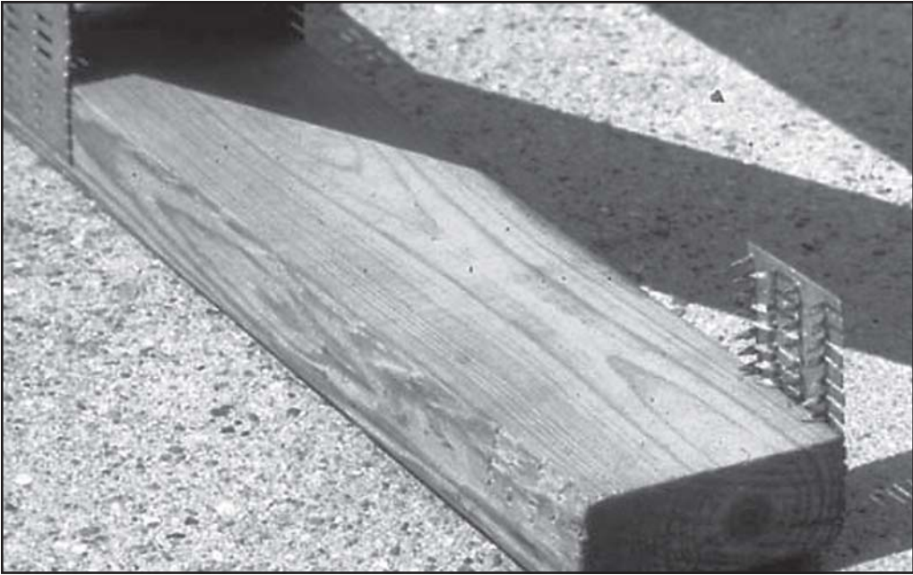
Fig. 11–2. The fire service should seek to outlaw the sheet metal surface fastener.
