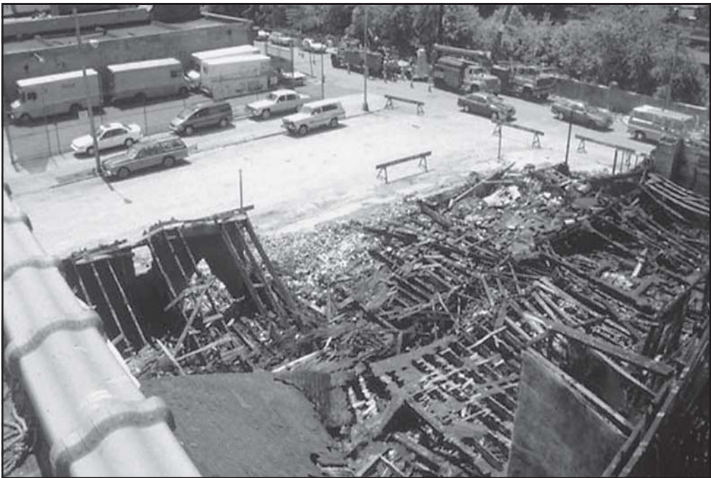
Fig. 8–6. A timber truss roof that caused the collapse of a front wall
