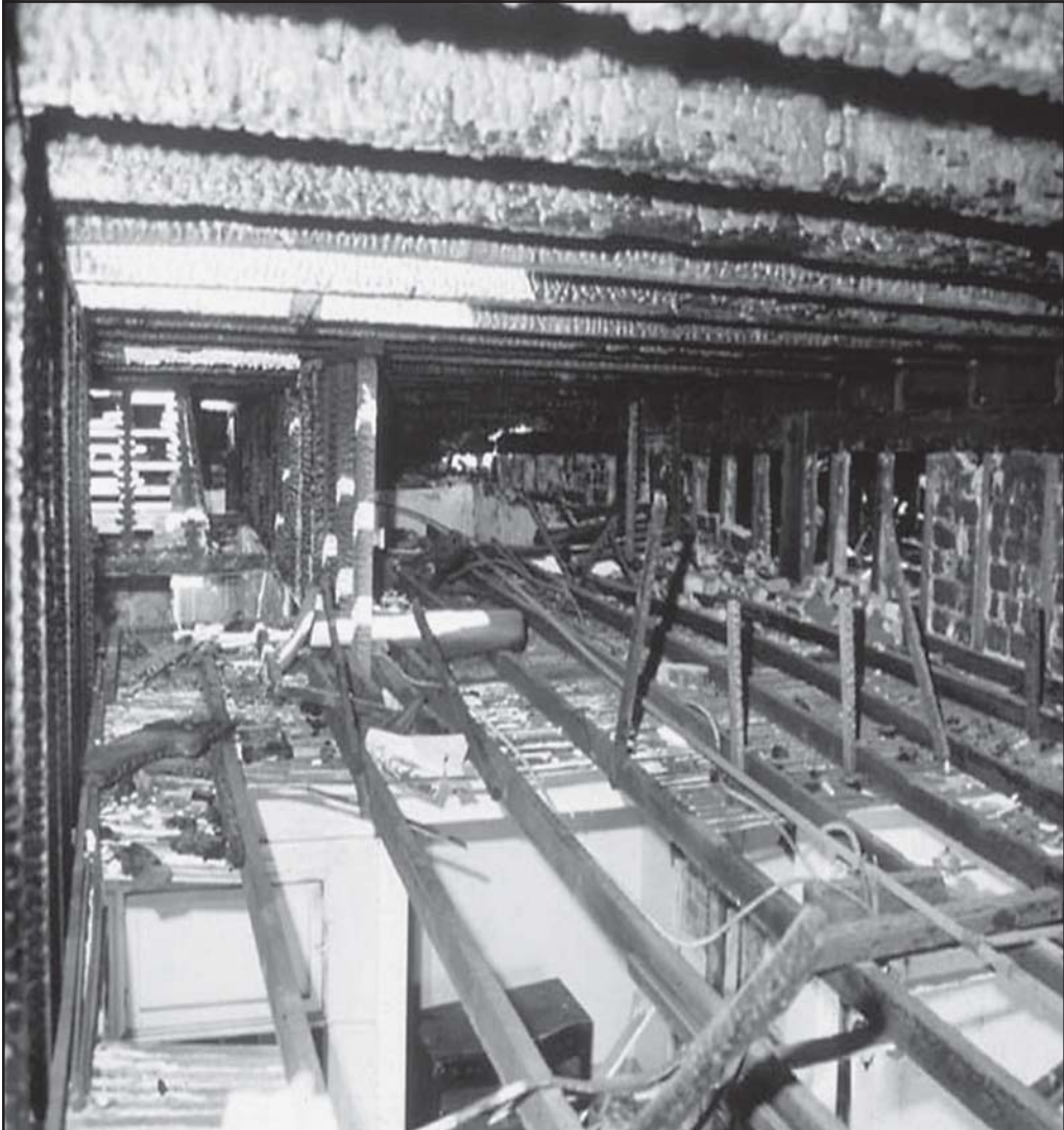
Fig. 15–6. The common roof space is a structural defect in row buildings.
