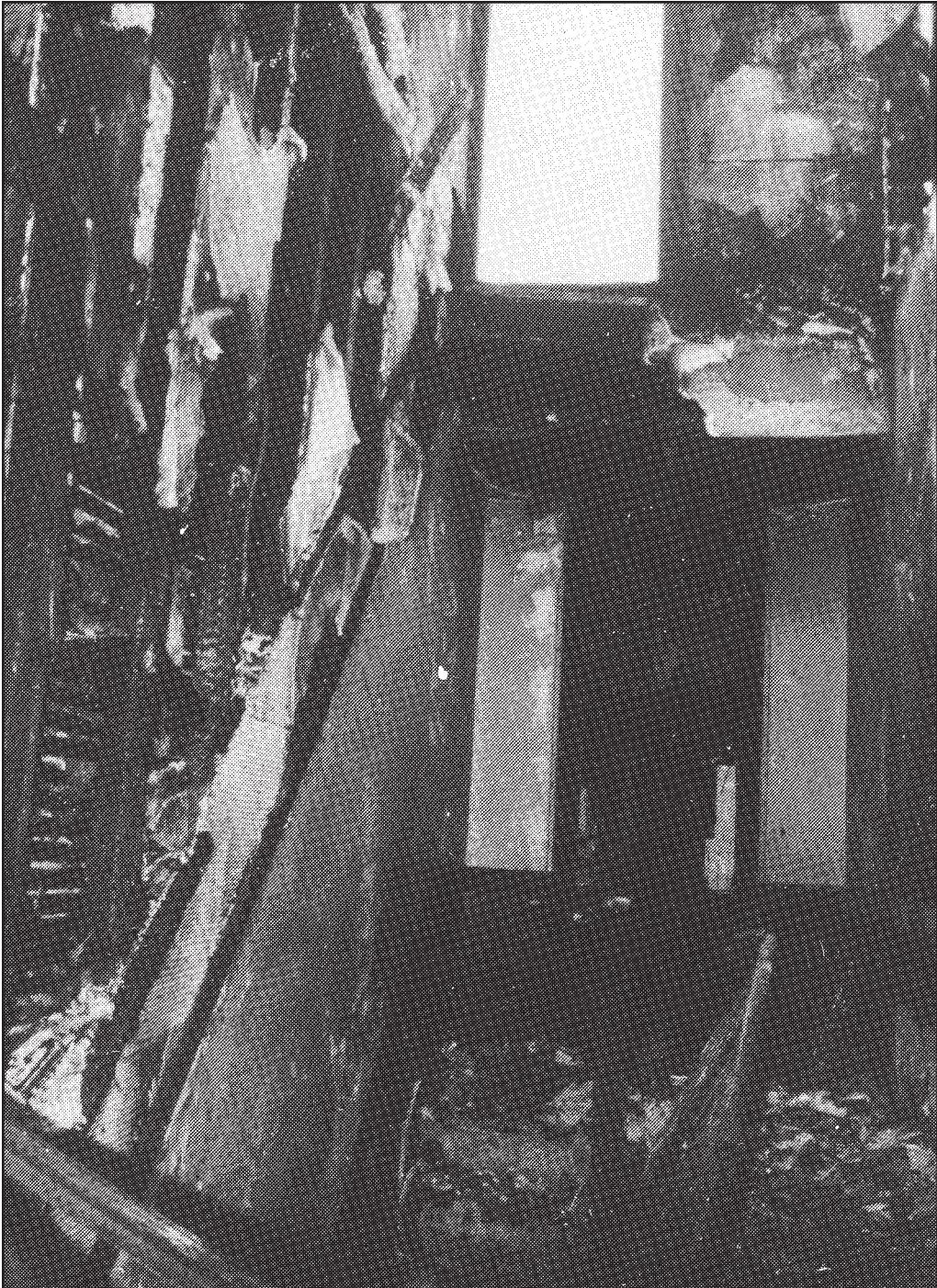
Fig. 13–1. A collapsed wooden straight-run stair
