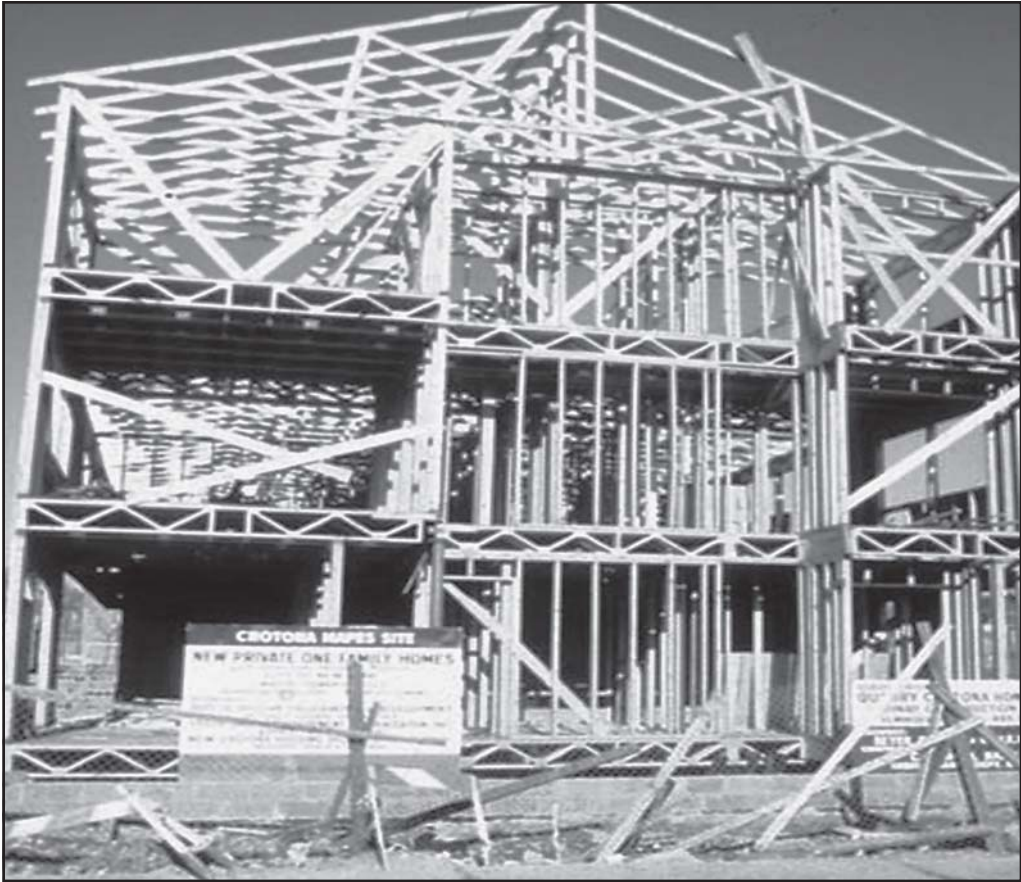
Fig. 11–1. There is nothing larger than 2×4-inch lumber in this lightweight truss roof and floor constructed building.
