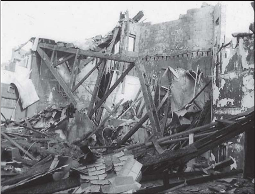
Fig. 8-10. Two Valley Stream, NY, firefighters were killed when this inclined plane timber truss roof collapsed.
