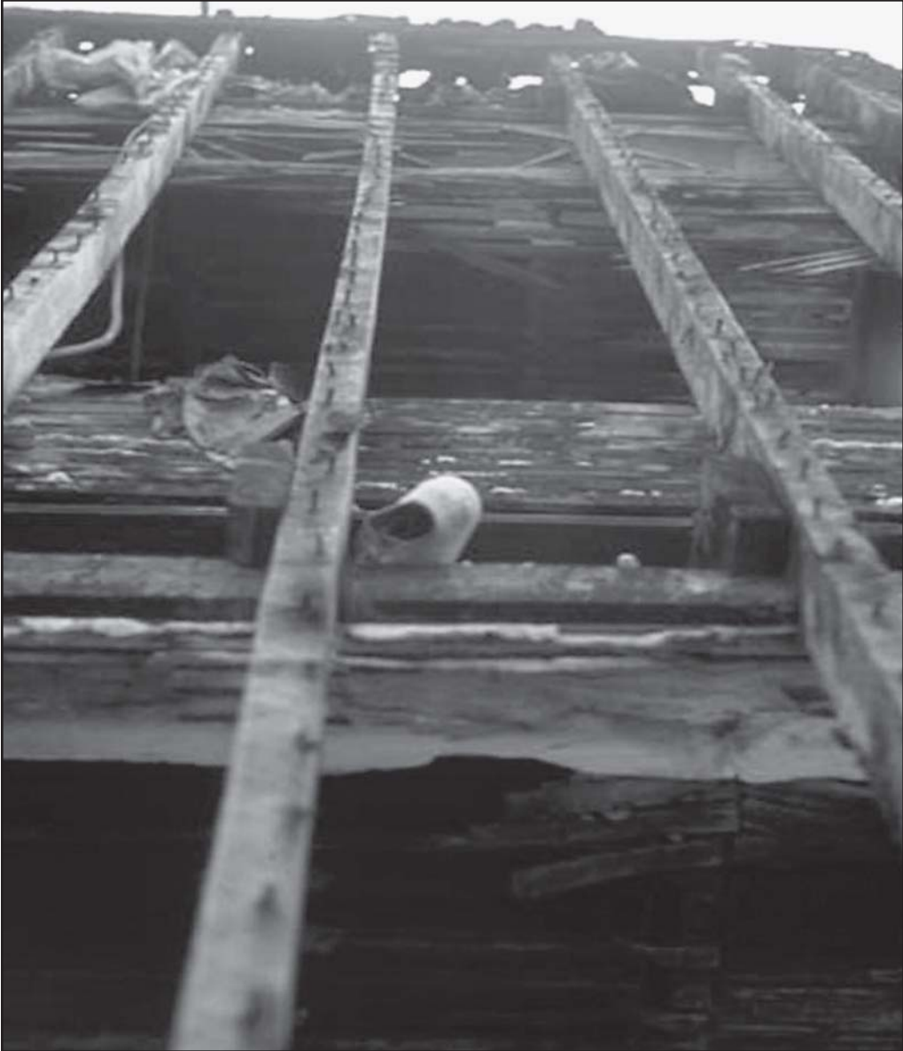
Fig. 2–2. Balloon frame construction has exterior walls that have studs extending continuously from the foundation to the top plate near the attic. This concealed space allows rapid fire spread from the cellar to the attic.
