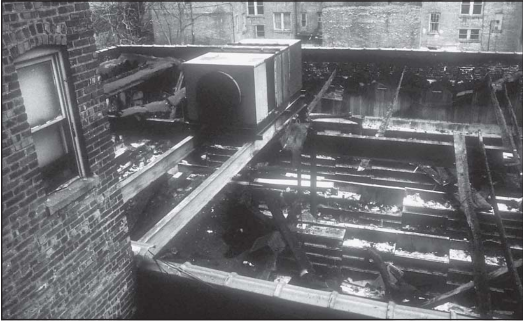
Fig. 9-9. The roof edge around a vent cut may suddenly collapse causing firefighters to lose their balance and fall with a power saw.
