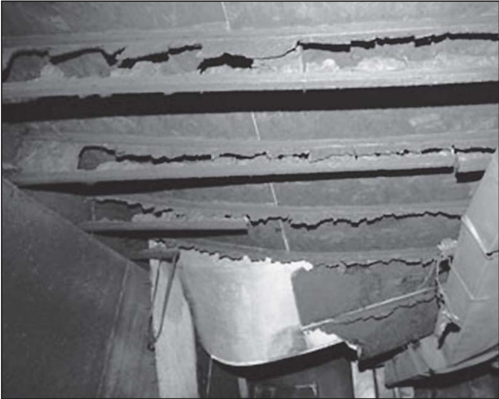
Fig. 23–4. The destruction of wood I-beam floor by fire
