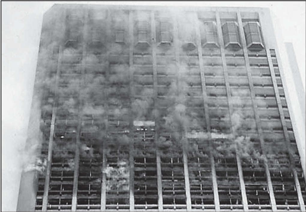
Fig. 3–7. Type I steel skeleton construction. The heat from a fire reaching the underside of a corrugated steel deck is transmitted upward to the concrete floor above. The concrete floor may buckle upward between 6 and 12 inches. The floor may also bow and sag downward as well.
