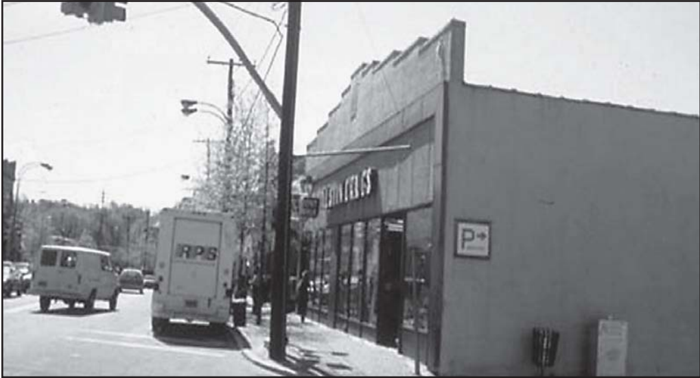
Fig. 5–3. A freestanding parapet wall. A master stream striking the back of this wall could cause it to collapse outward onto the sidewalk.
