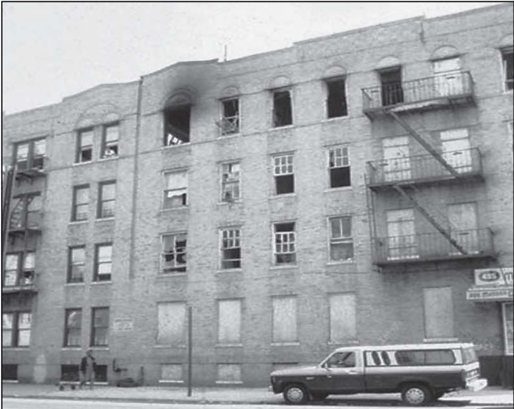
Fig. 12-5. FDNY firefighter Kevin Kane of Ladder 110 died when a suspended ceiling on the top floor of this multiple dwelling collapsed.
