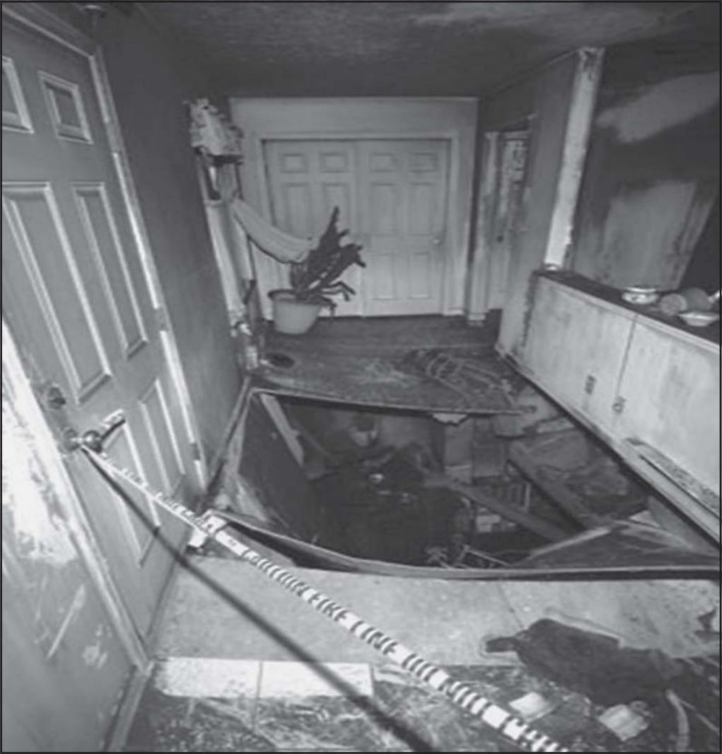
Fig. 23–3. The wood I-beam floor collapsed and killed Chief Steve Smith.
