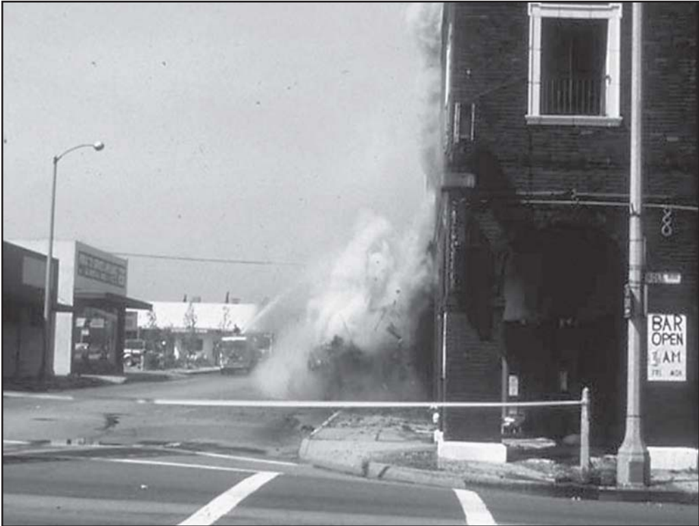
Fig. 4-4. An example of a curtain-fall collapse of a masonry wall
