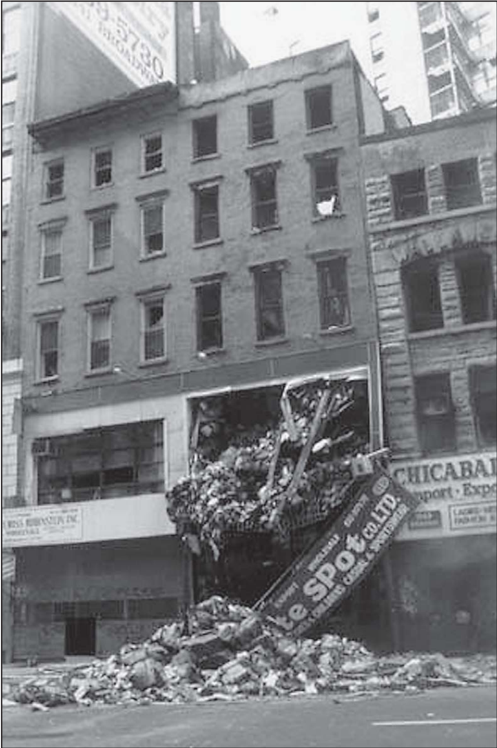
Fig. 6-4. An example of a multilevel floor collapse
