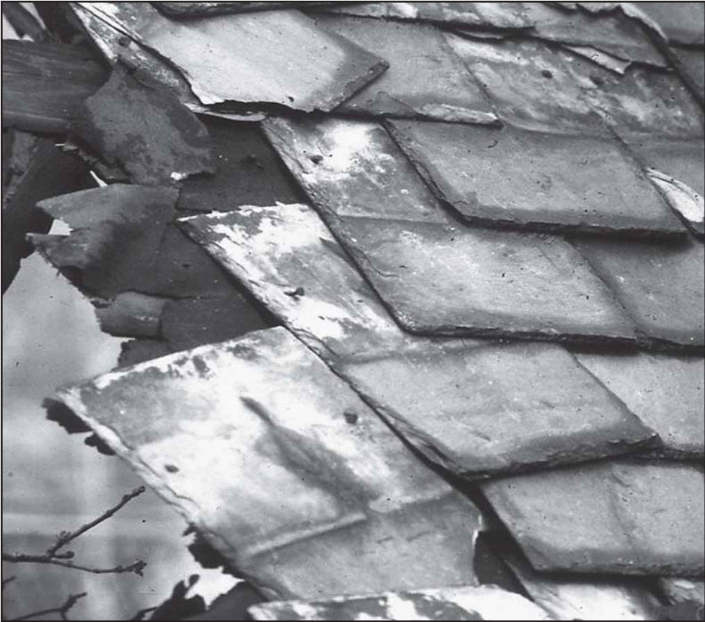
Fig. 7–6. Razor sharp slate shingles falling from a roof can seriously injure a firefighter.
