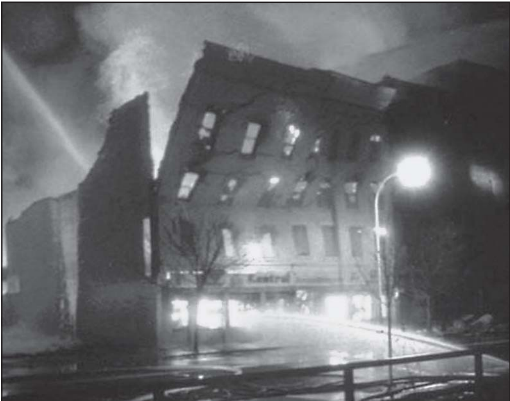
Fig. 4–6. An example of an inward outward wall collapse
