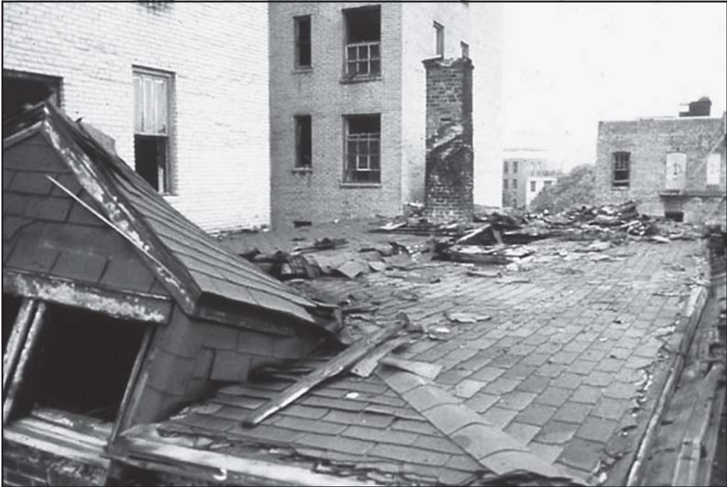
Fig. 7-2. This hip roof collapsed and trapped a firefighter working in the attic space.
