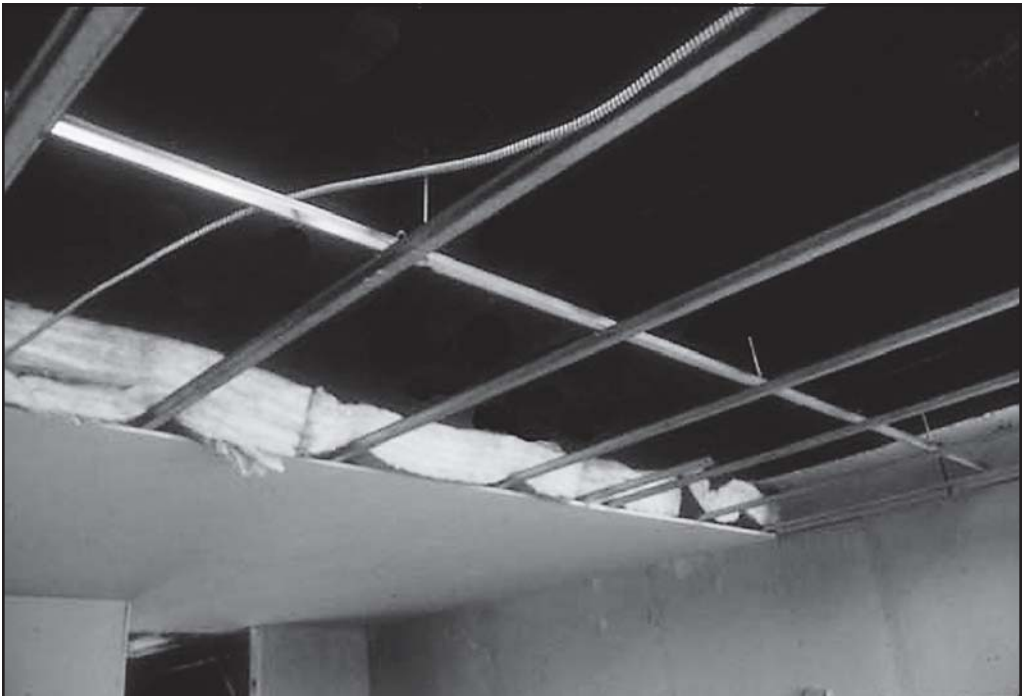
Fig. 12–4. The grid work and framing can trap a firefighter if the ceiling collapses.
