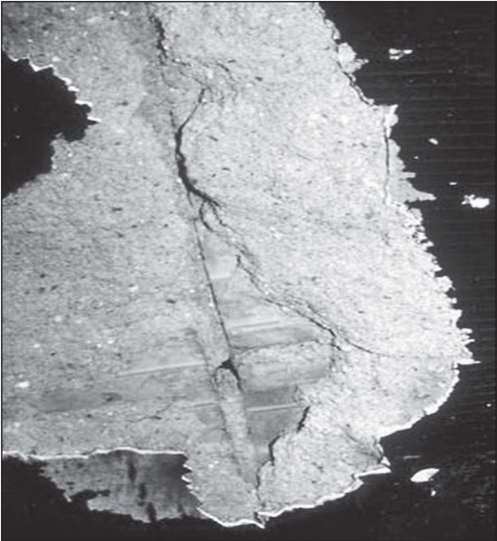
Fig. 16-2. Large chunks of concrete can collapse from a ceiling when heated by a fire.
