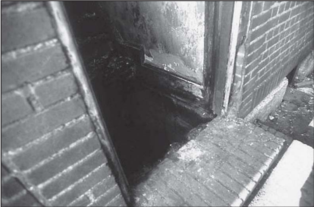
Fig. 6–2. Lieutenant John Clancy died when this floor deck collapsed.
