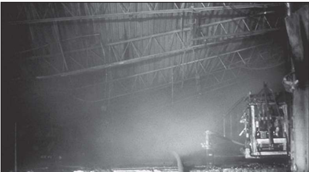
Fig. 10-6. This roof supported by lightweight steel bar joist collapsed during the early stages of the fire.
