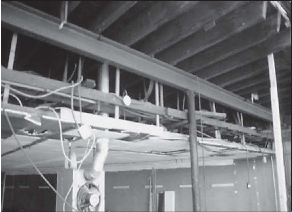
Fig. 12–9. When fire enters a ceiling with two dropped ceilings, fire extinguishment is difficult to nearly impossible.
