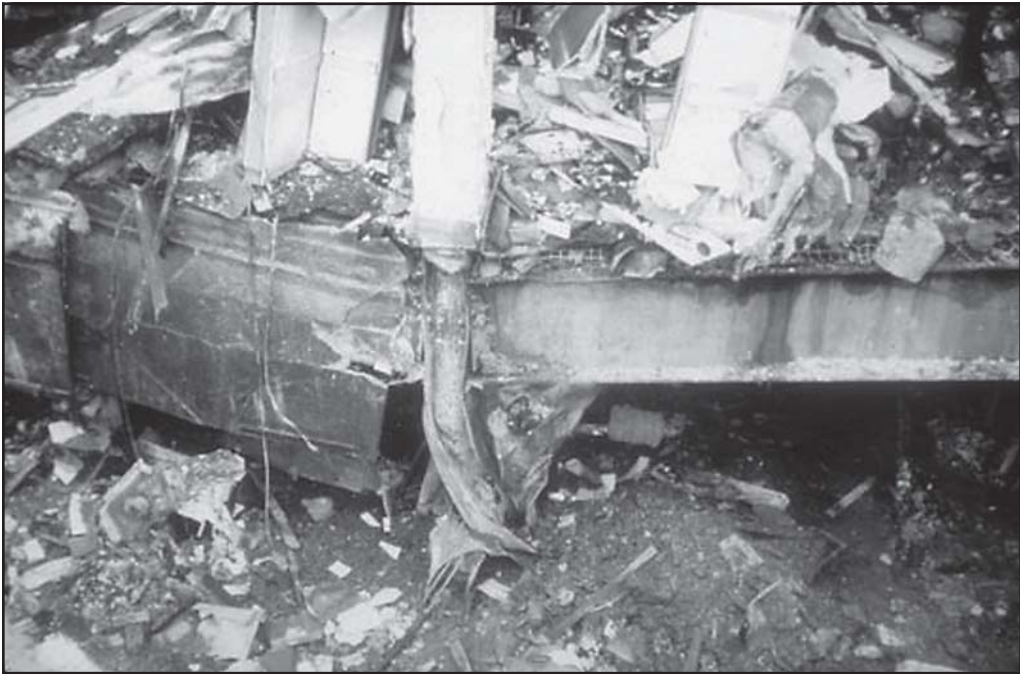
Fig. 1–1. Column failure was the cause of this floor collapse that killed four Brackenridge, PA, firefighters.
