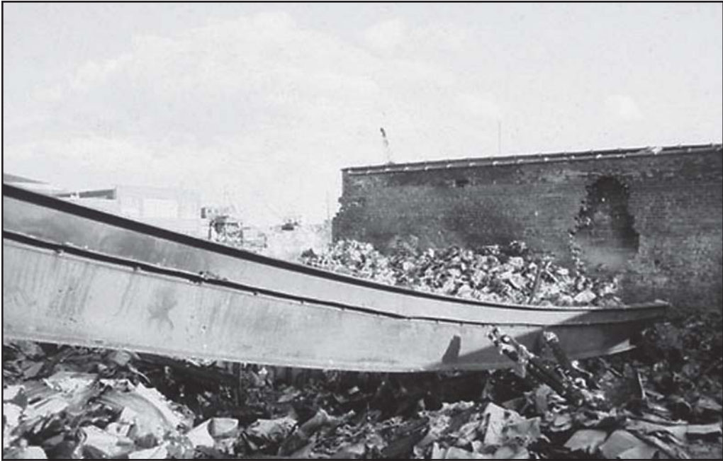
Fig. 10–7. This large steel girder buckled and pulled away from the wall and collapsed during a large area fire in a stationary store.
