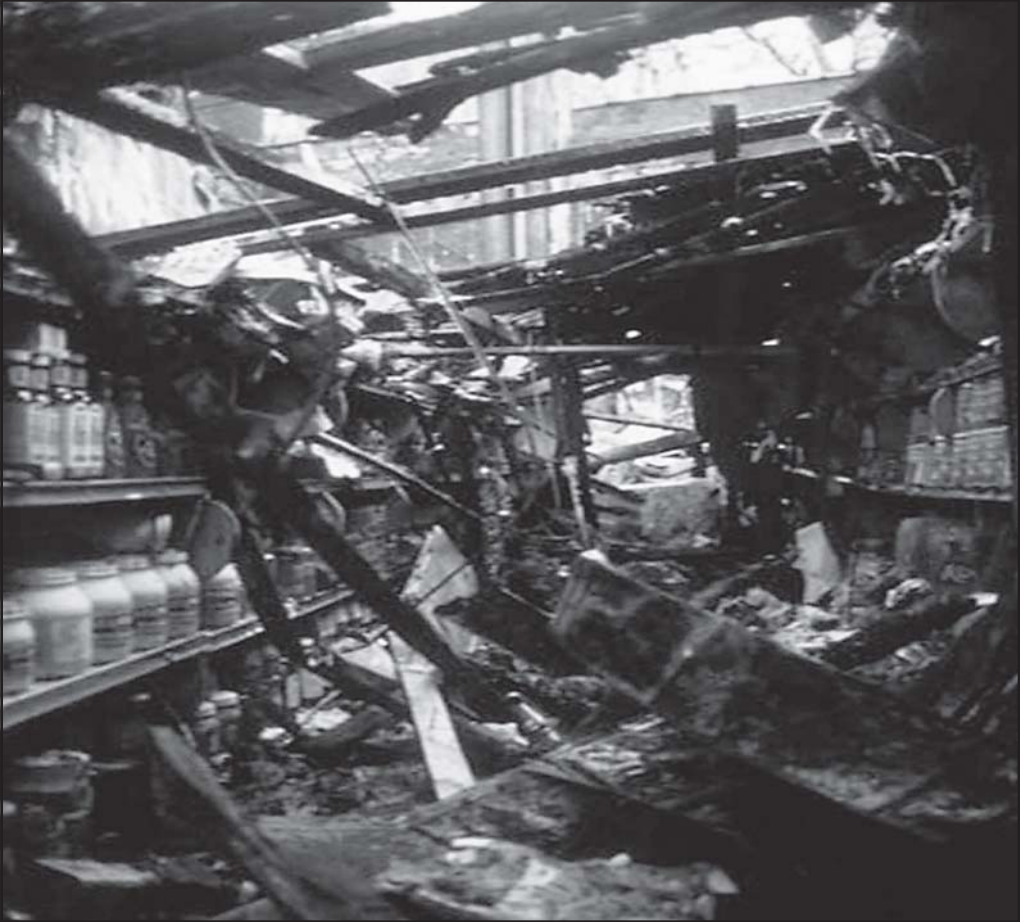
Fig. 12–1. Voids allowing firefighters to escape are created near centers and shelves when a ceiling collapses.
