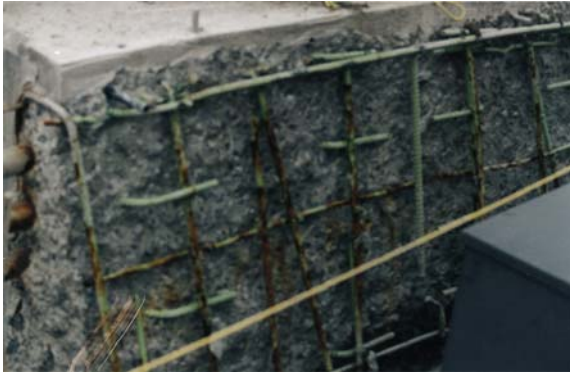
Figure 24.2 Example of the consequence of a very rough handling of epoxy-coated rebars. Courtesy of Daniel Vézina.
