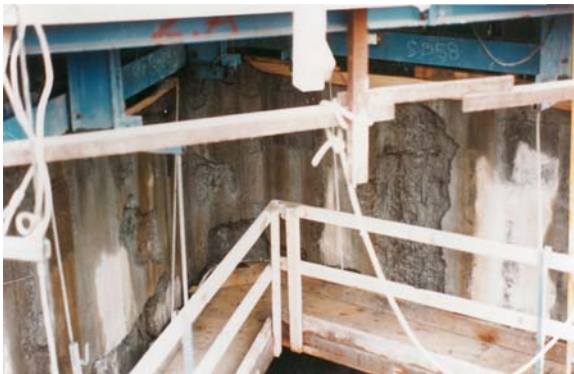
Figure 18.3 External surface of an offshore platform due to the fact that the slipforming occurred too late.
