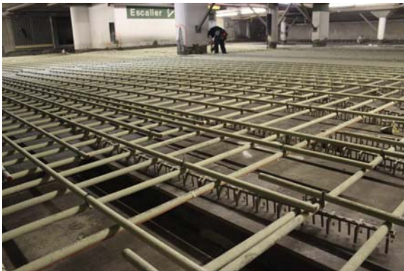
Figure 24.4 The use of glass fiber reinforced bars in an internal parking garage. Courtesy of Brahim Benmokrane.
