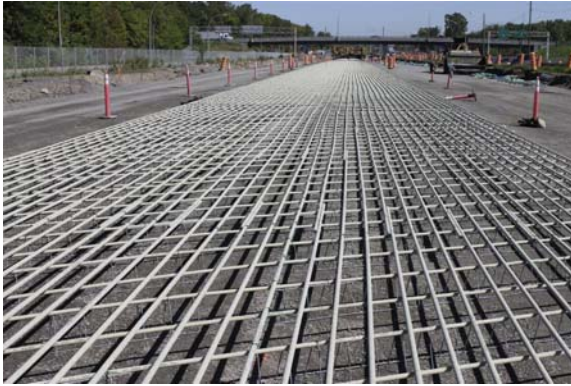
Figure 24.5 The use of glass fiber reinforced bars in a continuously reinforced pavement. Courtesy of Brahim Benmokrane.
