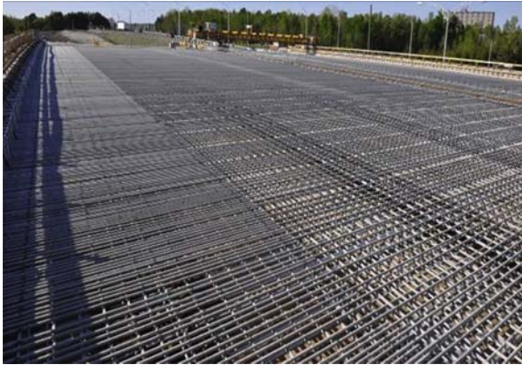
Figure 24.3 The use of glass fiber reinforced bars in a bridge deck. Courtesy of Daniel Vézina and Brahim Benmokrane.
