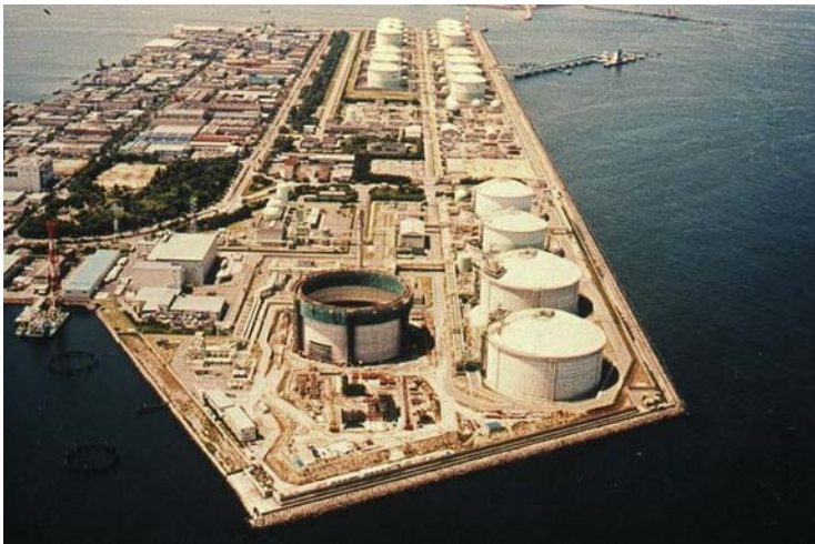
Figure 26.5 Construction of post-tensioned concrete LNG storage tank with a 60 MPa SCC in Senboku Terminal II in Osaka.
