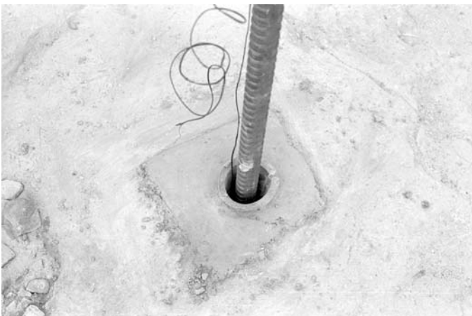
Figure 21.5 The small rectangular base built around each anchor to support the base of the hollow jack used to pull out the anchors. The temperature of each grout was monitored by a thermocouple.
