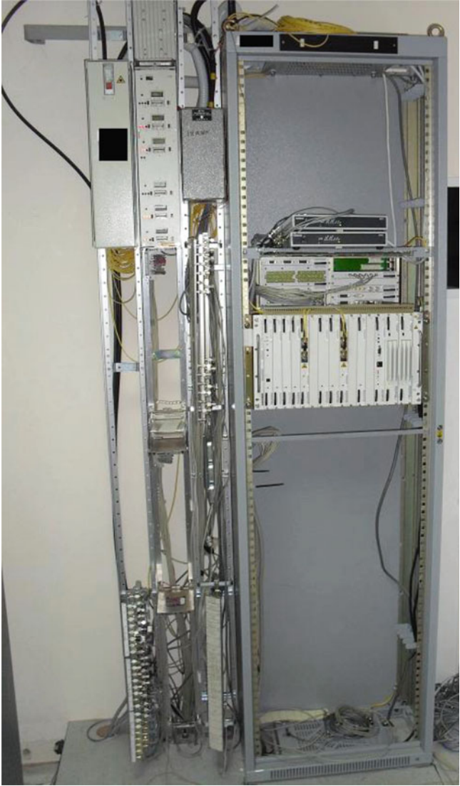
Fig. 3.2 Large size office demarcation point
