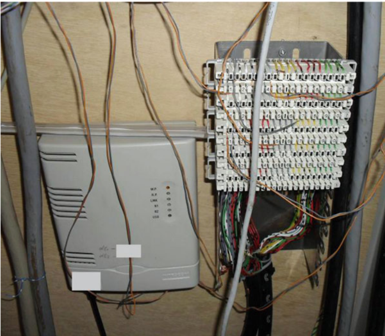
Fig. 3.4 Small office main distribution frame and CPE
