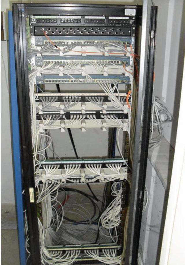
Fig. 3.7 Rack with patch panels
