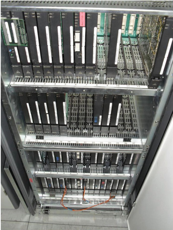
Fig. 1.2 The front side of the PBX
