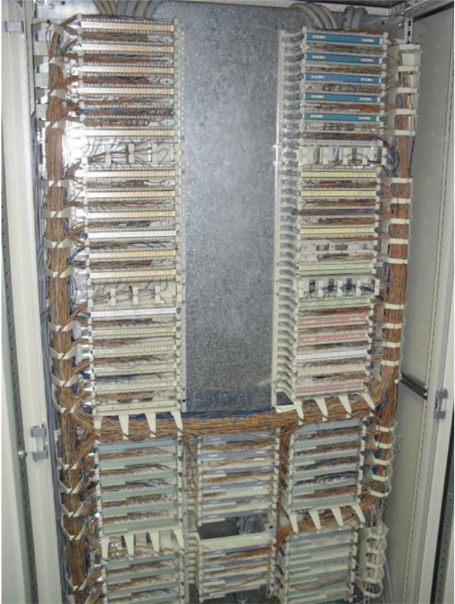
Fig. 3.6 Large company main distribution frame
