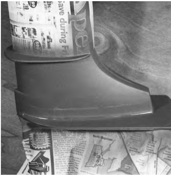
Figure 10-6. The corroded area masked off and ready to spray.
