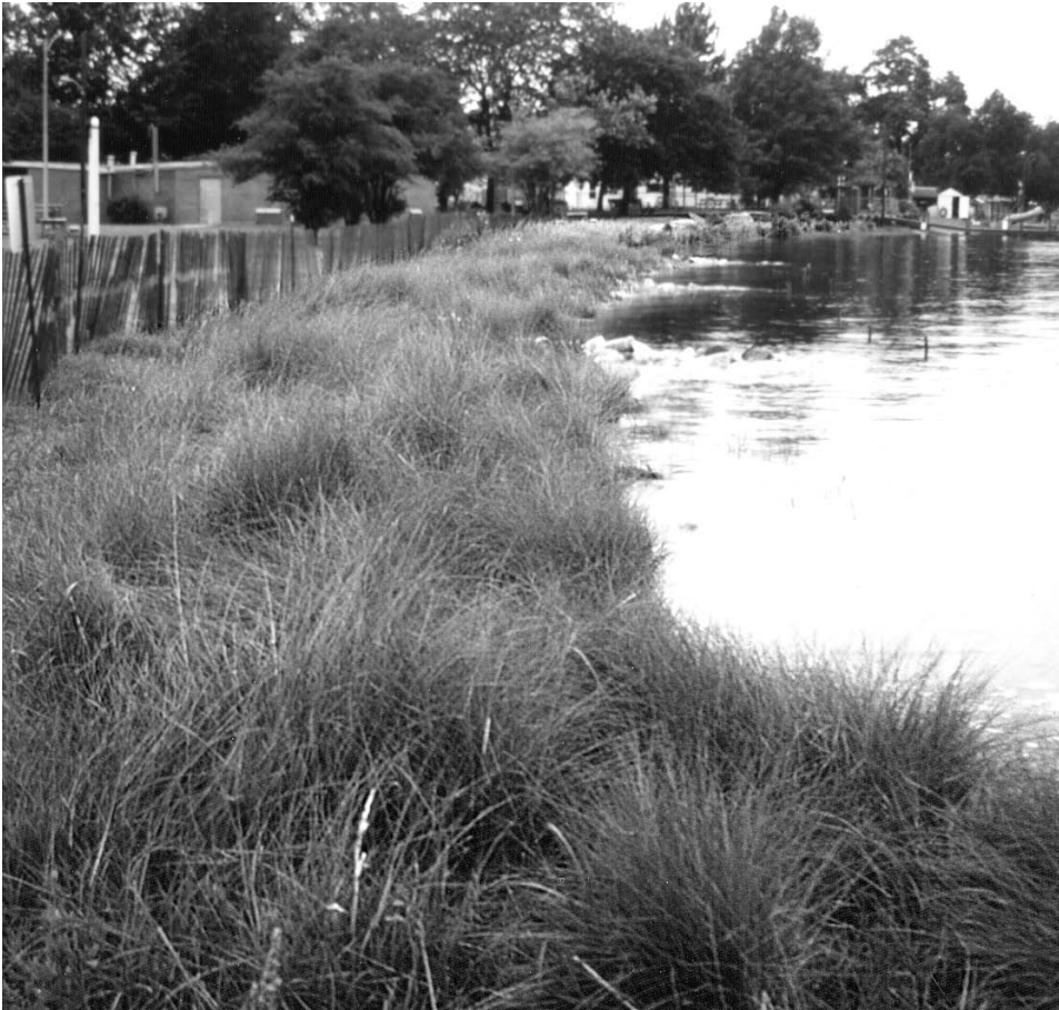
Shoreline enhancement project in Bear Creek, a tributary to the Patapsco River and the Chesapeake Bay. Work included grading eroded banks and planting wetland grasses. Photograph courtesy of Baltimore County, Maryland.
