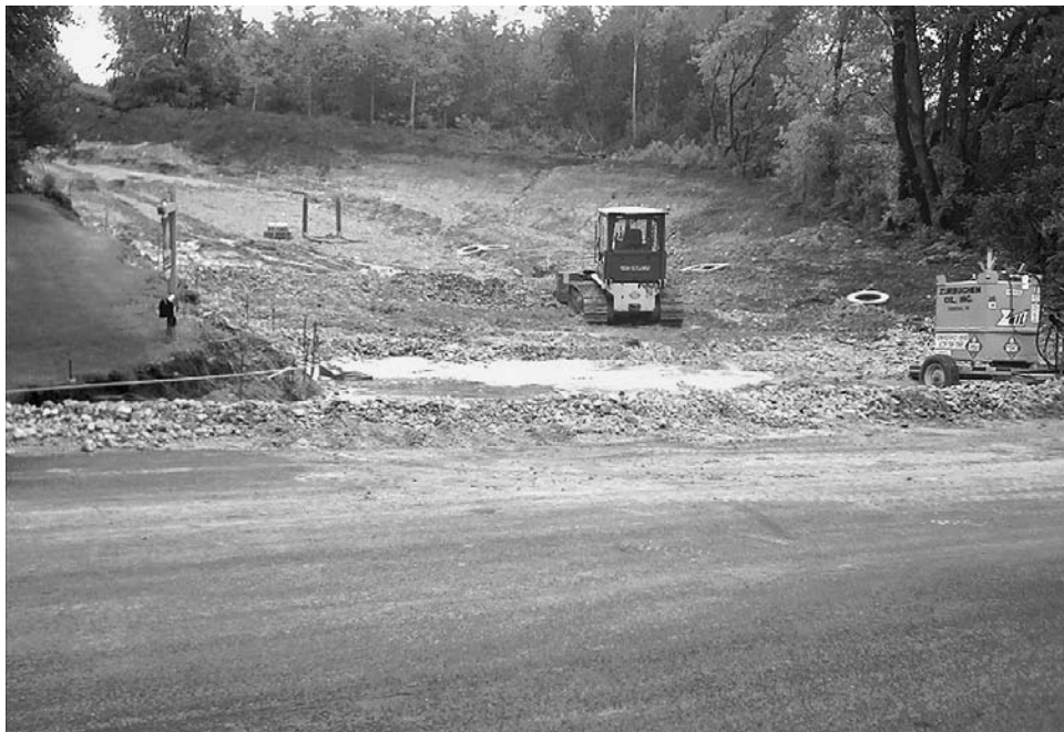
Dane County's new stormwater regulations will help to control urban erosion such as construction site runoff. Photograph courtesy of Dane County.
