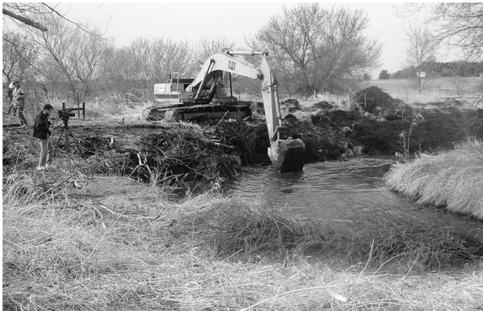
Stream restoration can include narrowing the channel and reshaping the banks. Photograph courtesy of Dane County.
