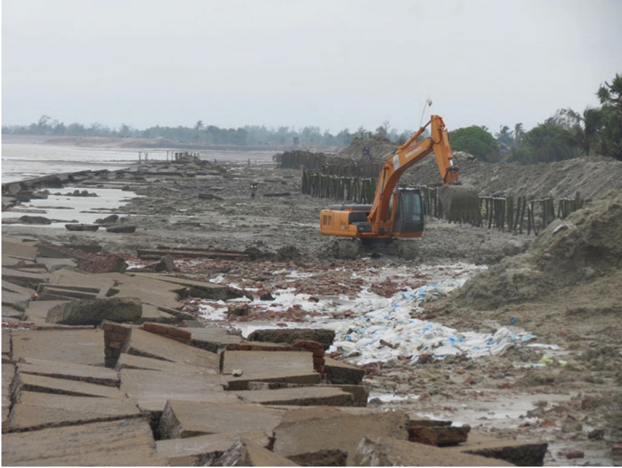
Photo 5.14 Debris of an embankment; concrete, wooden logs, earth, bricks and bamboo, all destroyed by the ravaging perigean spring tide in 2014, August 2014 Baliara, Mousuni, © Aditya Ghosh
