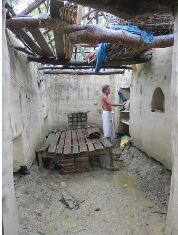
Photo 4.2 House of Shiv Shankar Pal in Baliara, Mousuni and the damage it suffered. Pal was among almost over 5000 households that suffered similar damages. July 2014 © Aditya Ghosh
